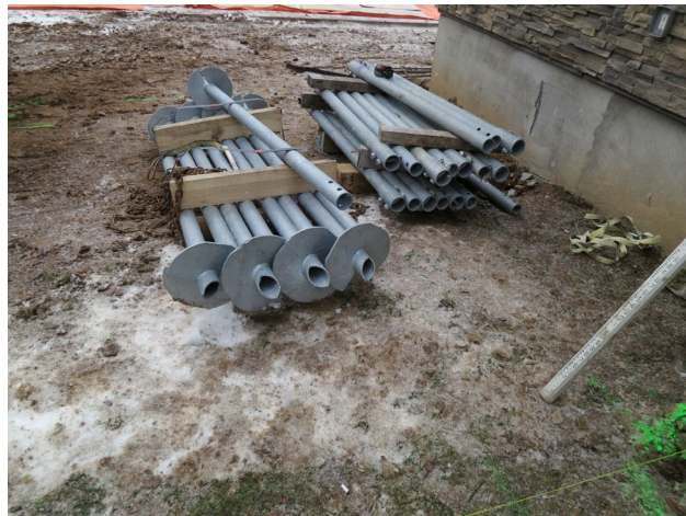
36 - Dec.22nd. A total of 11 helical piles (screw piles) were necessary on the south side of the club house. Based on the site specific ground conditions, each pile ended up approximately 21 ft. long.
