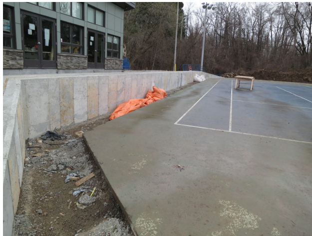
90 - April 14th. Front view of the deck wall and the exposed side of the wall will be cleaned up.
