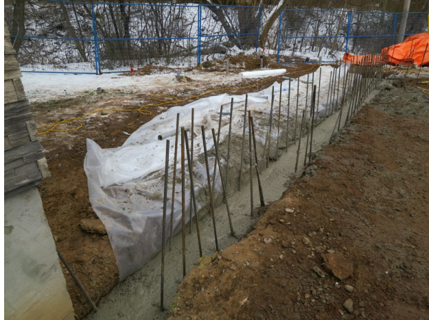
37 - Dec. 23rd. This just poured concrete foundation sits on helical piles and is for the backwall of the concrete deck, adjacent to and south of the clubhouse.
