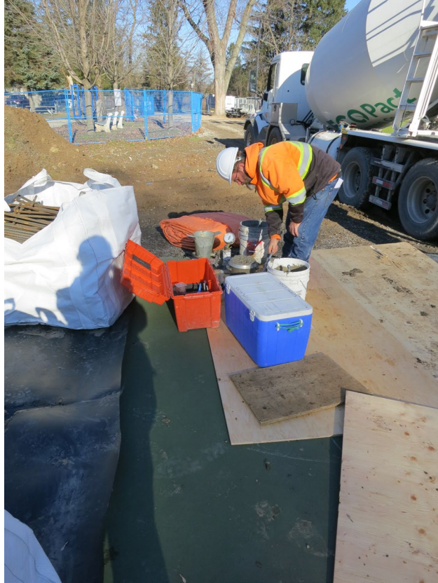
27 - Taking concrete test cylinders for compression tests. Air entrainment tests were carried out on the site.
