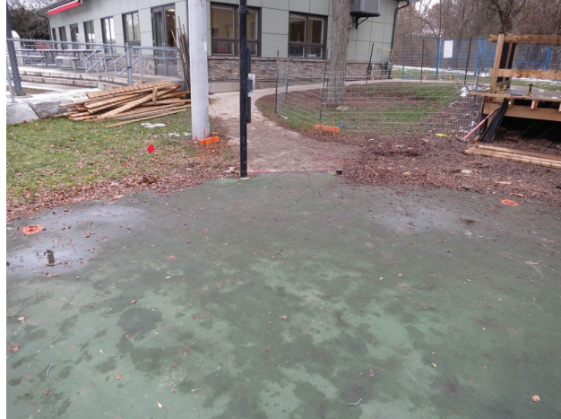
10 - Orange markers indicating building envelope. Location where the Dome fabric meets the grade beam.
