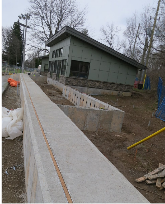
92 - April 14th. When the concrete is poured a 2x4 is inserted in the extrusion channel in which the dome is attached to. The back portion of the deck, beside the clubhouse, will be made out of wood. The posts will sit on the visible tubes (helical piles).
