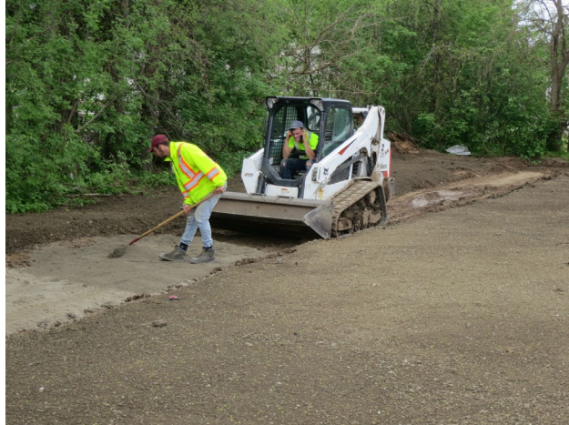
117 - May 17th. Construction of the path on the south side of the courts.
