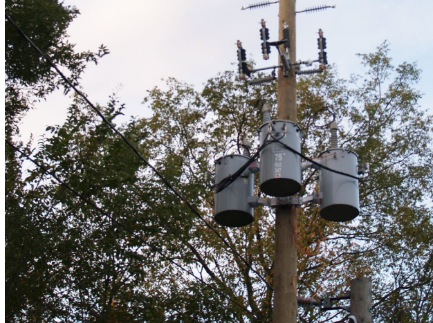
2 - November 30th. Installation of three phase transformer by Alectra utilities for the supply of extra power to the Dome's electrical equipment.
