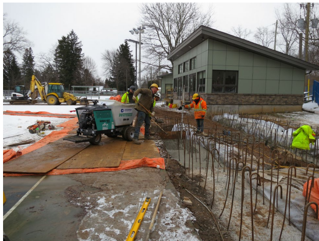
38 - Dec. 23rd. The pouring of concrete for the continuation of the foundation for the deck wall. The Dome fabric will be attached to the top of the wall . The deck will be a concrete one (fire regulation).
