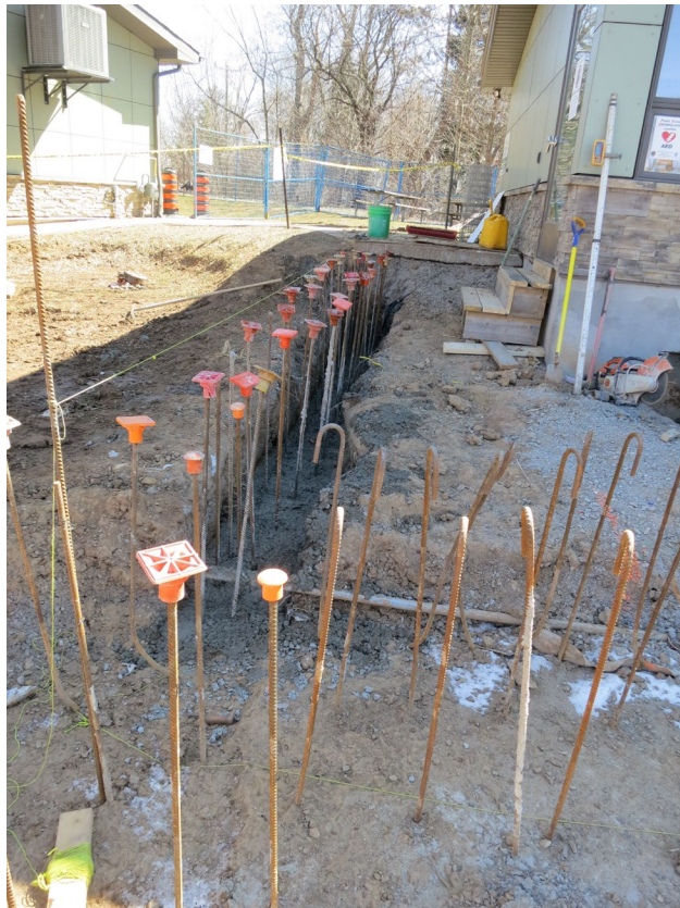
77 - March 29th. Foundation was poured for the north deck wall. The forming of all the deck walls will take place early next week.
