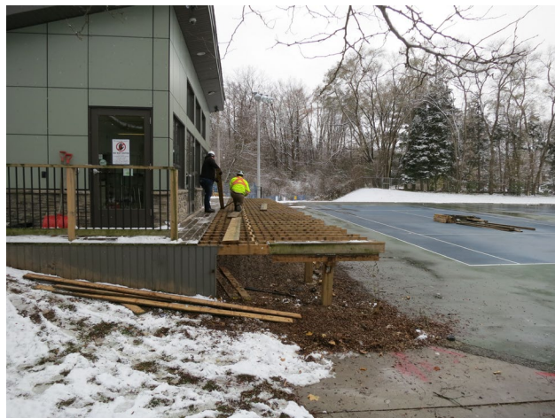
9 - Removal of wooden deck to be replaced by a concrete one ( fire regulation).
