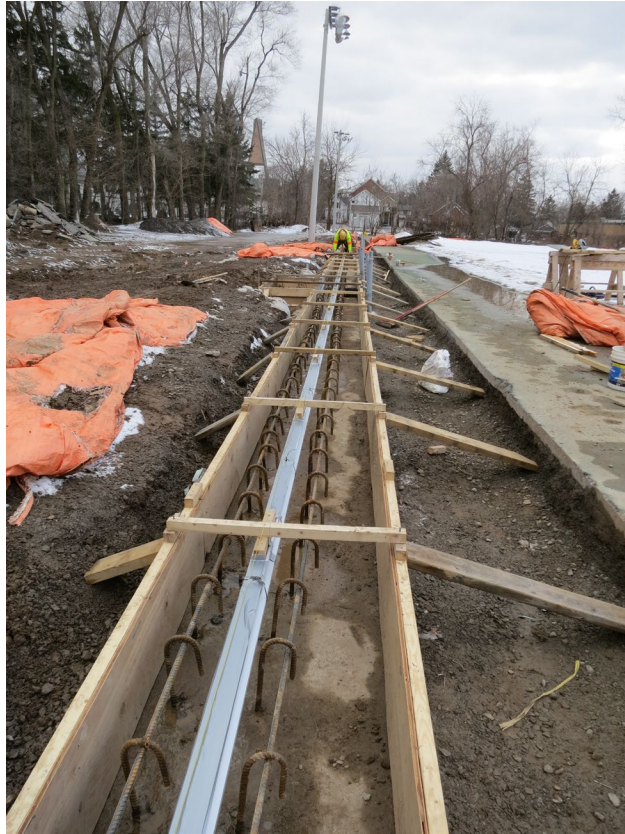
64 - March 8th. Twenty two meters of formwork for the top section of the grade beam ready for the concrete. The concrete will be poured on March 9th. Please note the aluminum channel in the middle of the form work. The bottom of the Dome fabric will be inserted in this channel.
