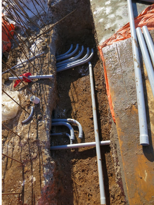
55 - Jan. 31st. Installation of the electrical conduits. Club house is on the left side of the picture.
