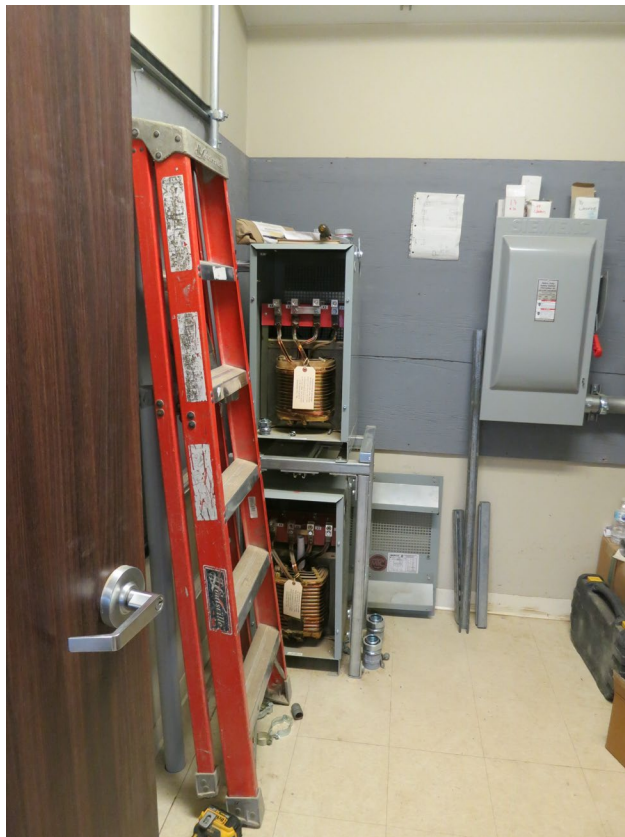
95 - April 21st. Installation of two transformers in the electrical room (former Pro's room).
