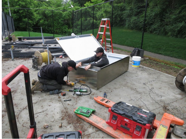
126 - June 9th. Electricians drilling holes for the installation of the electrical cabinet. I trust the fellow in the cabinet is wearing his safety boots.
