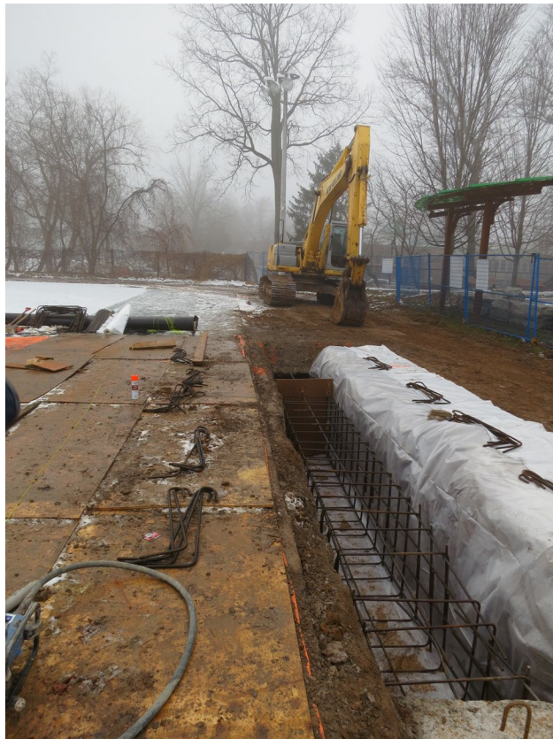
48 - Jan. 13th. One more day and the crew will be at the N/W corner of the courts and than they can tackle the remaining side, namely the west side.
