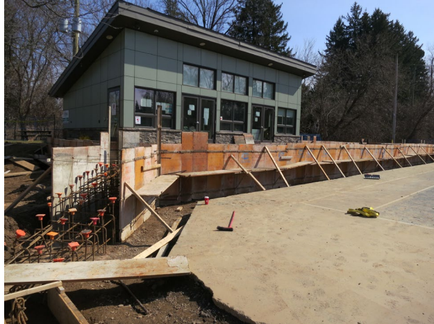
80 - April 5th. A sub- contractor installed the forms for the deck walls.
