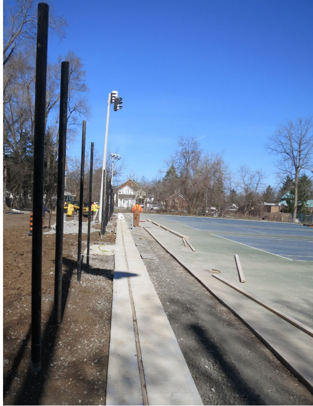
96 - April 22nd. Installation of the fence posts on the south side of the courts. The area between the posts and the grade beam will be concrete. Note workman compacting the gravel before Burlington Paving will be paving the conduit trenches on Monday, April 25th.
