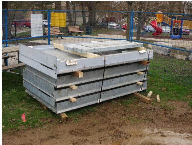
101 - April 26th. The four exit doors for the Dome were delivered today. These doors will be installed permanently. The combination unit (revolving door and pressure chamber) is under construction and will be delivered asap.
