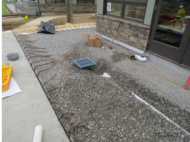
100 - April 25th. One of the drains to catch the runoff from the deck.
