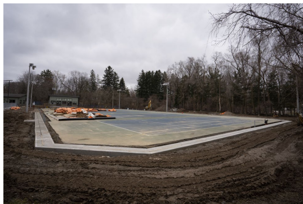
75 - March 28th, Overall view of the courts with the grade beam almost completed on three sides. The last section on the north side was poured this morning. Tomorrow, Tuesday March 29th, Demik will start the construction of the deck walls.
