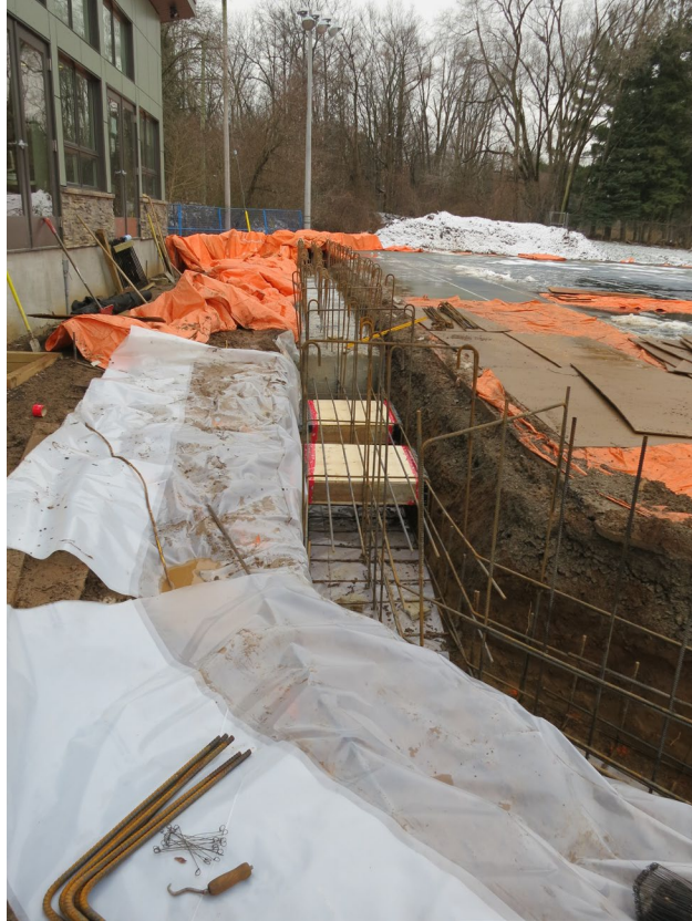
45 - Dec. 30th. This picture shows the foundation for the deck wall with the location of the form work for the two slots.
