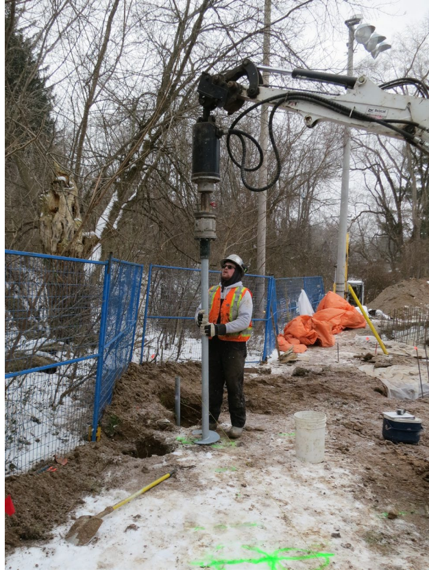
35 - Dec. 22nd. Helical Pile installation. Helical piles are a manufactured steel foundation anchor. The purpose of a helical pile is to provide foundational support for structures. In our case, required for the construction of the concrete deck and the wood deck, immediately south of the clubhouse..
