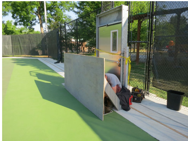
129 - June 22nd. Final repaired section of the court surface. ACS used the previous US Open green paint when the courts were constructed.
