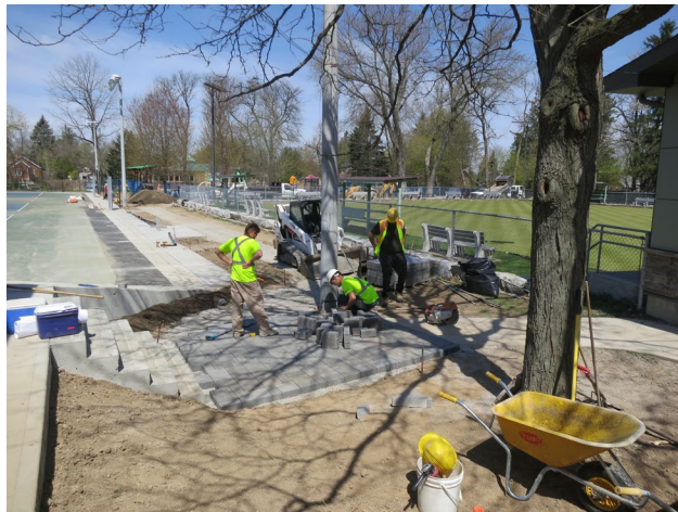
109 - May 10th. Installation of the interlocking walkway by the landscapers. Beneath the walkway is the existing infiltration system and therefore we had to use interlocking stones and not concrete.
