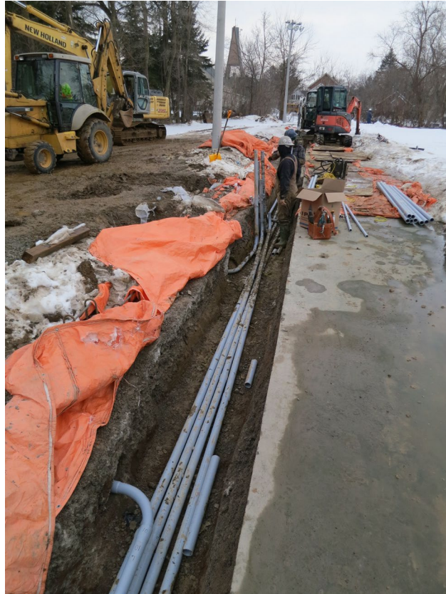
60 - March 1st. Installing electrical conduits on the south side of the courts.
