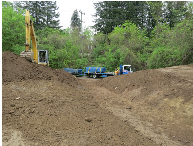
118 - May 19th. Infiltration unit backfilled and path to be graveled. The hoarding around the construction site was removed today.
