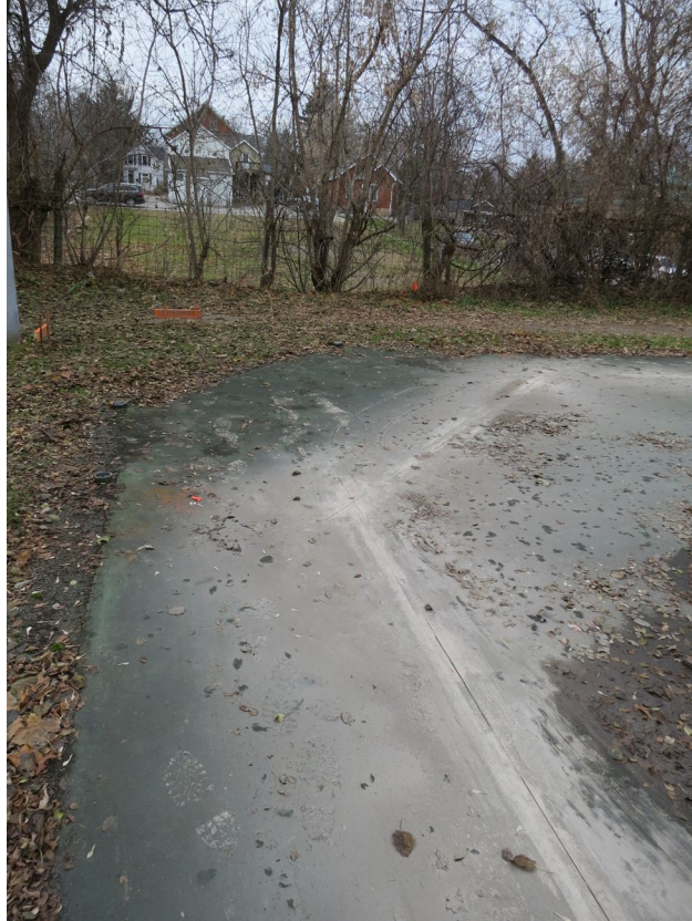
16 - Asphalt strip to be removed for the construction of the grade beam.
