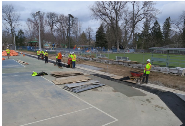
97 - April 25th. Burlington Paving paved all the conduit trenches this morning and they were finished by noon.
