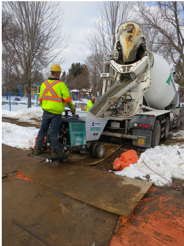
52 - Jan. 19th. Delivery of the concrete mix for the N/W corner of the courts.
