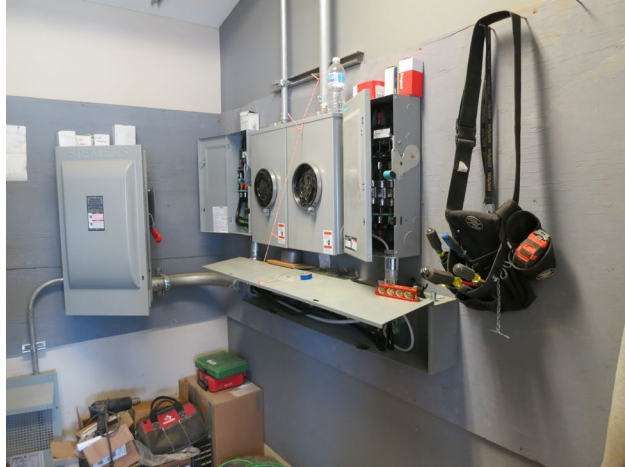
108 - May 10th. Electrical panels will be on three walls of the electrical room.
