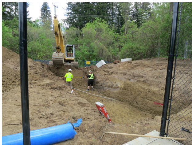
116 - May 17th. Construction of the storm water management infiltration system. This trench will be filled with 2 inch clear stone.
