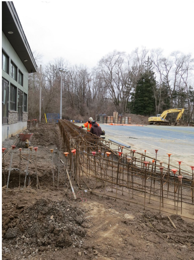
79 - April 1st. Deck wall ready for forming and the electricians are installing conduits for the electrical outlets in the wall facing the court. The Dome is attached to the top of the deck wall and also on top of the two transition walls on either side of the deck wall.
