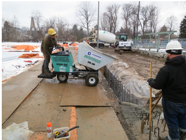
46 - Jan. 5th, 2022. Pouring of concrete for the foundation of the grade beam at the main entrance to the Dome. At this location, there will be a revolving door and an entrance for wheel chairs.
