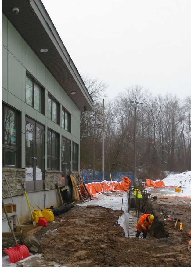
40 - Dec. 29th. Installation of the reinforcing steel for the foundation of the deck wall. Please note the polyethylene sheet. This sheet is to provide a "slip-plane" to prevent frost adhesion between the soil and the foundation wall concrete.
