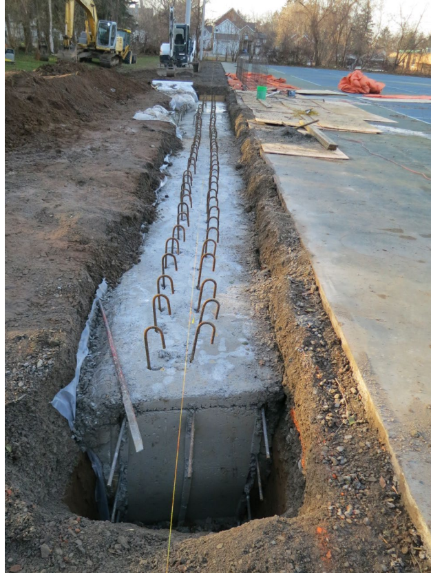
29 - Phase I of the grade beam completed. Phase II will be the concrete cap on top of Phase I, and this cap will house the aluminum rail holding the Dome fabric in place.
