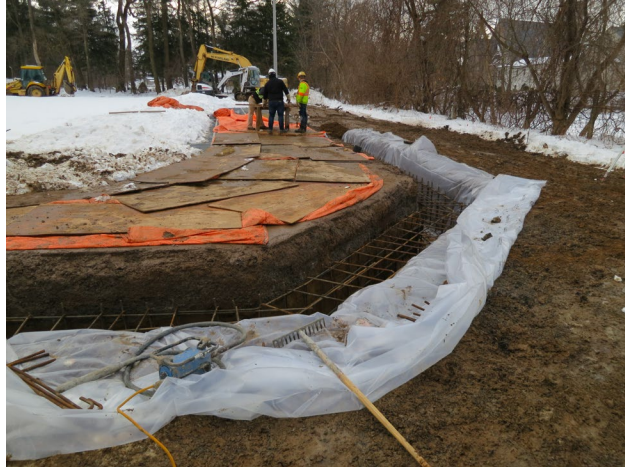
51 - Jan. 19th. N/W corner of the courts. Trench ready to receive 18 cubic meters of concrete mix.
