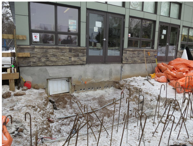
54 - Ja, 27th. Ten holes drilled into the lower wall of the club house for the electrical and security PVC conduits.
