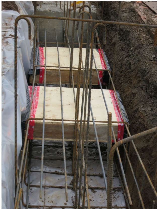
44 - Dec. 30th. Form work to create two slots, each 1 m wide X 0.2 m high, required to slip electrical conduits through.
