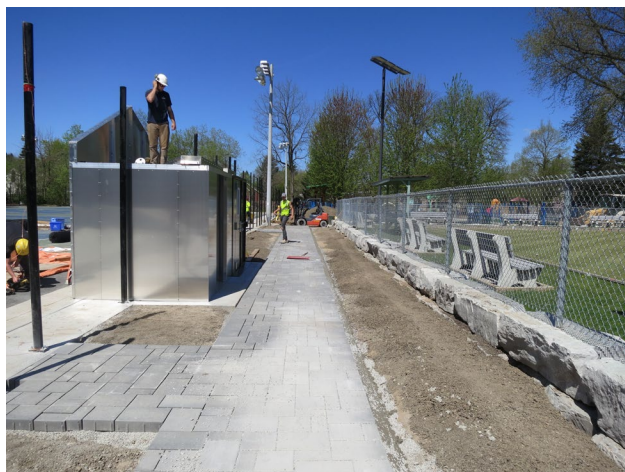
113 - May 13th. Interlocking walkway leading to the main entrance of the Dome and to the entrance and exit gates for summer play.
