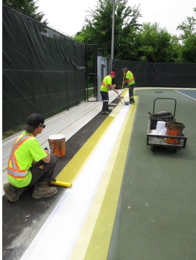
128 - June 15th. Repair of court surface by Ancaster Court Services (ACS). Laying and gluing of fiberglass screens prior to painting.
