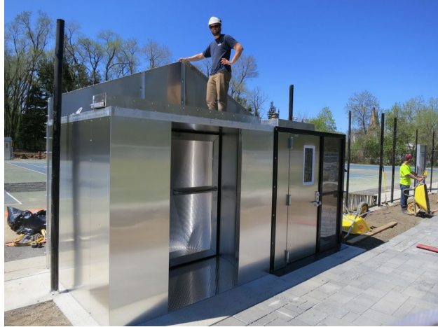
111 - May 13th. The Combo unit was delivered this morning and Demik is completing the installation.
