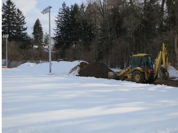
53 - Jan. 19th. All that excavated material piled up has to be removed from the site and can now be hauled away, since the test results of the soil samples determined that it is "clean soil".
