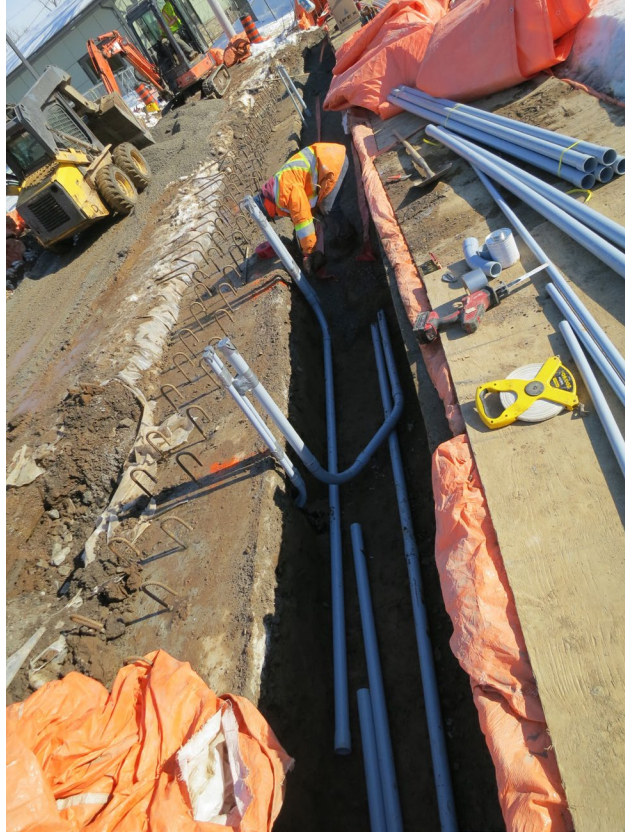
56 - Feb. 9th. Installation of electrical conduits on the north side of the courts. Risers at the "combination" entrance unit to the Dome.
