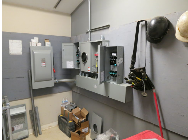
94 - April 21st. Installation of all the electrical equipment necessary for the operation of the Dome's mechanical equipment and lights.
