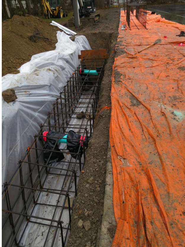
30 - Grade beam across from proposed mechanical pad. Note 6" diam. PVC pipes for electrical conduits to slip through.
