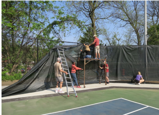
121 - May 21st. Big day today. Nets and windscreens are being installed by an army of volunteers.
