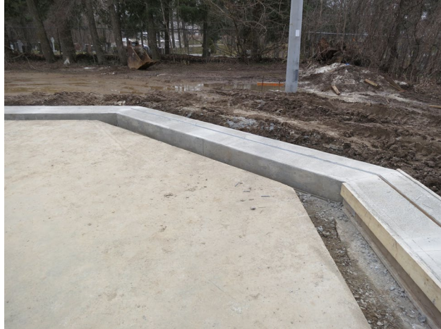
68 - March 18th. S/W corner of court. Top section of grade beam was poured in this area on March 17th and the forms were removed on March 18th.
