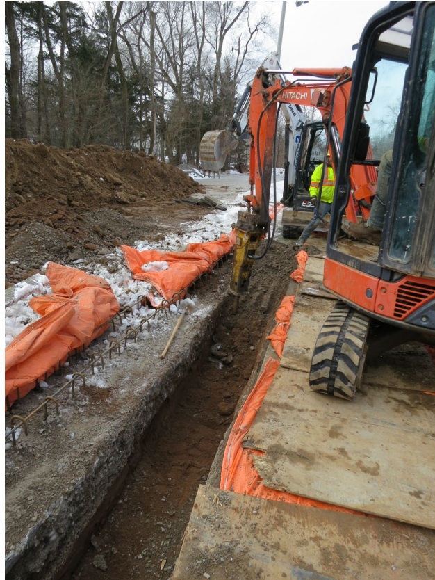
59 - Feb. 23rd. Since the frost is at least 4 feet down, Demik has to use a Hydraulic Breaker/ Jackhammer to loosen the soil. The trench is for the installation of the electrical conduits to be installed on the south side of the courts.
