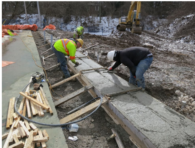
65 - March 9th. Seven cubic meters (m 3 ) of concrete was used to fill the 22 m of form work.
