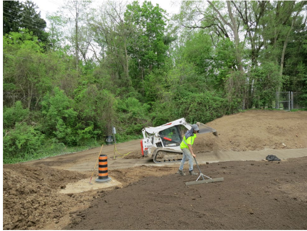
120 - May 20th. Path almost completed and top soil being spread for sodding the areas starting next week.
