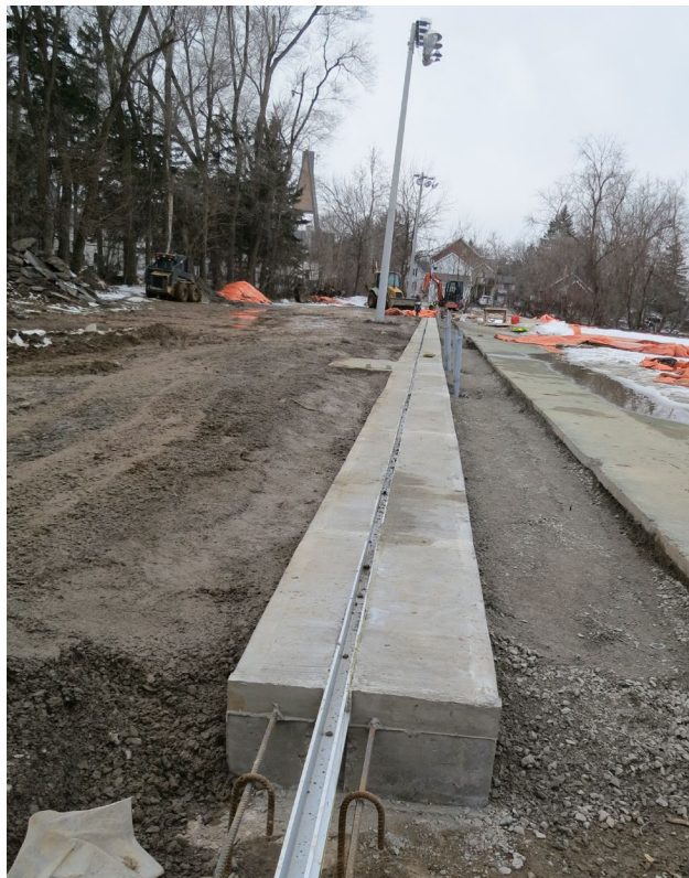
67 - March 14th. A great view of part of the grade beam on the south side.
