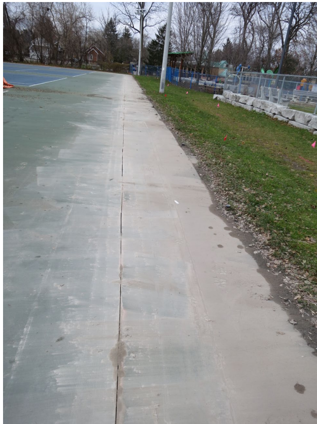
15 - Asphalt strip to be removed for the construction of the grade beam.
