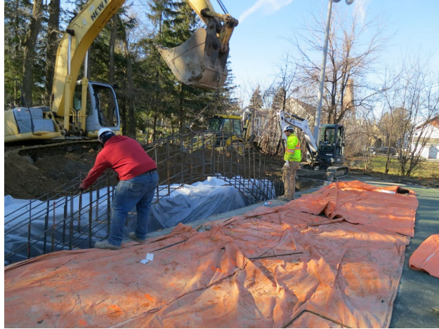
32 - December 17th. No, they are not building an "archway". The lowering of reinforcing steel into the trench and the concrete was poured this afternoon.
