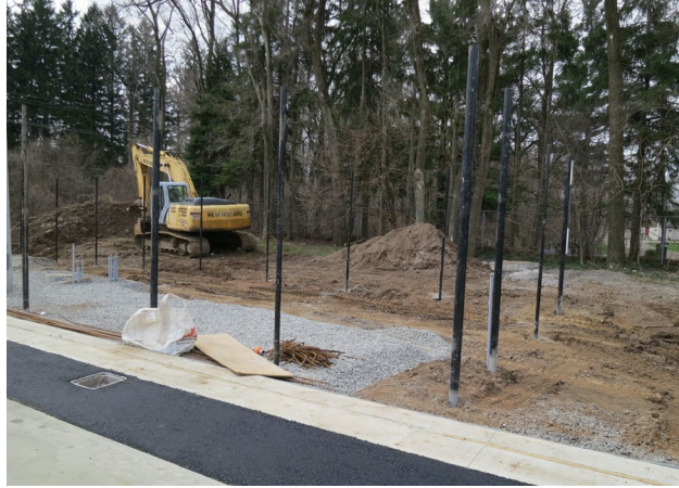
98 - April 25th. Construction of the mechanical and storage shed pad. Notice the fence posts around the proposed pad.
