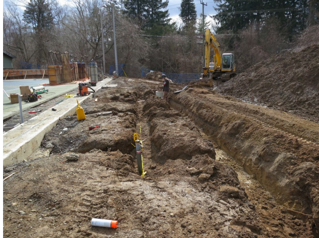
83 - April 7th. Trenches for the installation of the electrical conduits and the two hand holes at the mechanical pad location.
