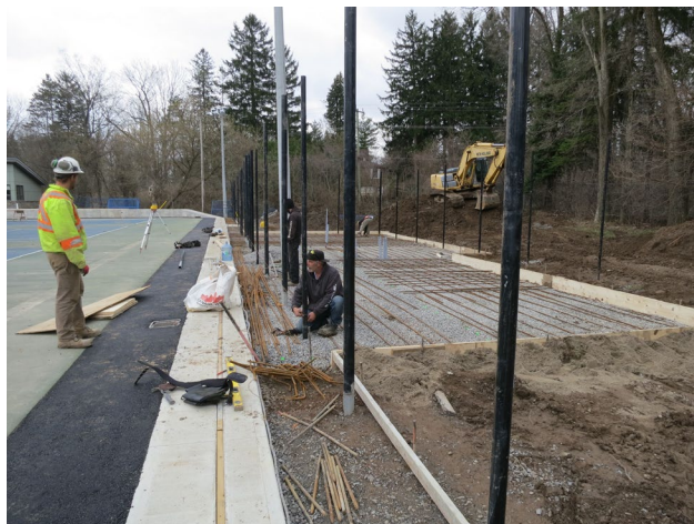
102 - April 26th. Installation of the reinforcing steel for the mechanical and storage shed pad. Concrete will be poured this coming Friday.
