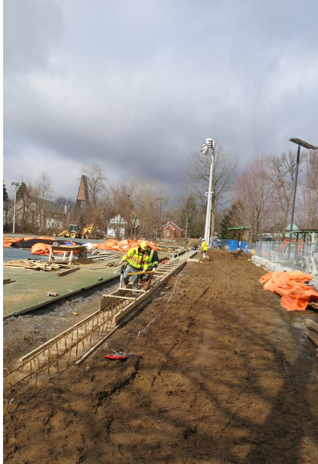
70 - March 25, Top of the grade beam approaching the deck wall on the north side of the courts, concrete will be poured on Monday, March 28th.
