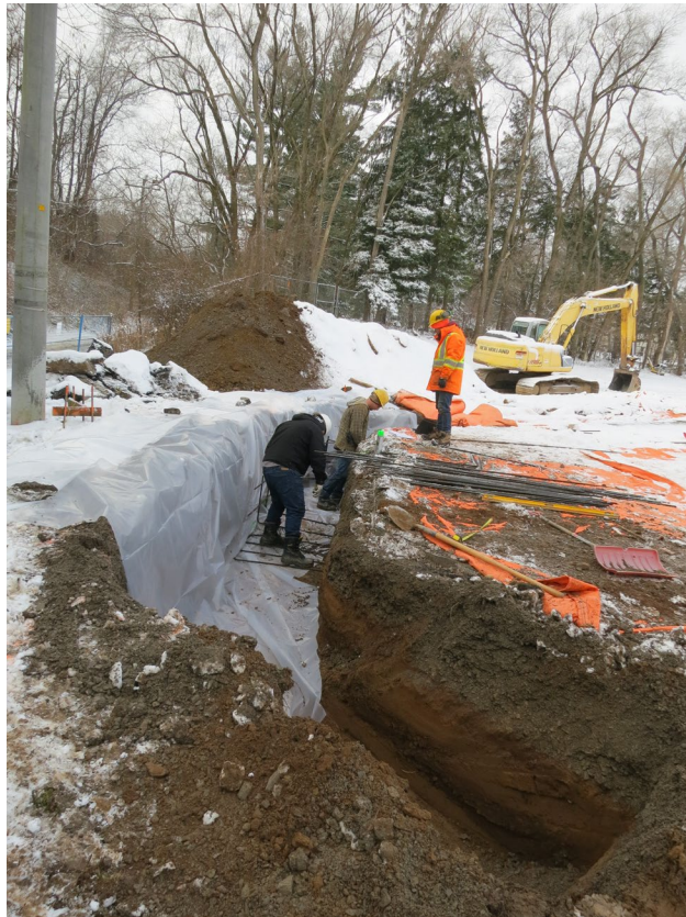
33 - December 20th. Construction of the grade beam at the South/East corner of the courts.
