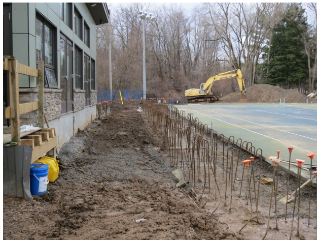
71 - March 25. Reinforcing steel of the deck wall and Demik will be forming the wall very soon.
