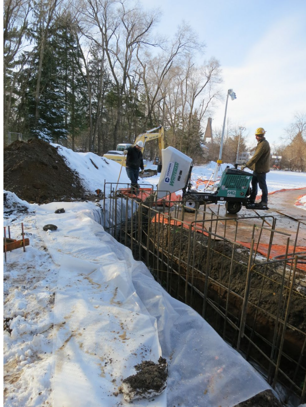
34 - December 20th. Pouring of the concrete at the South/East corner of the courts. The height of this section will gradually change from deck level to ground level.
