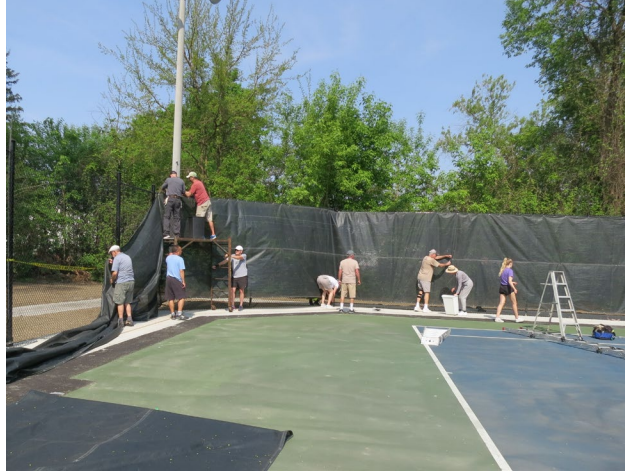
123 - May 21st. Great team work and the work was completed before the storm.
