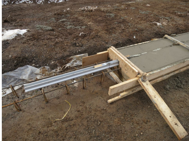
66 - March 9th. Clear view of the aluminum channel. The top of the channel is covered with tape to prevent concrete accumulating in the channel.
