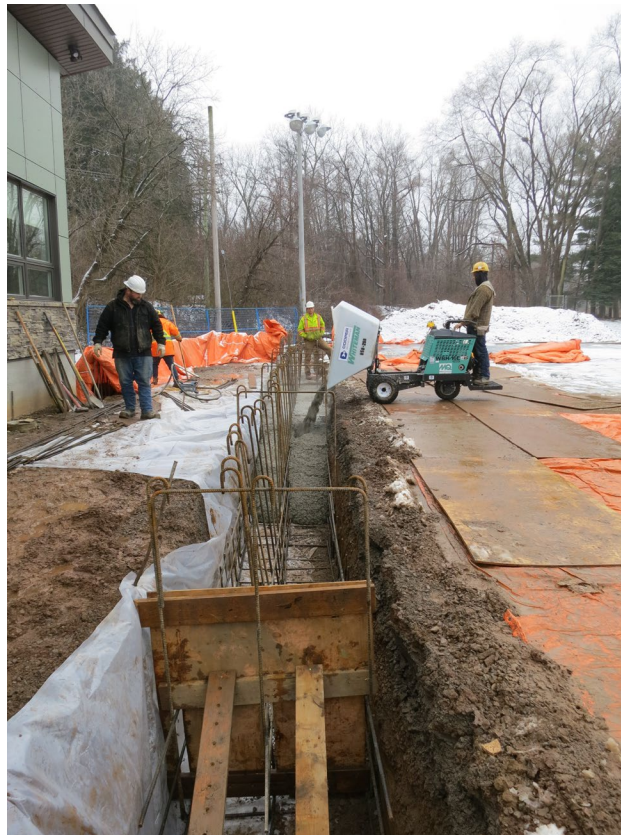
41 - Dec. 29th. The pouring of concrete for the foundation of the deck wall. Today, they poured 13 cubic meters of concrete.
