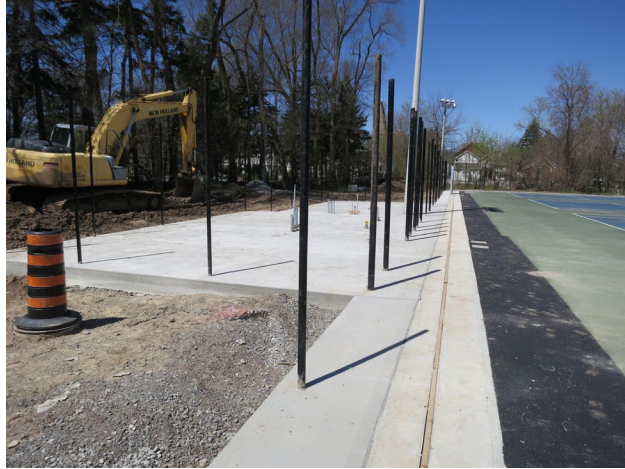
106 - 1st. week of May. Mechanical and storage shed pad. Court fence being installed.
