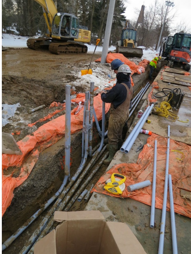
61 - March 1st. Conduit risers at the inside of the grade beam for the installation of the electrical junction boxes.
