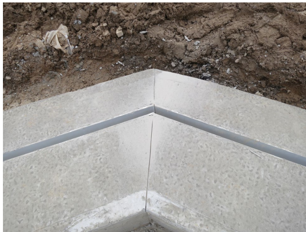
69 - March 18th. Need and clean construction of one of the 45 degree corners.
