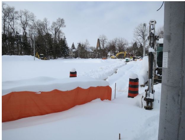
50 - Jan. 18th. Snow clearing today before construction can continue. Three days of good "construction weather" will complete the foundation of the grade beam around the courts.
