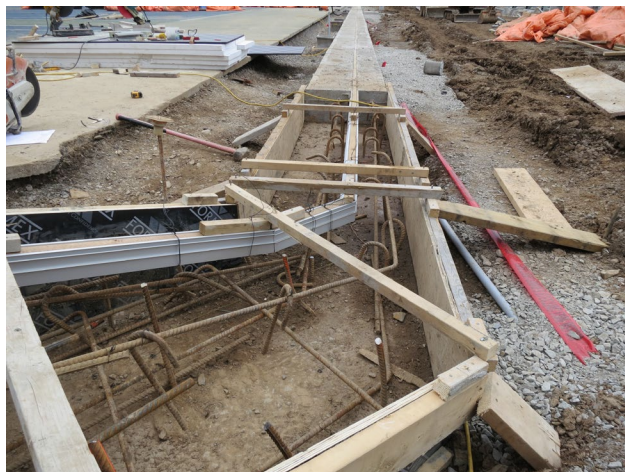
82 - April 6th. Notice the fine cut composite angels of the aluminum channel.
