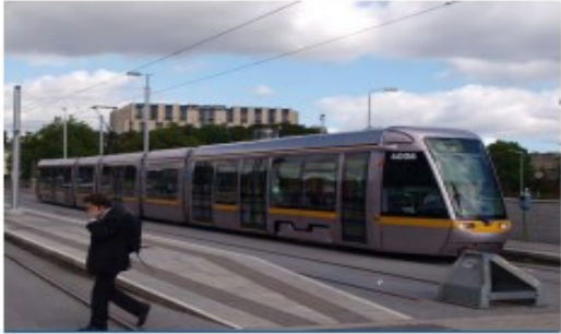
Overhead Catenary System (OCS)
