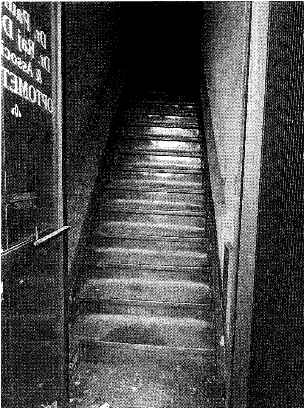
KING STREET ENTRANCE 2 – separate entrance for 2 nd floor tenant – 19 th century wood trim indicates an original staircase – the treads and risers have been clad in vinyl
