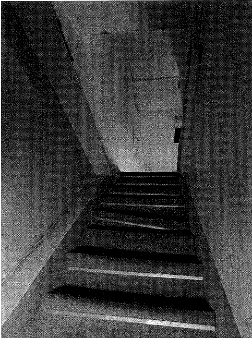
ATTIC STAIRS – steep staircase to the attic with no handrails – evidence of rot in the stair treads & stringer
