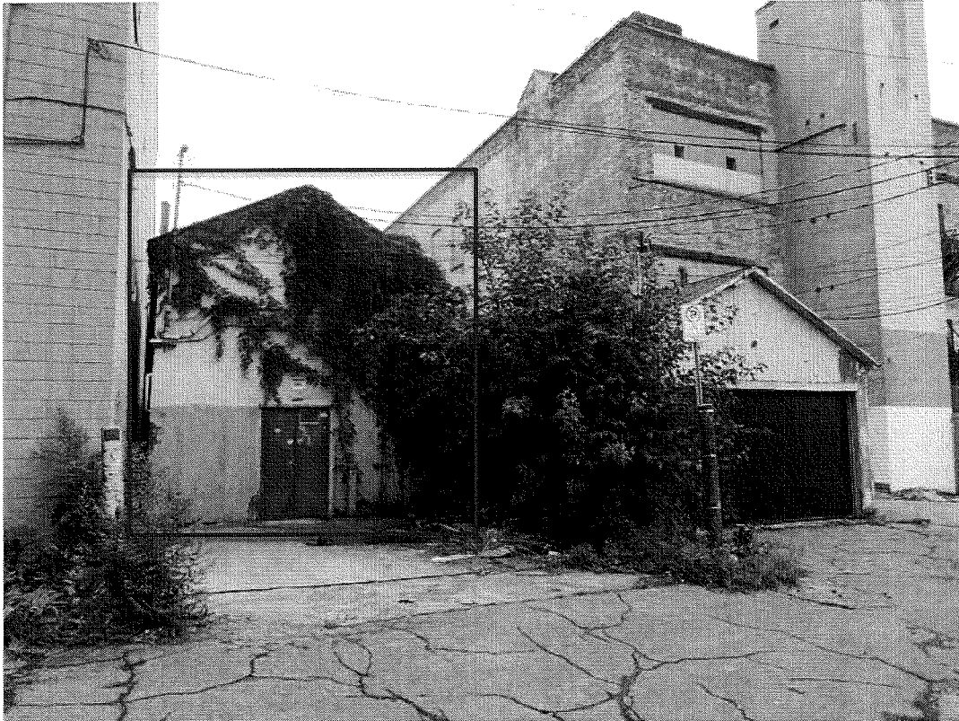
REAR FAÇADE - backs onto an alleyway and surface parking lot – there is a 1.5-storey garage at the back
