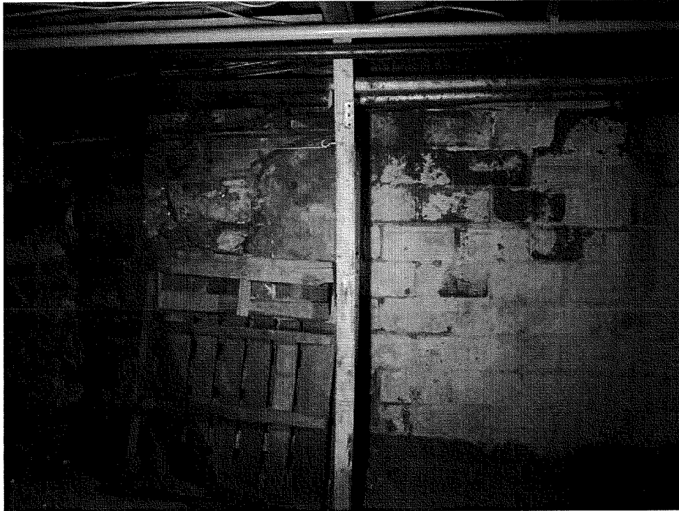
BASEMENT – rubblestone under the historic portion at the front and concrete block under the later additions at the back
