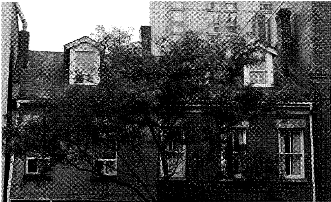
Original roofline is intact but is in very poor condition
