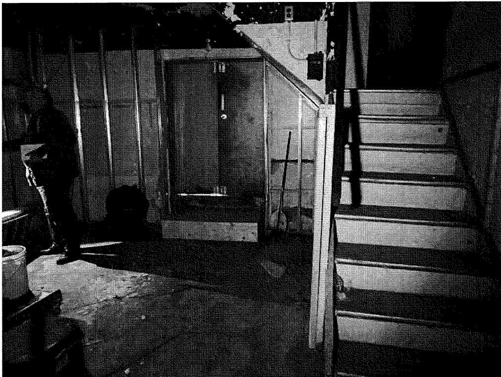
1 st FLOOR – rear section – this area has been gutted – no historic fabric
