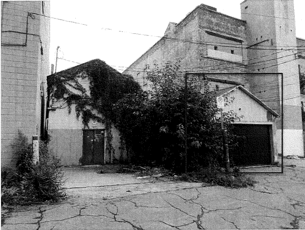
REAR FAÇADE - backs onto an alleyway and surface parking lot – there is a metal clad garage at the back
