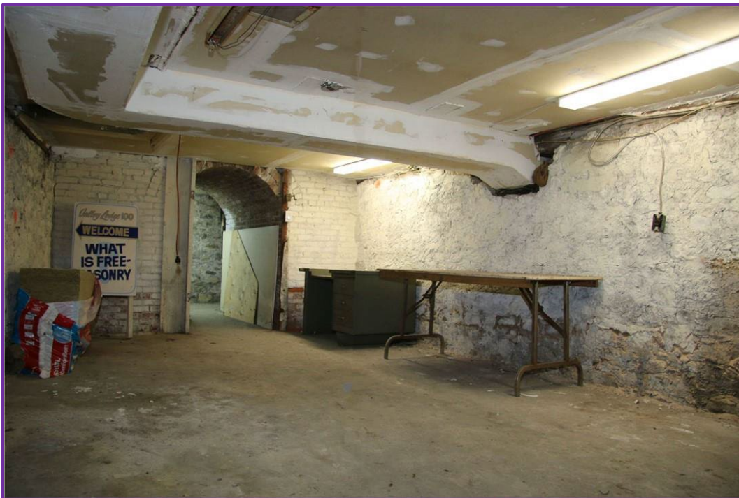
Basement area with rubblestone walls looking towards a barrel-vaulted archway (orientation unknown).
