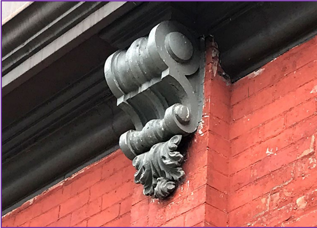
Close-up view of one of the galvanized iron brackets mounted to the brick piers below the cornice defining to the top of the first storey. AG September 2022
