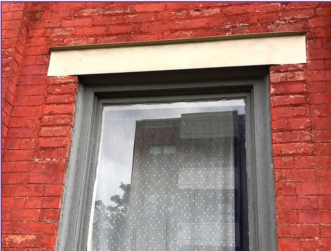
Close-up view of the stacked bricks framing the top of the windows and the aluminum now protecting the brick masonry lintels, once obscured and protected by the galvanized-iron window hoods. AG September 2022
