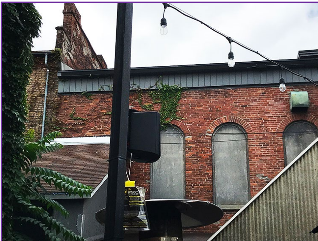
A section of the rear façade viewed from King Street, showing four round-arched window openings, one bricked in and largely obscured by a shed-roofed addition and three filled in with wood panels.
