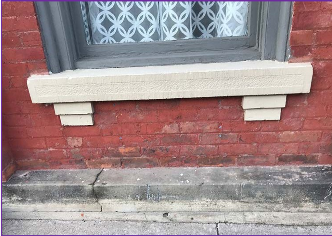
Closeup view of one of the six identical stone sills and the projecting cut stone blocks of the above grade foundation wall. AG August 2022
