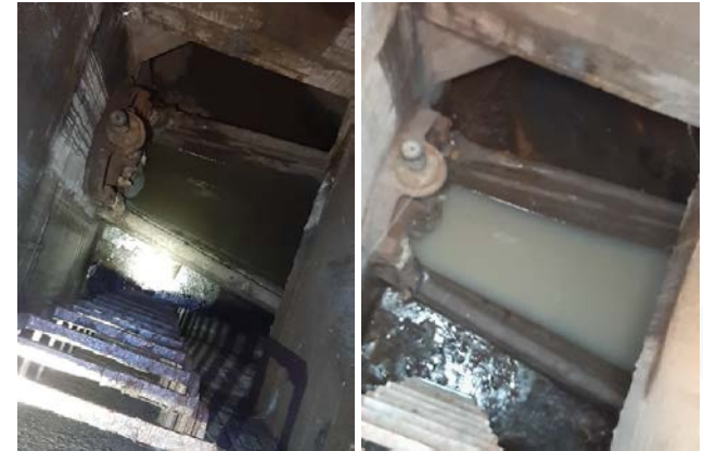
Dunn Ave – suspended trough regulator
