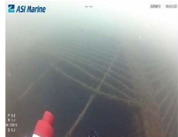
Low lift raw water intake
