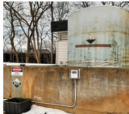
Dundas Ferric Tanks
