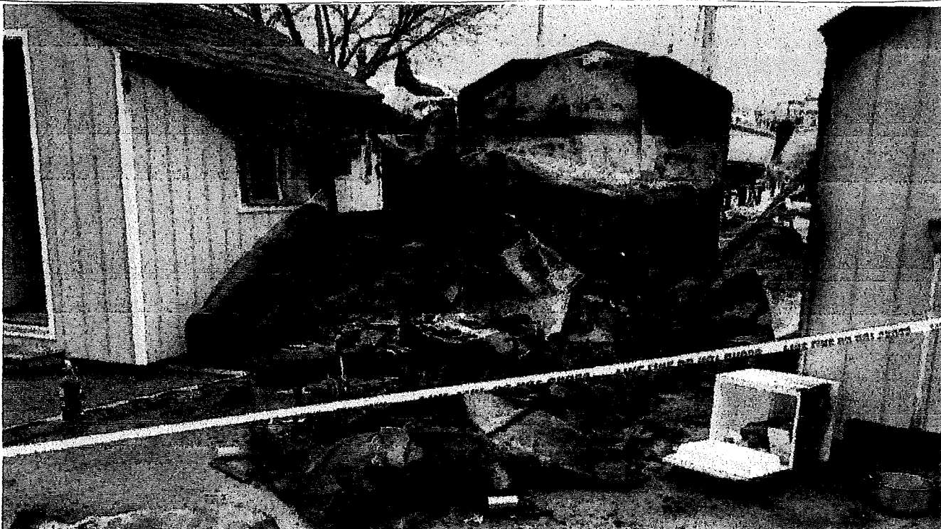
A sleeping cabin at Portsmouth Olympic Harbour in Kingston burned to the ground in the early morning
