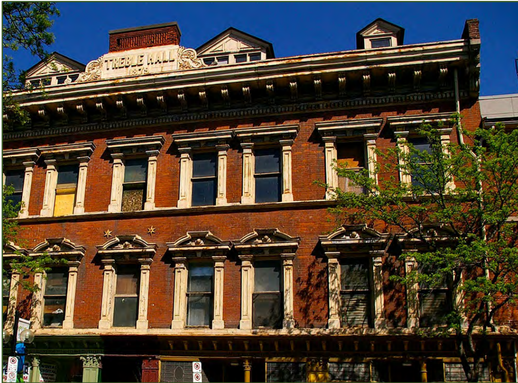
Closer view of the galvanized-ironwork showing exposed metal where the paint has worn off.
