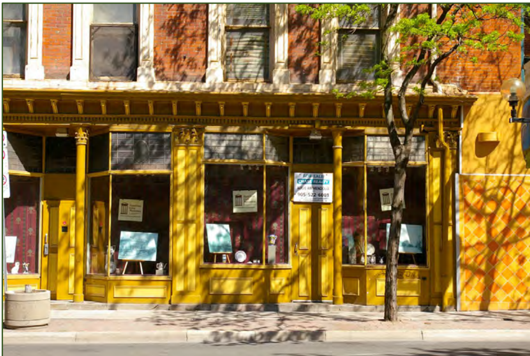
Close-up view of one of the four cast-iron storefronts featuring round freestanding columns and pilasters with Corinthian capitals. The attenuated columns separating the glass panes of the windows could only have been fabricated of cast iron due to its tensile strength.
