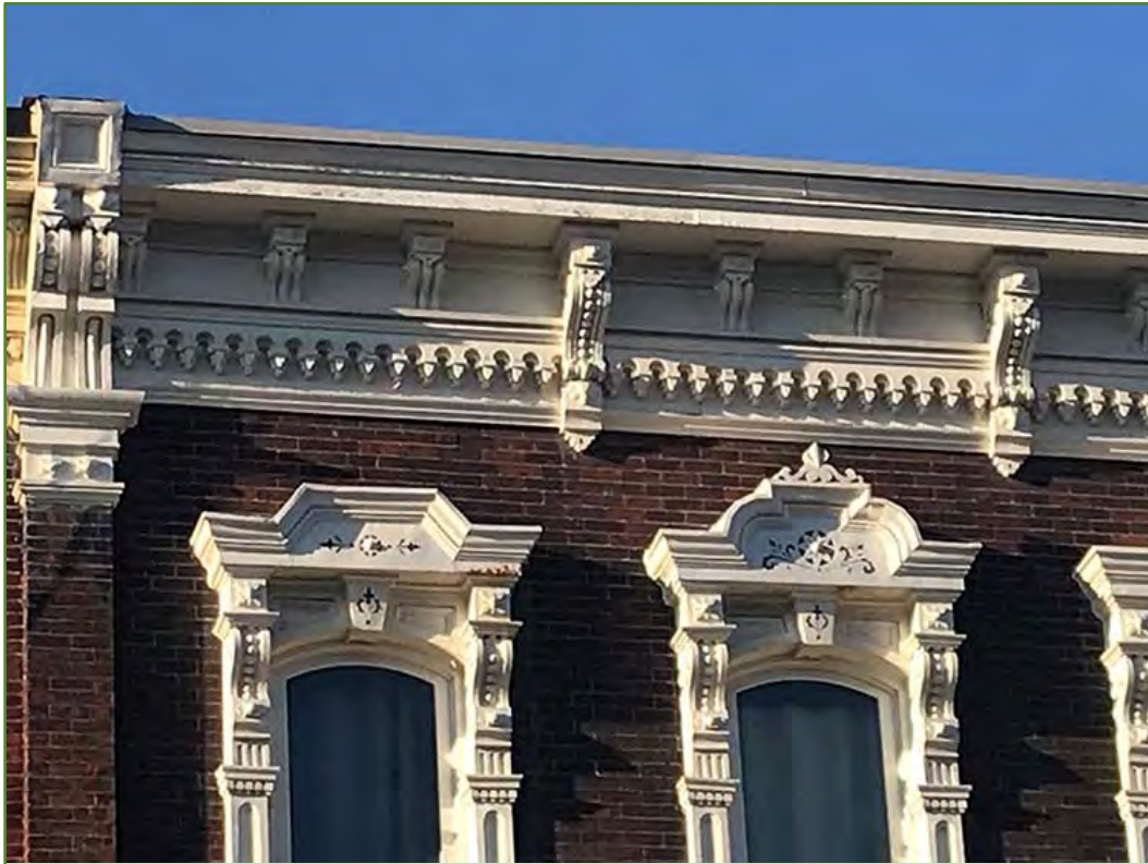
Close-up of the cornice and window surrounds of #11. Photo by the author, September 2021.
