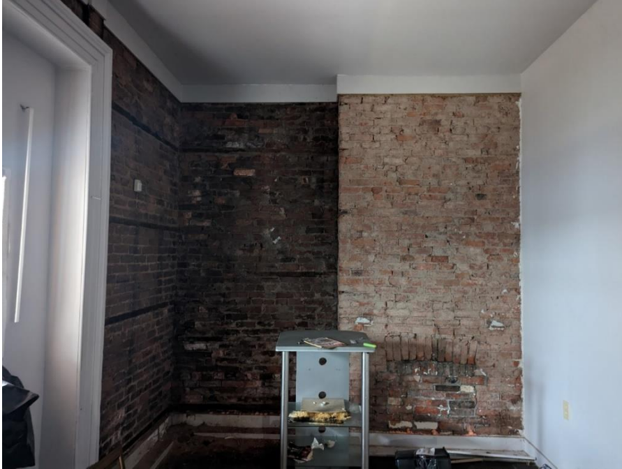
115-117 George Street, Interior Brick Wall City of Hamilton, January 20, 2023
