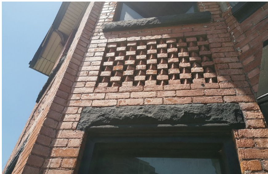
Close-up at exterior wall, showing the checkered brick pattern at the spandrel. The walls appear to have a remnant thin film over the brick surfaces. Note the modern cladding at the soffit above.
