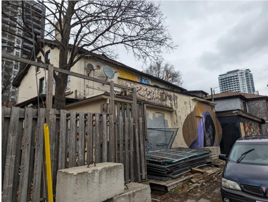
115-117 George Street, South and West (Rear and Side) Elevations City of Hamilton, January 20, 2023
