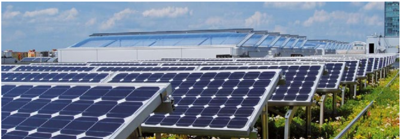
Cool roof and solar panels help reduce the heat island effect and improve energy efficiency.
