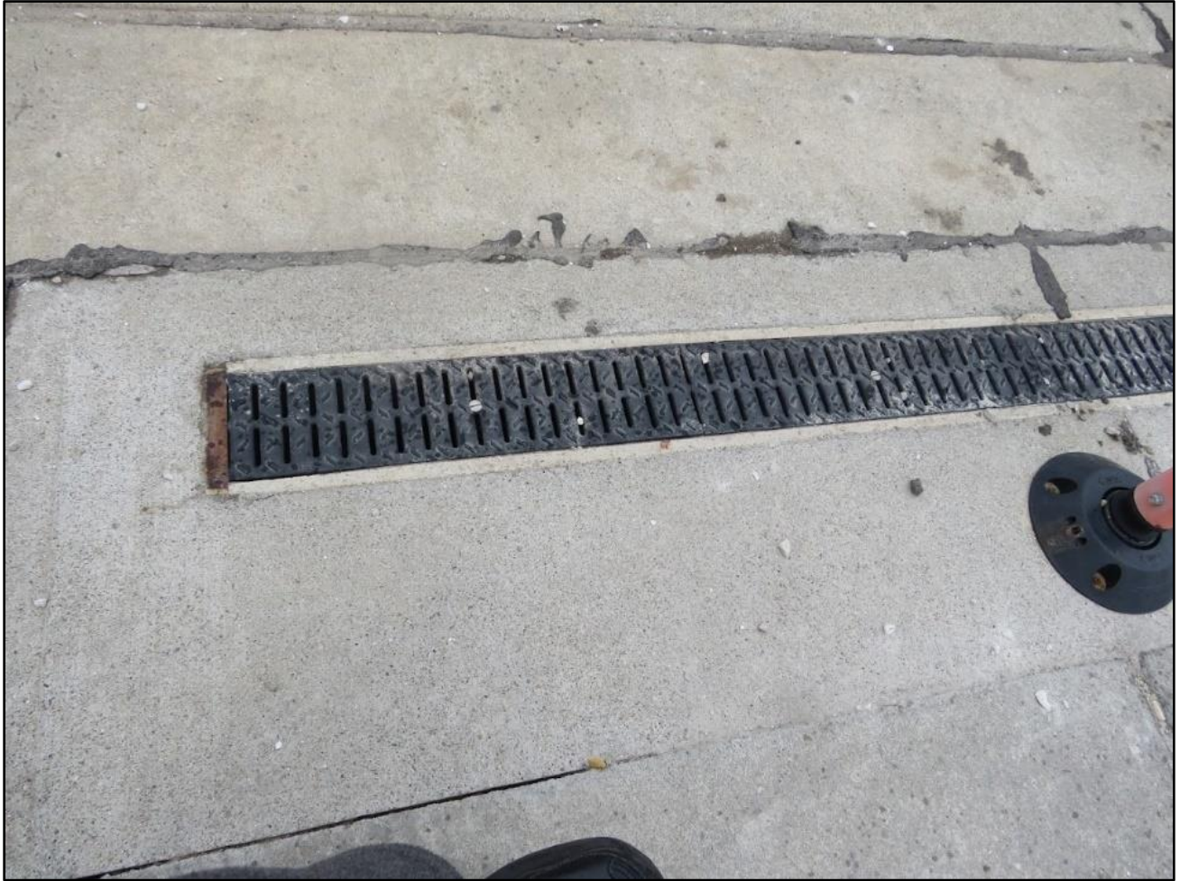
Figure 11: Checkplate drainage channel beside pedestrian pathway. *Minimal tactile warning of danger.
