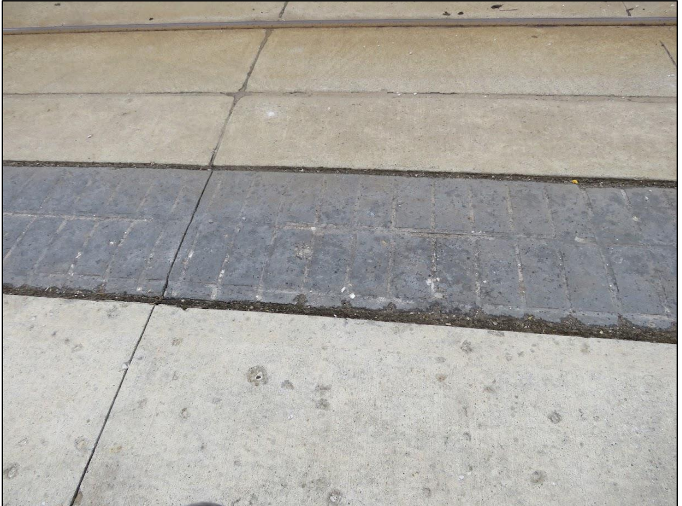
Figure 7: Image of safety tactile markings on emergency pedestrian pathway
