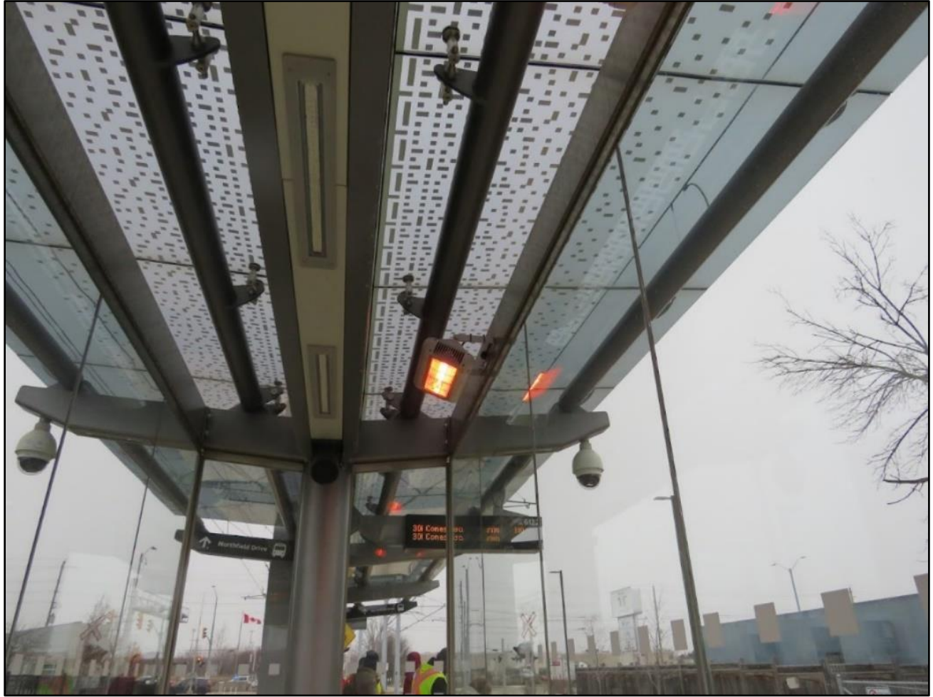
Figure 5: Image of an LRT station platform shelter with arena style heaters and sprinkler system
