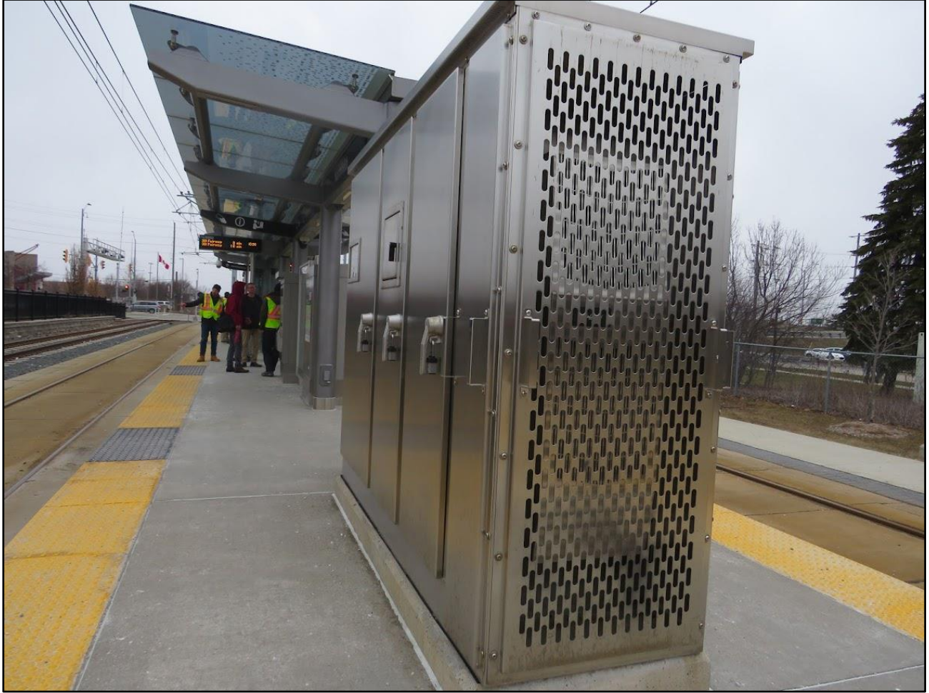
Figure 19: Power box on platform. *Hard to see and takes up a lot of space. Not much room for a wheelchair to pass without running over the tactile plates.
