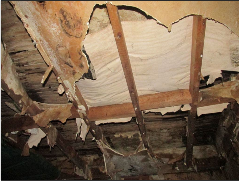
Figure 3: View of damage to an interior ceiling.
