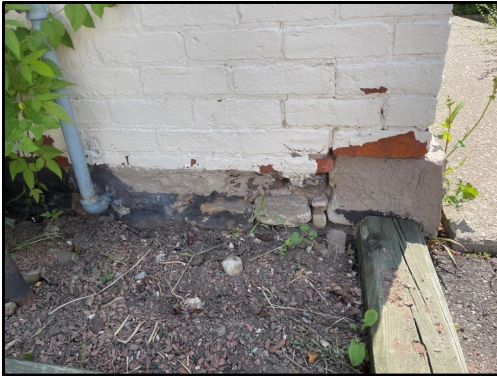
Image 15: Detail of Southwest Corner of 215 King Street West Fieldstone Foundation (Photo taken on August 6, 2021; Facing East)
