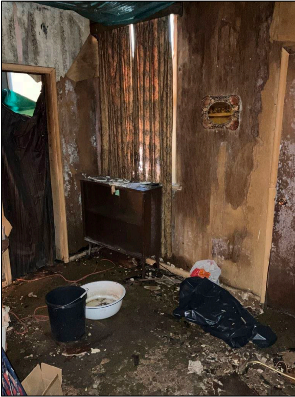
Figure 9: View of damage to interior.
