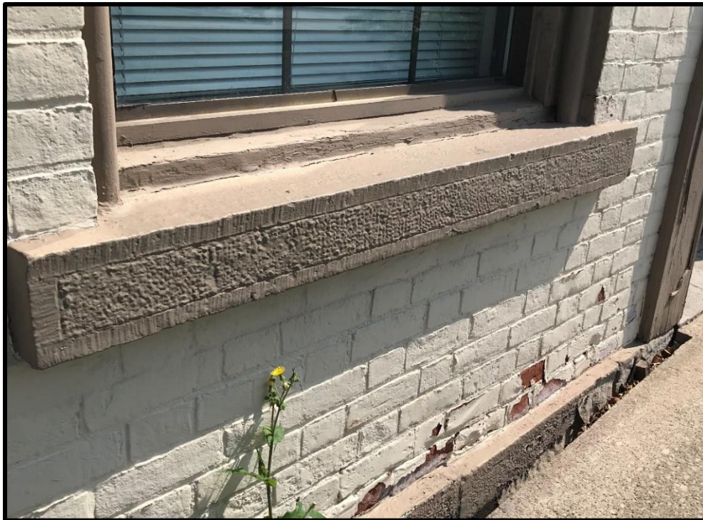
Image 10: Rusticated Sill on 215 King Street West Façade (Photo taken on August 6, 2021; Facing North)
