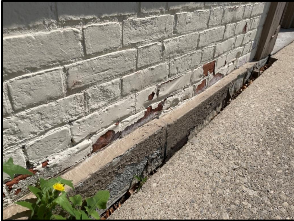
Image 13: 215 King Street West Elevation Brickwork in Flemish Bond Showing Signs of Deterioration (Photo taken on August 6, 2021; Facing North)
