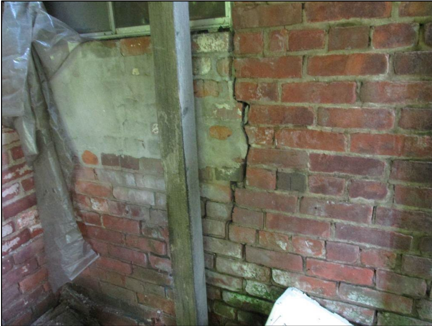
Figure 1: View of water damage under exterior window.
