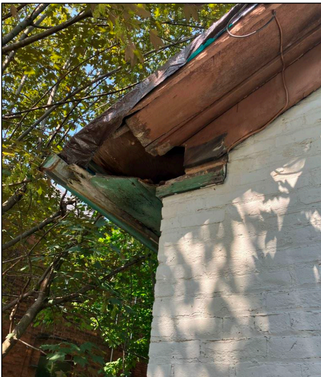
Figure 2: View of damage to soffits.
