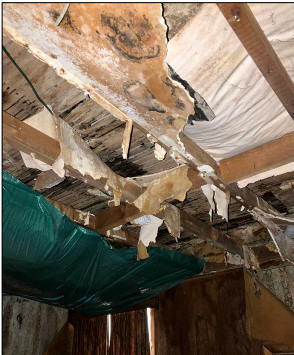
Figure 10: View of damage to an interior ceiling.
