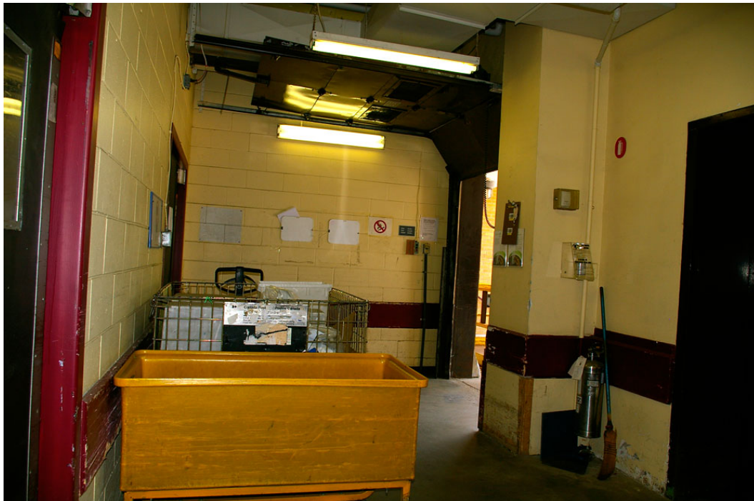
Photo 41: The 1979 Mail Lobby enclosed with concrete block partition walls, looking towards the south wall and the west-facing doorway with the overhead metal rolling door opening onto the loading dock. Visible on the far right is the elevator entrance.
