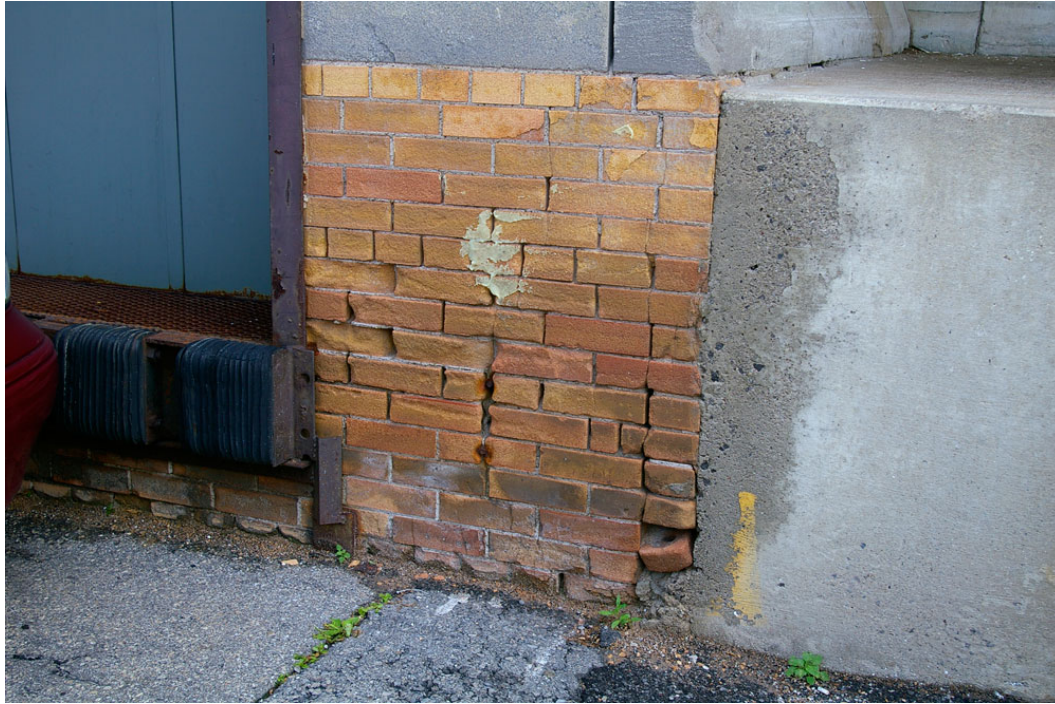
Photo 23: Detail of one of the two sections of deteriorated brick masonry foundation flanking the elevator doorway on the west facade. To the right is the concrete loading dock platform.
