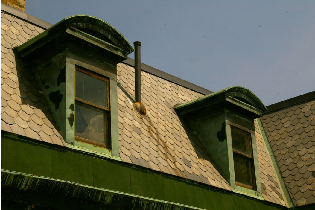
Photo 25: Close-up view of the scalloped slates and two of the three copper-clad dormers on the south face of the mansard roof. Photo taken from a window on the east facade of the second storey addition (see below). Shows some of the recent darker grey replacement slates (1990s repair work).
