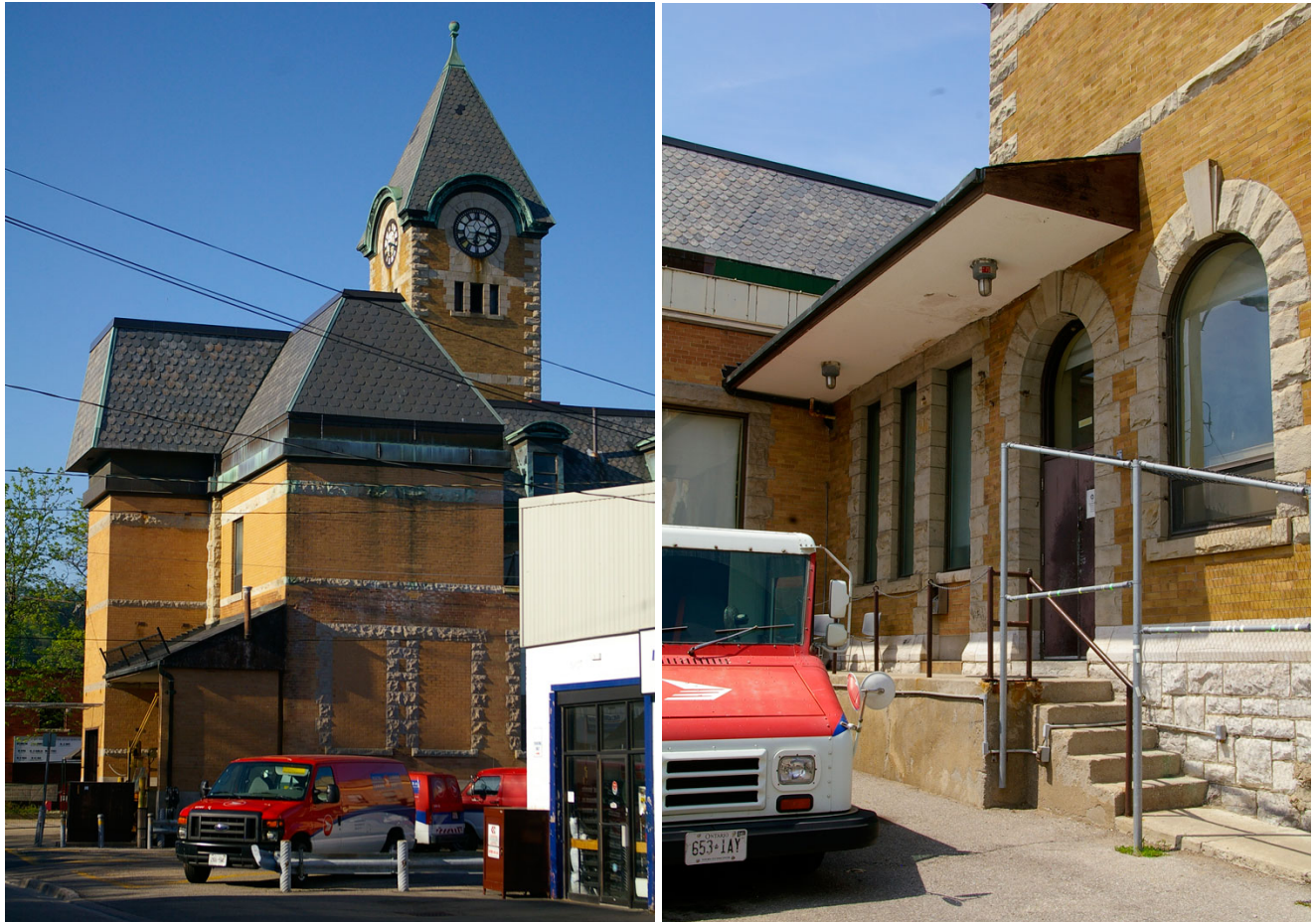
Photo 21 (left): Back wall of the west wing, showing the 1979 second storey addition, the shed roof addition to the loading dock with a solid brick masonry end wall and wood-clad roof gable, and the two ground floor windows blocked up at this time for the new rear stairwell.
