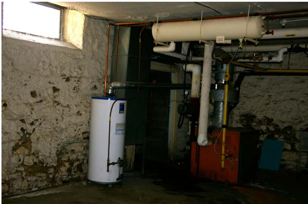
Photo 33: View of the south-east corner of the basement showing the existing gas-fueled boiler (first or second replacement for the original coal-burning boiler). The doorway behind the furnace, not shown on the 1911 Basement Plan (Figure 12), was located under the fourth window on the east facade, which has since been blocked up. It provided access to the coal chute ( Photo 11 ).
