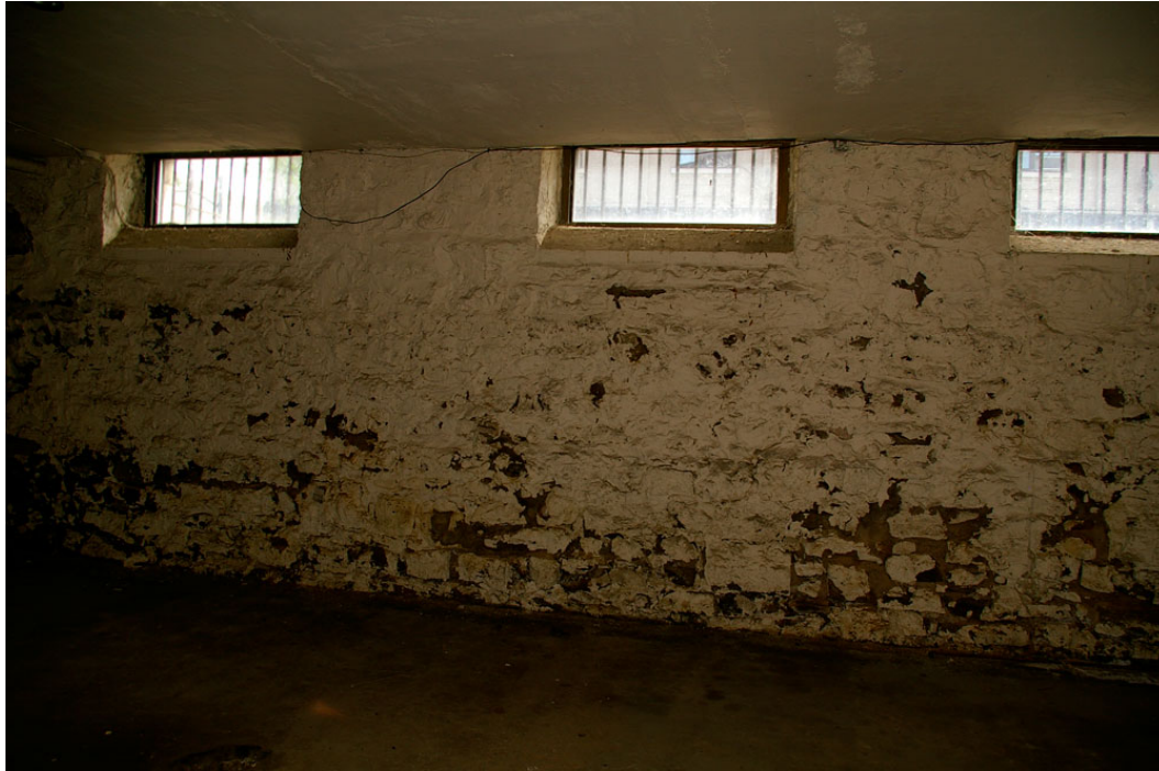
Photo 32: Section of the east wall of the basement of the original building showing the rubblestone construction and three of the four above grade fixed-paned wood windows with metal bars on the exterior.
