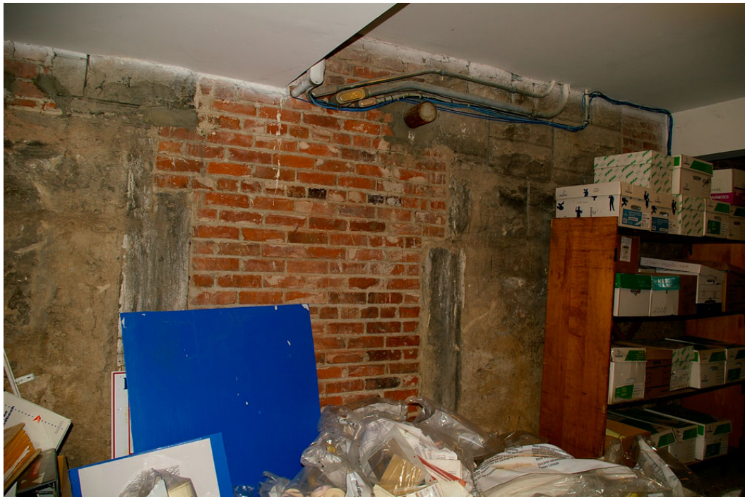
Photo 31: Inside face of the rear (south facing) stone masonry wall of the original basement with a section of brick masonry construction, the reason for which remains unclear.
