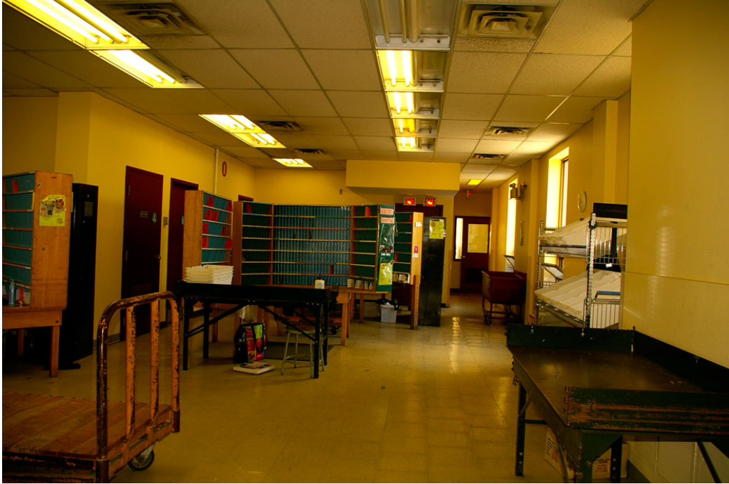
Photo 59: Second floor looking east towards the open doorway to the lunch room in the south-east wing, with three doors on the left: (from west to east) the janitor's closet, the men's washroom and the women's washroom (barely visible in the corner above the sorting booth). Directly ahead but mostly obscured from view is the doorway (fire exit) to the enclosed concrete block stairwell constructed as part of the 1979 renovations (A2: Figure 47 ).
