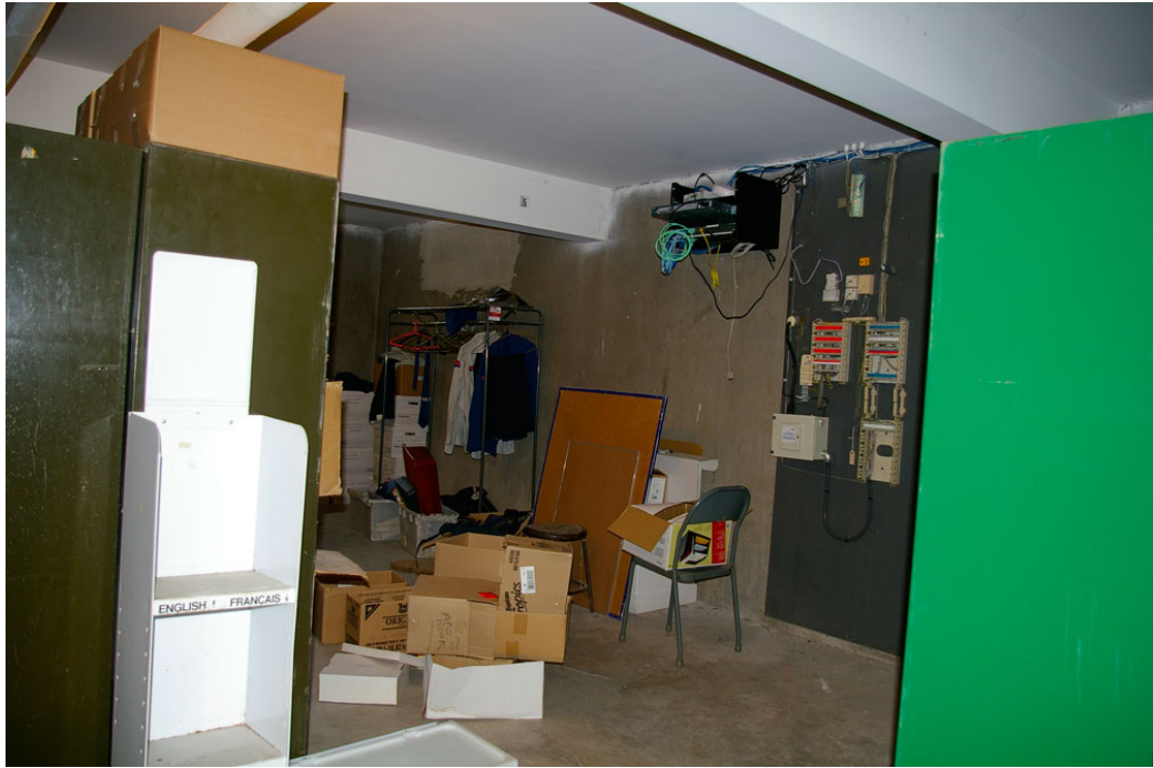
Photo 28: View of the concrete back wall of the pre-1949 rear extension, from close to its west wall looking south-east. Shows the poured concrete floor and the reinforced concrete beams supporting the floor above.
