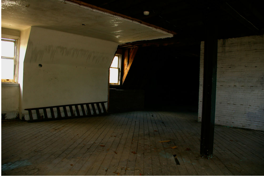
Photo 62: Third floor looking south-west towards the unfinished area on the west side with a plastered wall and section of the ceiling marking the footprint of the south-facing bedroom of the caretaker's suite. Visible is the steel I-beam column supporting the south-west corner of the corner of the clock tower. The south-east corner is supported by an identical column now embedded in the north-west corner of the 1979 concrete block stairwell addition, as shown in Photo 63 and Photo 64 .
