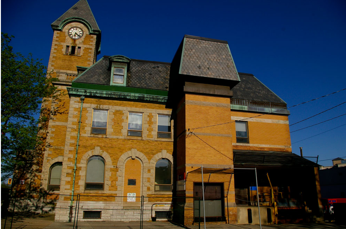
Photo 12: West facade showing the 1960 elevator shaft, and some of the additions and alterations made in 1979, including the second-storey addition behind the elevator shaft, the mansard roof wrapped around the mechanical room on top of the shaft, and the removal of steps in front of the west entrance, which had previously been partially blocked up for the installation of a mail receiver.
