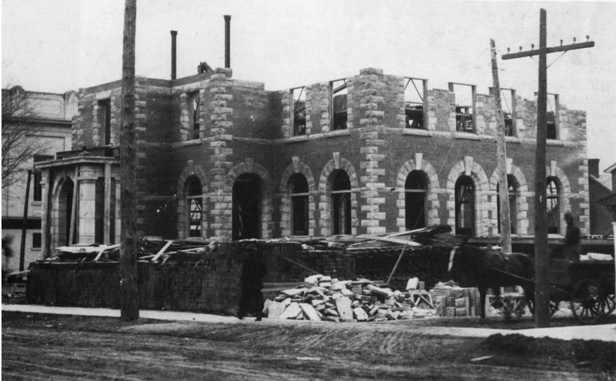
Figure 28: View looking south-east of the Dundas Post Office under construction, between the late fall of 1912 and the early spring of 1913 (based on the absence of foliage on the partially visible tree to the left). Surrounding the building are piles of bricks, stones and wood for bracing. Construction materials would have been brought short distances to the building site by horse and cart.
