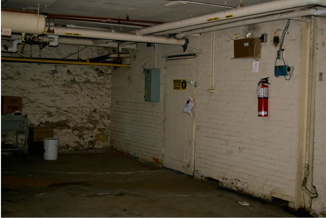
Photo 34: An oblique view of the east-facing brick masonry wall of the boiler room looking towards the rear (south) rubblestone wall, with hot water pipes and a cylindrical tank for the original boiler.
