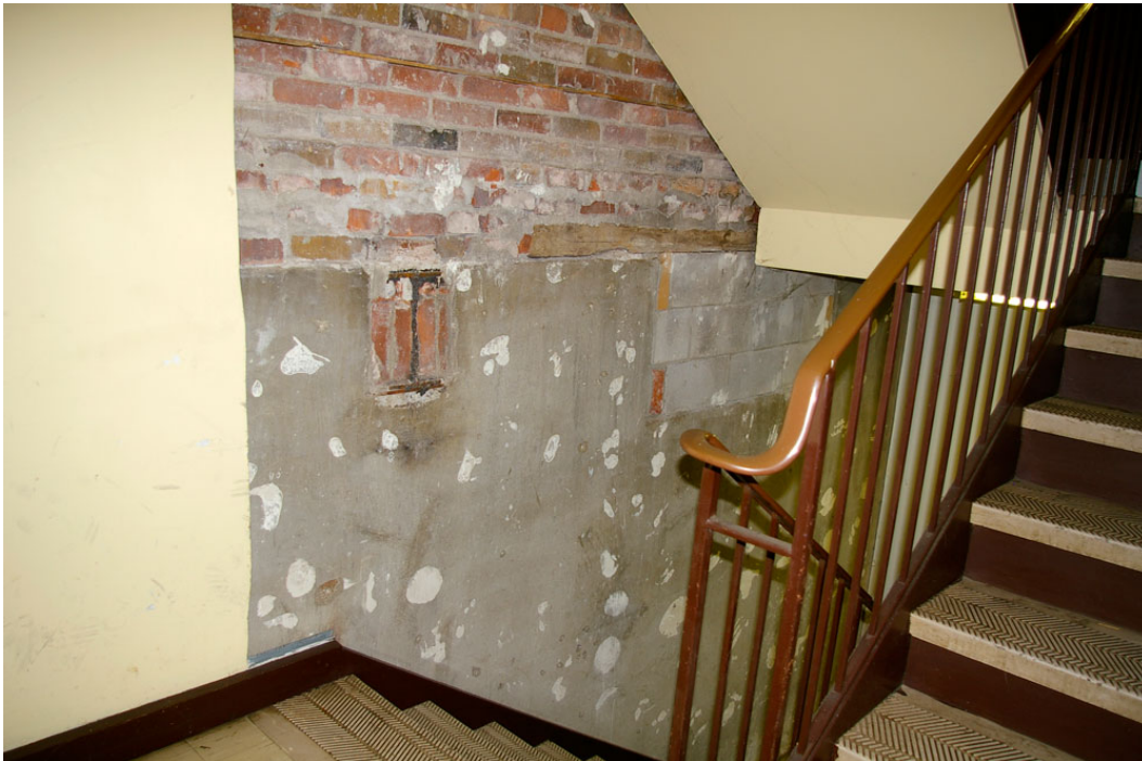
Photo 35: Rear stairwell on the landing between the ground floor and the basement, showing the concrete block construction of the foundation walls of the pre-1949 rear extension and a section of exposed double brick masonry wall above.
