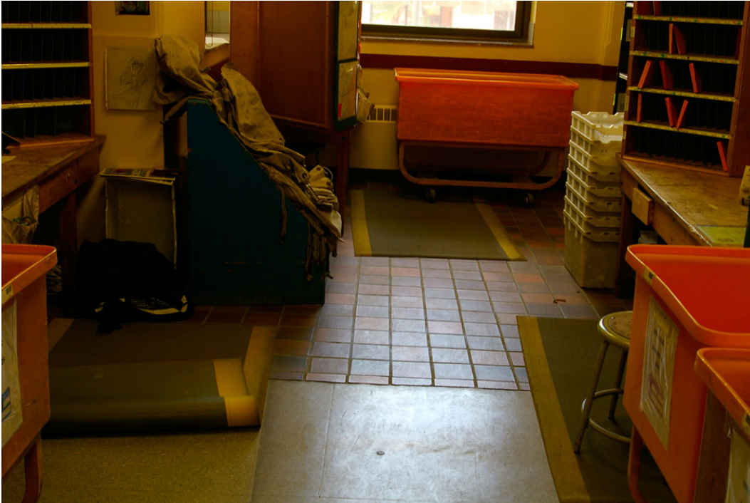
Photo 44: Close-up view of the above photograph showing the glazed terra cotta tile laid in the Public Lobby and the two enclosed entrance vestibules, as part of the 1979 renovations. This tile ended in front of the counter and abutting it is a section of what appears to be original sheet linoleum flooring which still covers a portion of the working area on the ground floor.
