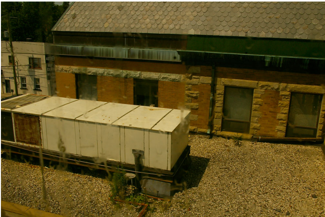
Photo 26: View of the tar and gravel roof of the one storey section as enlarged by the pre-1949 rear extension with the air handling unit installed in 1979. Also shows the copper fascia and eavestroughing (relined with pre-finished galvanized iron) of the original building and the shallower copper fascia and eavestroughing of the 1979 addition. Photo taken through a dirty window on the third floor of the west facade of the east wing looking south-west towards McMurray Street.
