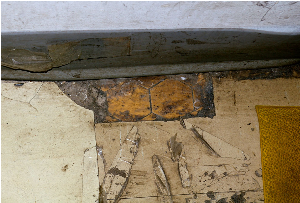
Photo 45: A small area of hexagonal tile floor exposed beneath old linoleum flooring near the back corner of a north-south partition wall to the left of the original front counter which was moved forward in 1960.
