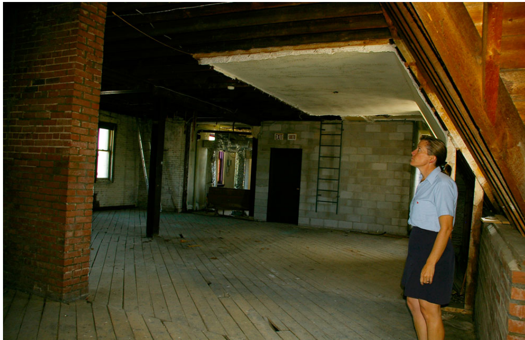
Photo 63: Part of the unfinished area of the third floor and the south-facing bedroom of the caretaker's suite (delineated by the plaster ceiling) looking north-east towards the 1979 stairwell addition, the north-east corner of the clock tower (with the steel ladder) and the east window of the frontispiece (originally in the open stairwell with the wood staircase, as shown on the 1911 Third Floor Plan (No. 4: Figure 21 )).
