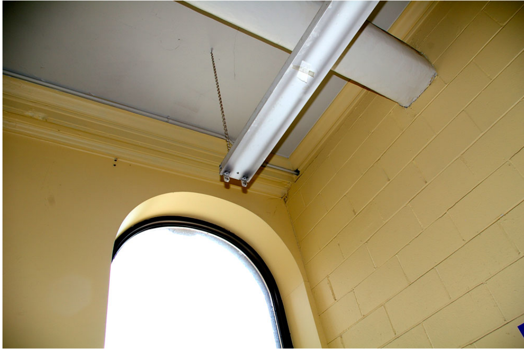
Photo 42: Detail of the original wood cove between the outer wall and the ceiling, which is now only visible in the Mail Room. View of the north-west corner with an original arched window opening on the west facade. The interior concrete block partition wall separates the Mail Lobby from the Vault room.
