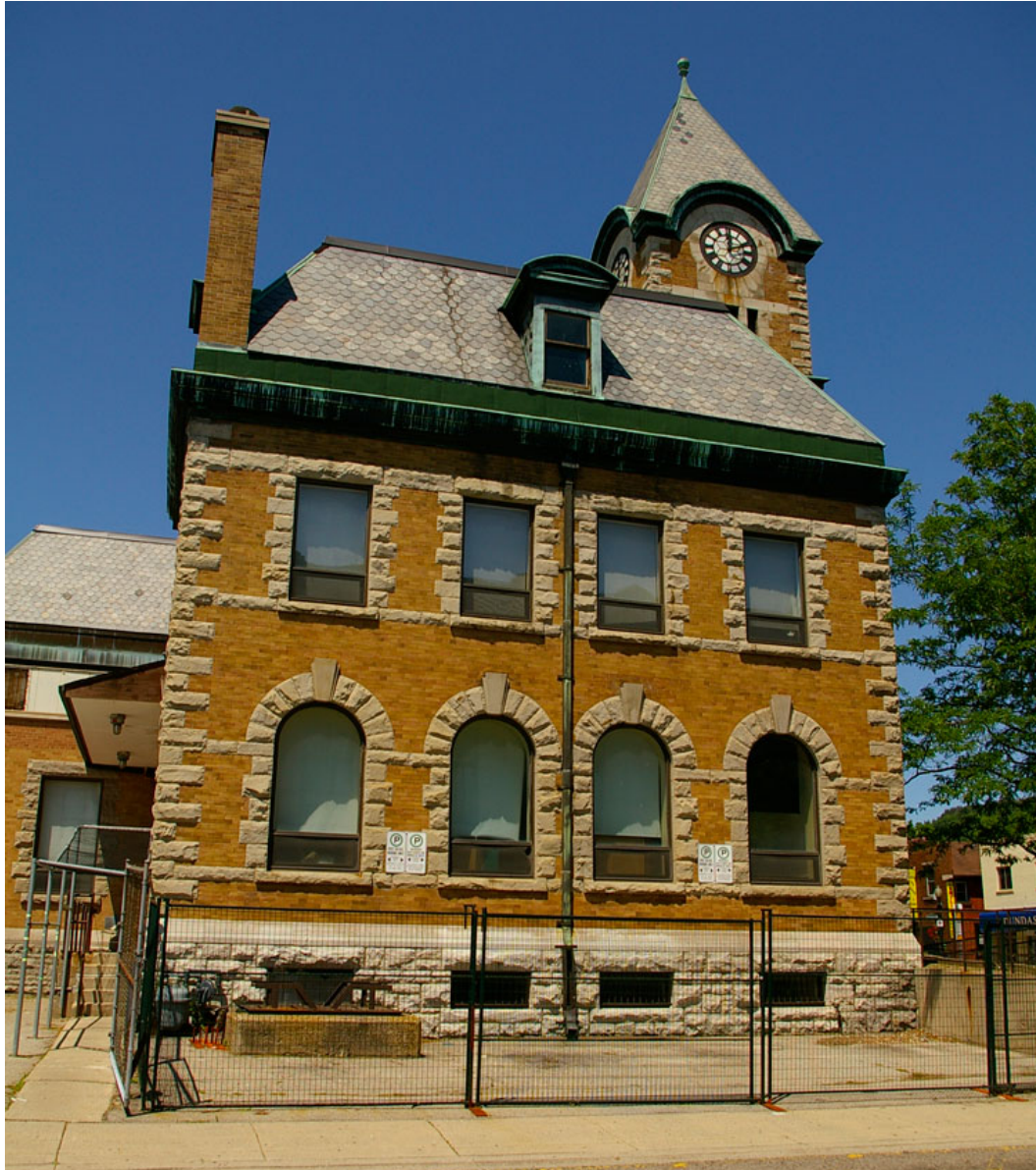
Photo 11: East facade of the building, showing the steps to the original concrete loading platform, and one of the two east-facing windows of the pre-1949 rear extension. Alterations and additions dating back to 1979 include the replacement windows on the first and second storeys and the cantilevered shed roof over the rear platform. Also shows the original concrete coal chute with its iron lid and a window opening behind (blocked up from inside) above a doorway in the basement, which provided access to the chute.
