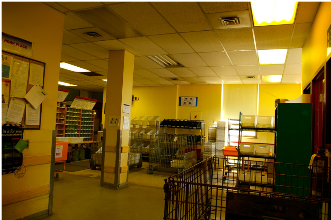
Photo 39: South-east corner of the pre-1949 rear extension looking east through one of the two east-facing windows. Shows the column and wall section marking the location of the rear wall of the original building. The flooring in this area appears to be the original sheet linoleum laid when the addition was built. Shows a variety of shelves and bins used to sort and move mail within the building.
