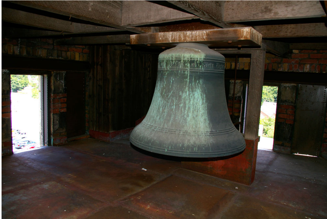
Photo 76: Fifth floor housing the bell. Shows the galvanized-iron panels covering the floor structure, which was intended to deflect the sound of the bell away from the floors below and out the openings.
