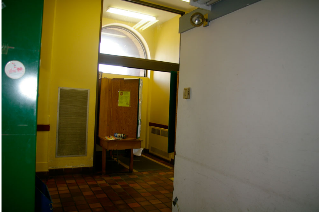
Photo 48: View from beside the west partition wall towards the main entrance facing King Street. The doorway has been blocked up in recent history with a drywall partition to create an additional letter sorting booth. The rooms to the left (original Mail Receiver Room) and right have also been sealed off from the former Public Lobby area. The doors of the inner vestibule, as rebuilt in aluminum and glass in 1979, were removed, likely when the letter sorting booth was created. The door frame and glass transom above were left intact.
