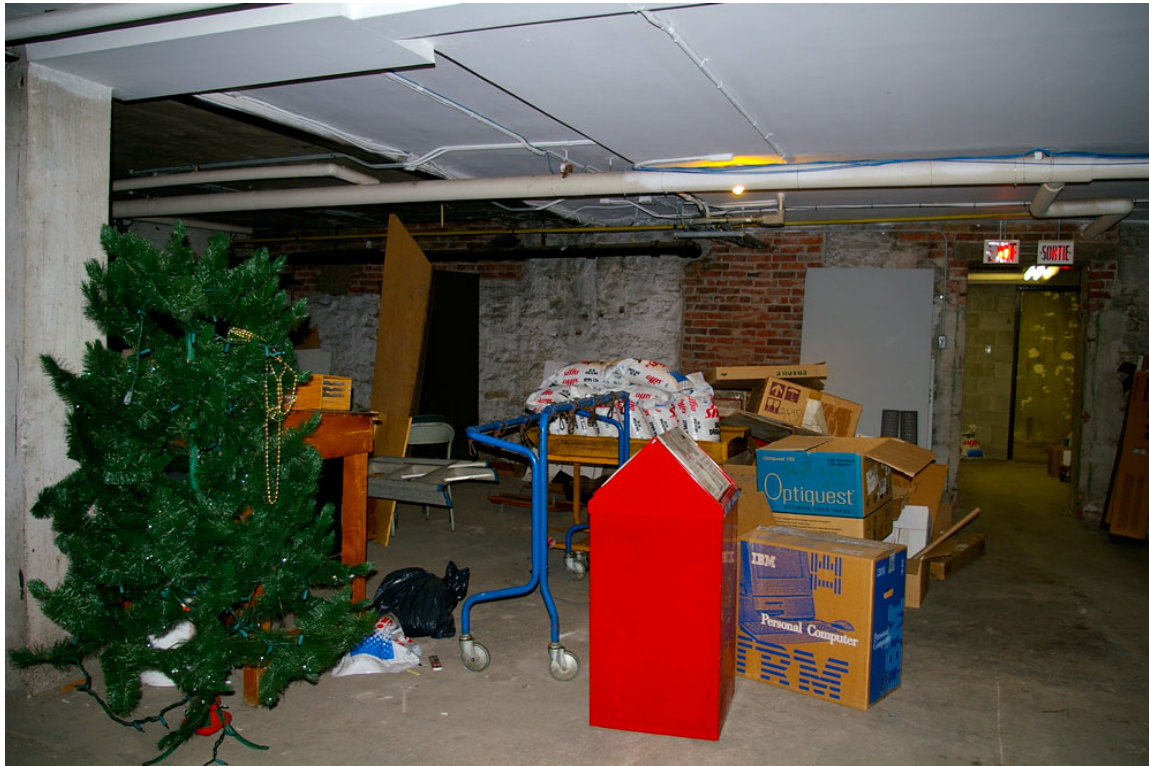
Photo 27: View looking south-east towards the original rear wall of the basement, constructed of rubblestone construction with some brick masonry infill. On the right is an opening leading into the pre-1949 rear extension and the doorway to the enclosed concrete block stairwell added in 1979. Flooring throughout both areas is poured concrete.
