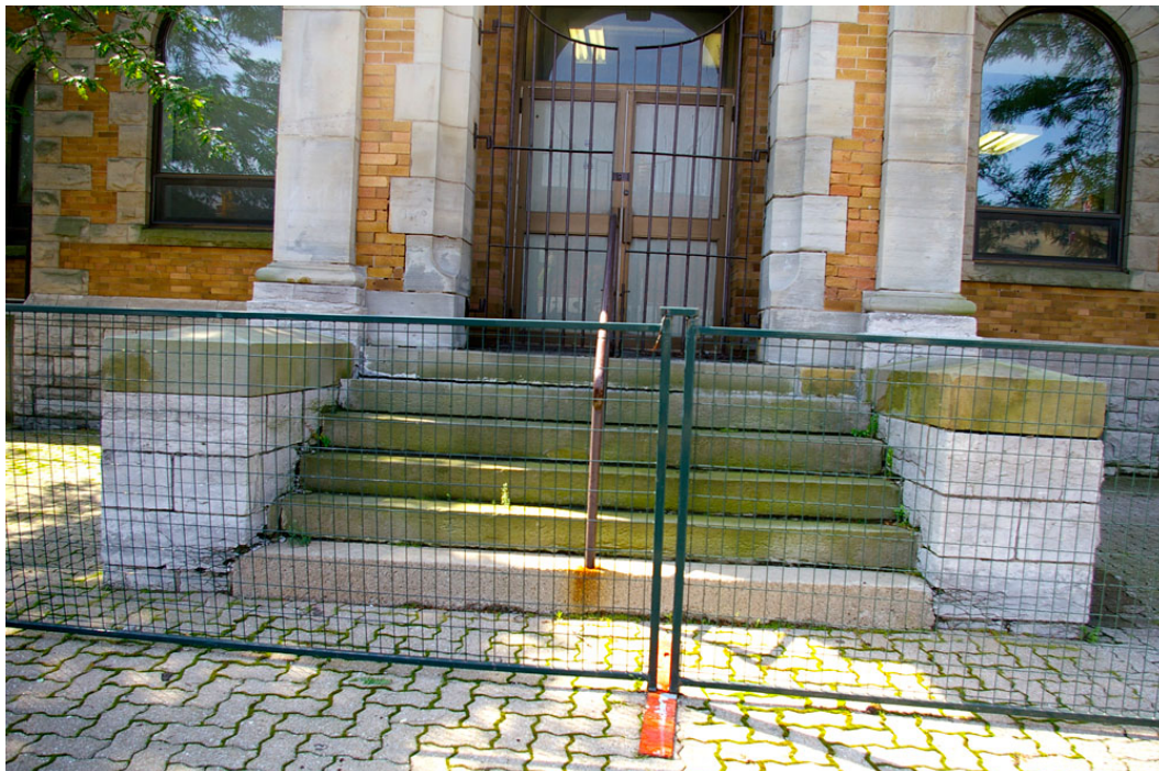
Photo 18: Close-up view of the front stairway with the low stone piers on either side of the stone/concrete steps, the metal safety railing erected for repairs undertaken in the mid-1990s and the metal security gates in the portico archway (date of installation unknown).
