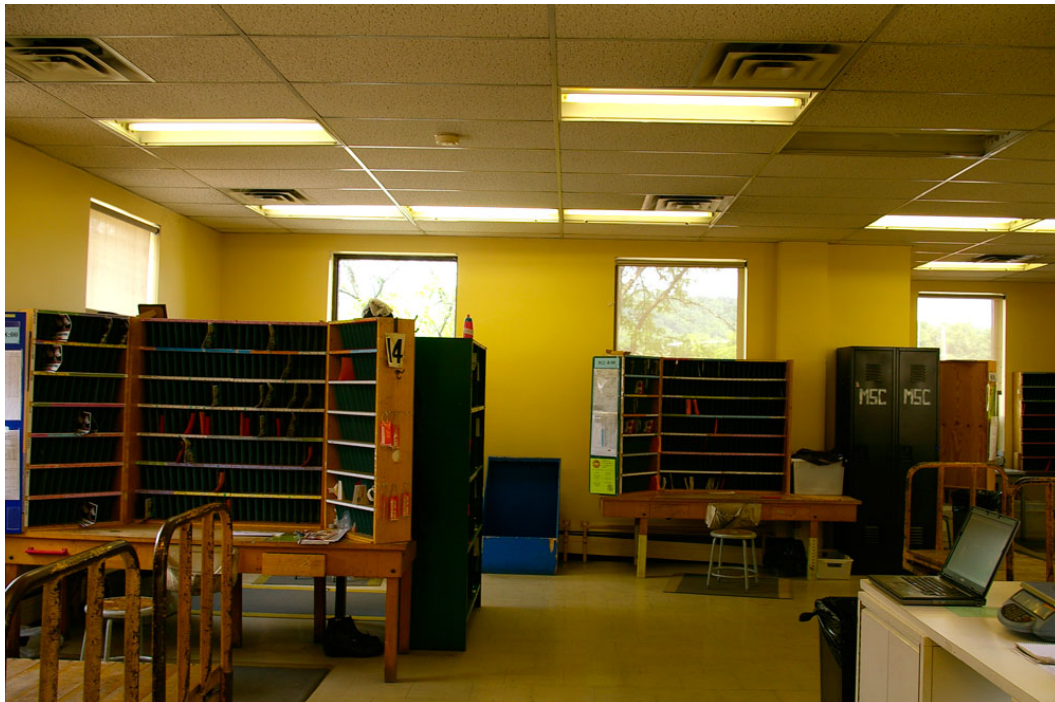
Photo 58: View of the north-west corner of the second floor looking directly north, with the west window of the frontispiece partially visible on the right. This and subsequent photos show the dropped panel ceiling installed in 1979. Many of the plexiglass panels which originally covered the recessed fluorescent lighting tubes have been removed.
