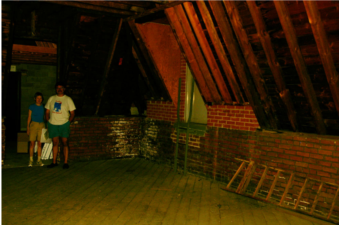
Photo 61: Unfinished area of the third floor looking south-west, with the author and Stan Nowak standing in front of the doorway to the 1979 addition. Visible beyond is the exposed concrete block wall and doorway of the rear stairwell. The short ladder and doorway leads to the mechanical room on top of the 1960 elevator shaft. Also shows the juncture of the framing for the mansard roof with the top of the brick masonry wall of the original building and newer brick masonry and roof alterations for the bridging section of the elevator shaft, as shown on the sections of the 1959 drawing showing the elevator addition (A-1: Figure 42 ). Lying on the floor is one of two remaining original wood ladders used to access the clock tower (replaced with steel ones).
