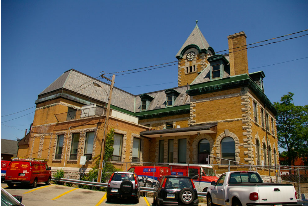
Photo 19: South facade looking north-west showing the one-storey pre-1949 extension and the 1979 second storey extension of the west wing.
