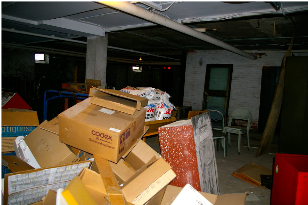
Photo 29: View of a large portion of the original basement looking north-east towards the front wall, showing a portion of the west wall of the boiler room (brick masonry construction) and the reinforced concrete column on the west side of the basement. The other three columns supporting the ground floor and back wall of the second floor are steel I-beams embedded in the east-west brick masonry wall of the boiler room, as shown on the 1911 Basement Floor Plan (Figure 18).
