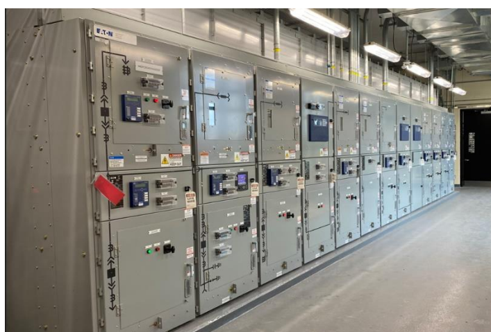
Figure 6: New control panels
