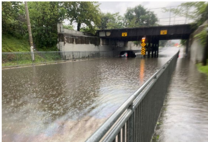
August 2023 storm – flooding on Birch Avenue
