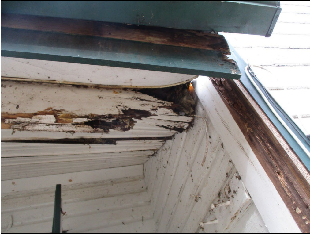
Figure 11: Detail View of damage to side porch
