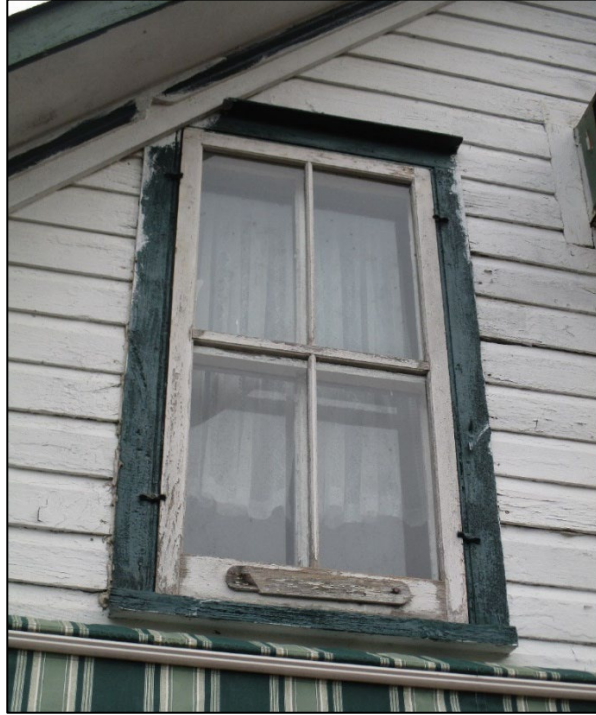
Figure 9: View of deterioration to wooden storm window
