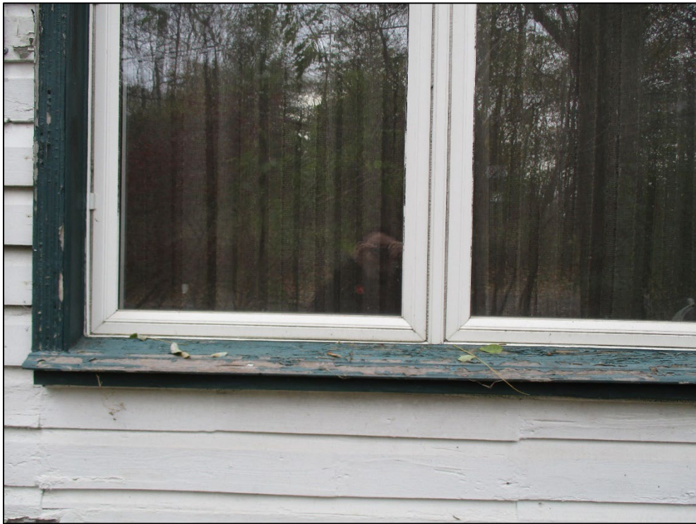
Figure 6: View of deteriorating window frames with contemporary replacement windows
