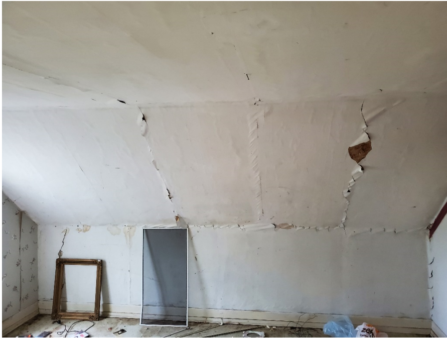
Photo No 01: 2 nd Floor North Wall above Kitchen
