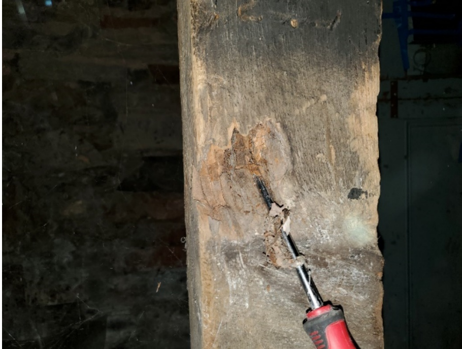
Photo No 09: Rotten Wood Knott
