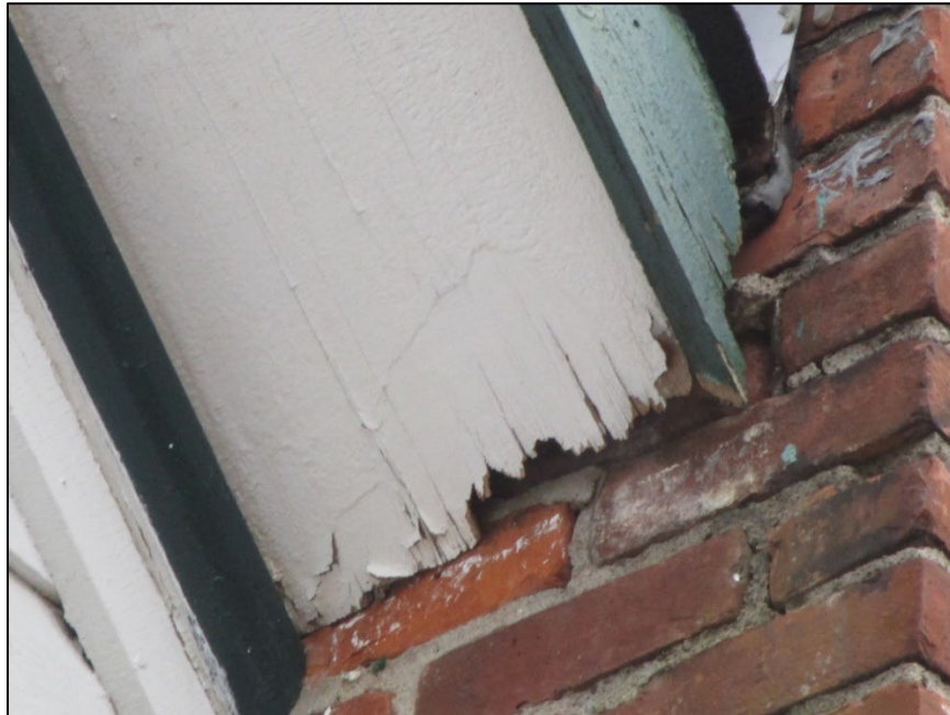
Figure 8: Detail View of damage to eaves
