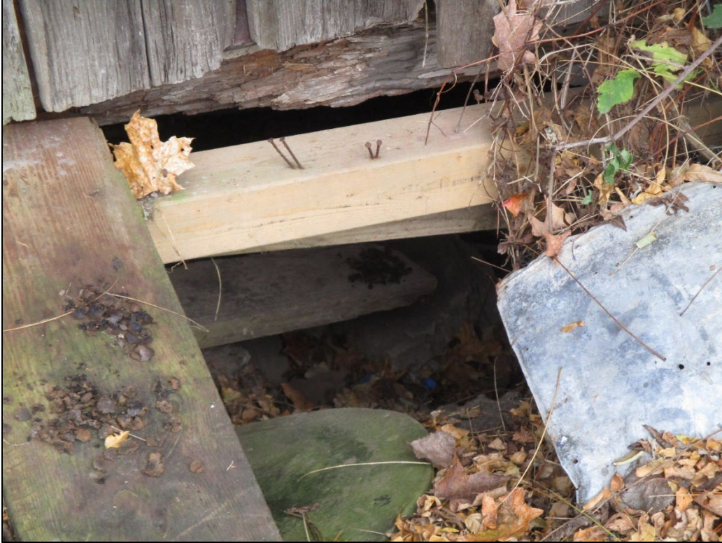
Figure 5: View of damage to shed foundation
