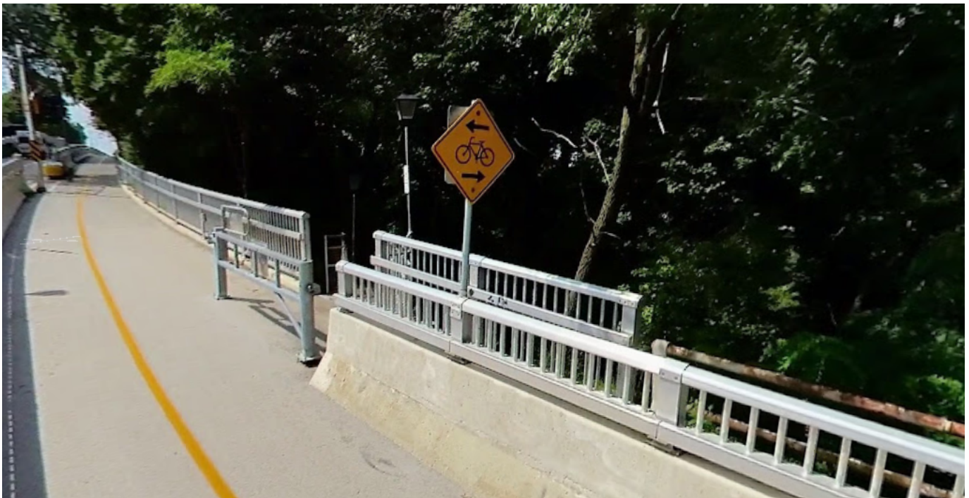
Photo by Smart Commute Hamilton. Top access of stairs shows vegetation covering lighting causing visibility issues.
