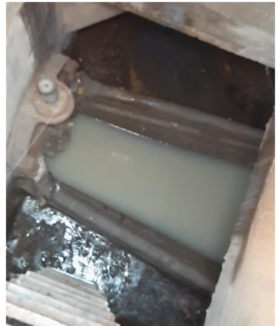
Sewer regulators in Hamilton's combined sewer system
