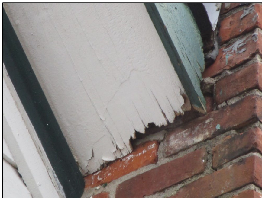
Figure 8: Detail View of damage to eaves
