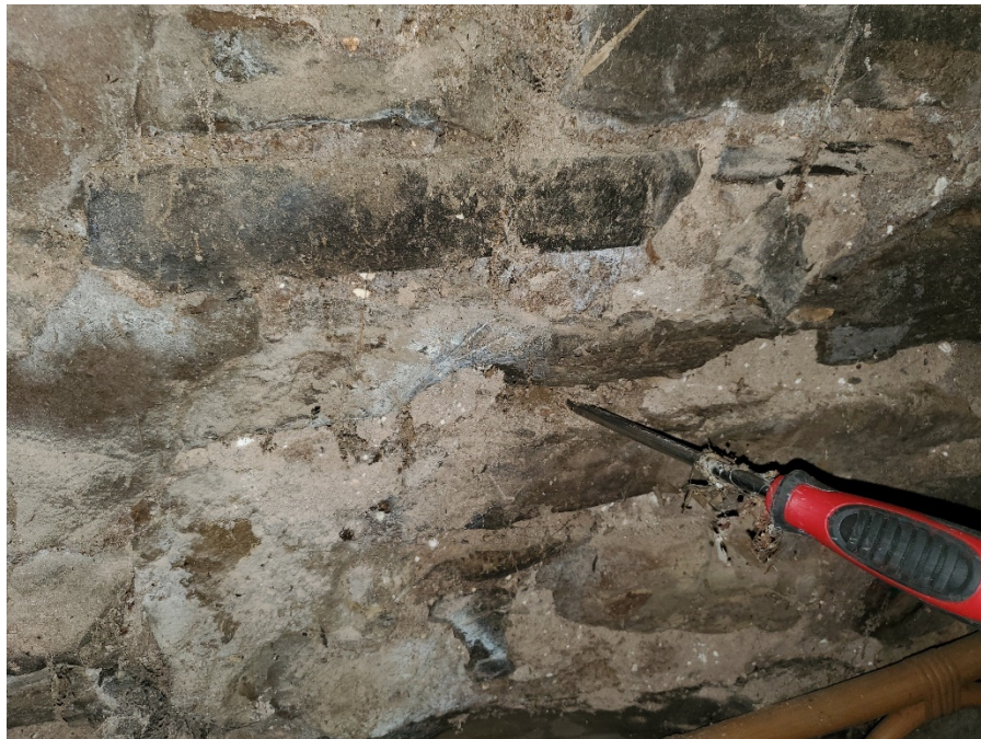
Photo No 10: Spalled Mortar Joint
