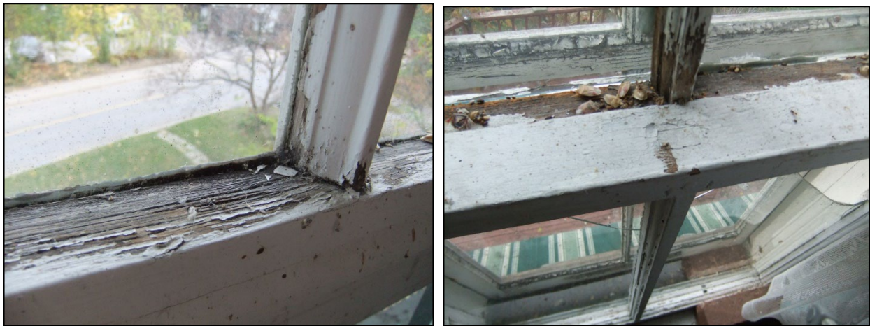
Figure 16: View of deterioration of upper-storey wood windows
