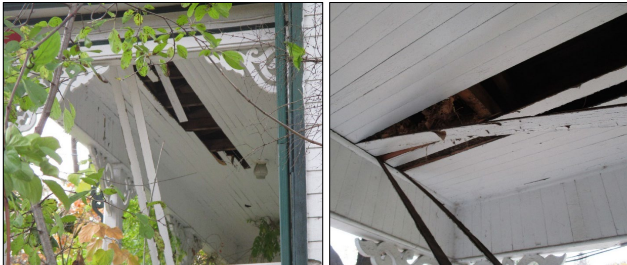
Figure 7: Views of damage to front porch ceiling
