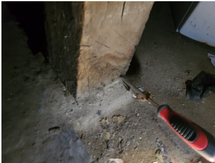
Photo No 08: Rotted Post Base
