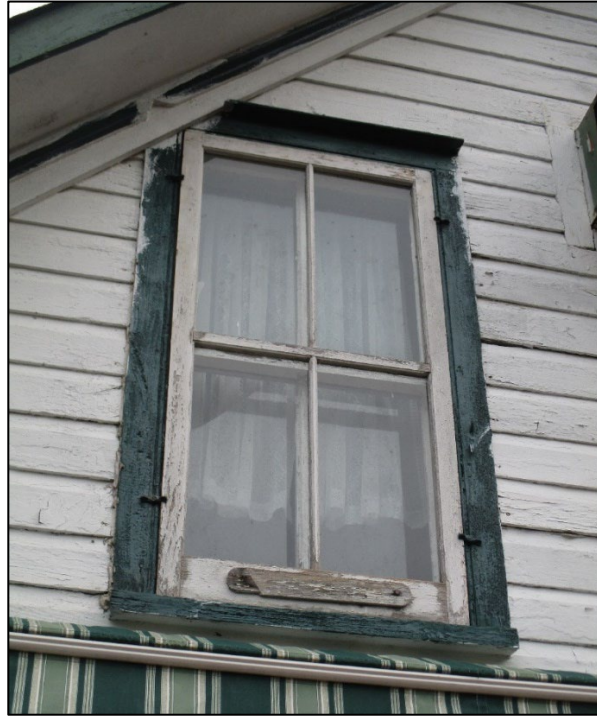
Figure 9: View of deterioration to wooden storm window
