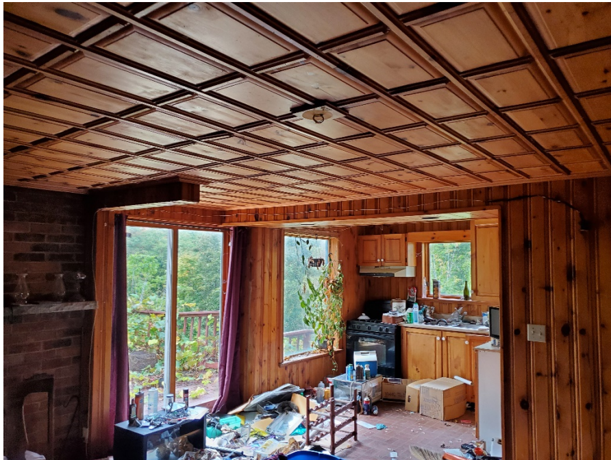
Photo No 02: North Kitchen Wall below Photo No:01
