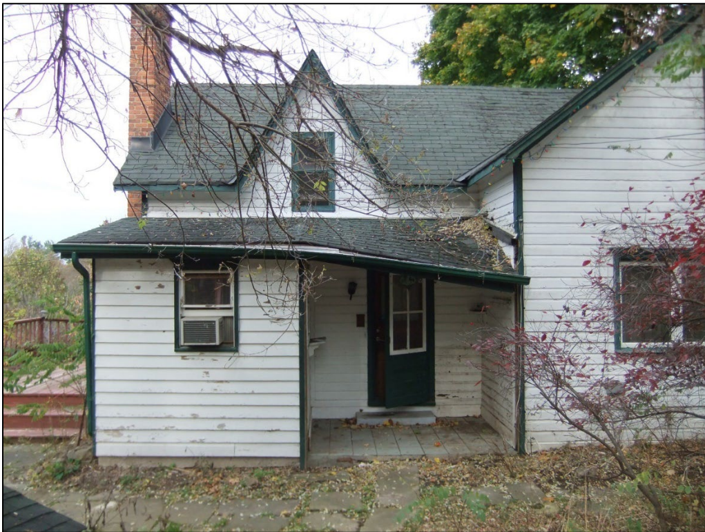
Figure 10: View of South Exterior and partially-collapsed side porch
