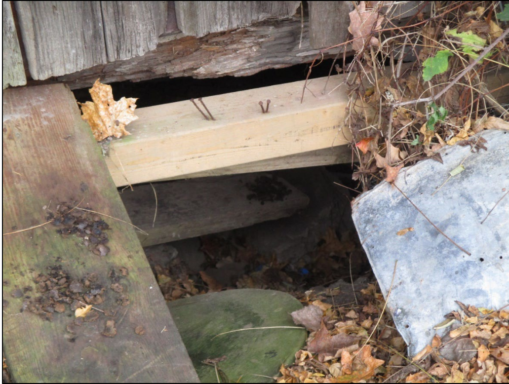
Figure 5: View of damage to shed foundation
