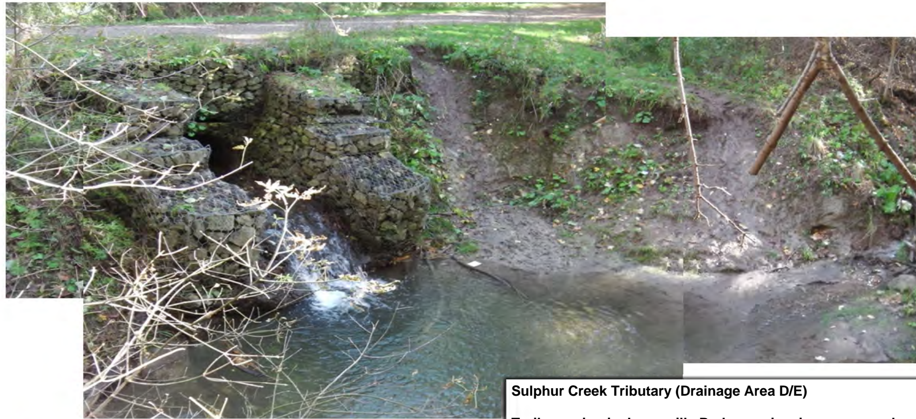
Sulphur Creek Tributary (Drainage Area F) Outfall from existing SWM Pond elevated with bed incision on downstream side to foundation invert.
