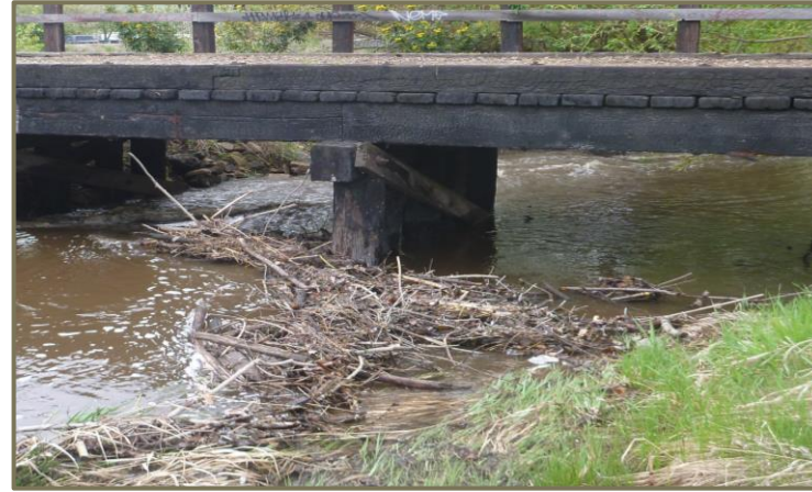
Debris in Creeks
