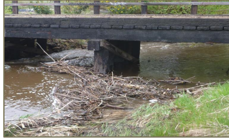
Debris in Creeks
