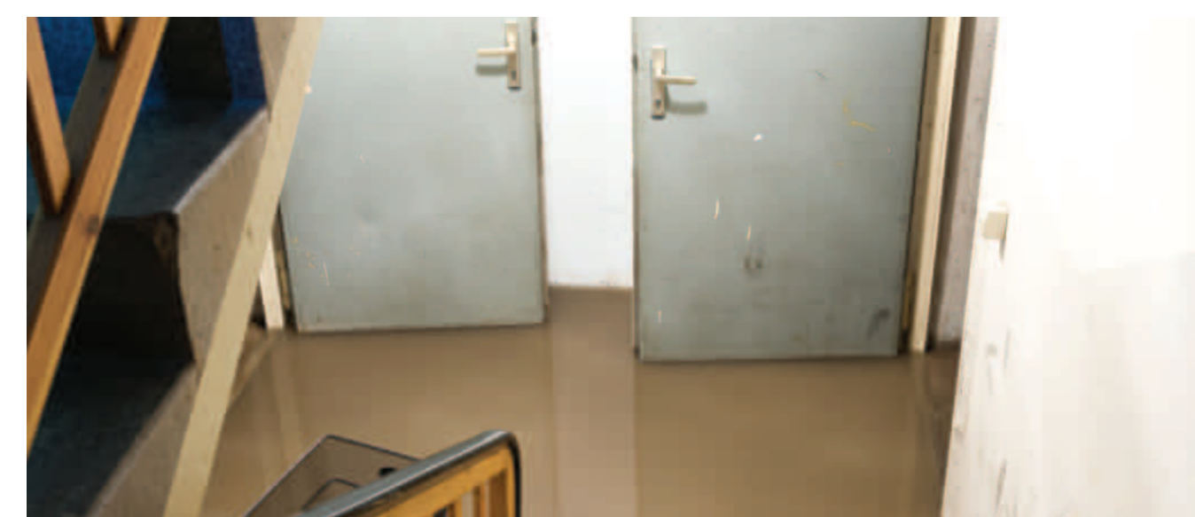
System Surcharge/Basement Flooding
