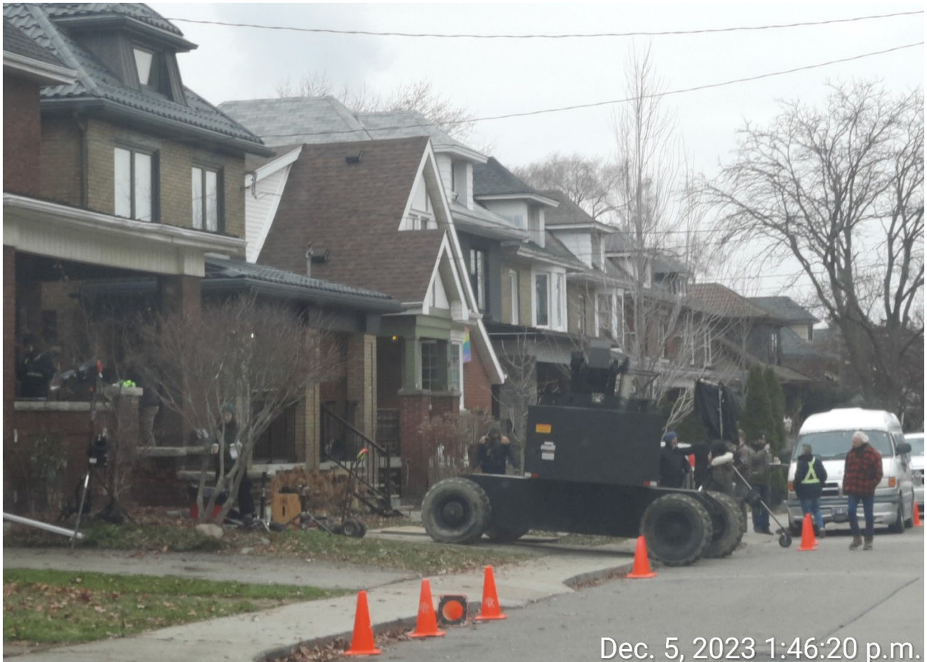
PRODUCTION EQUIPMENT BLOCKING THE SIDEWALK No Occupancy Permit
