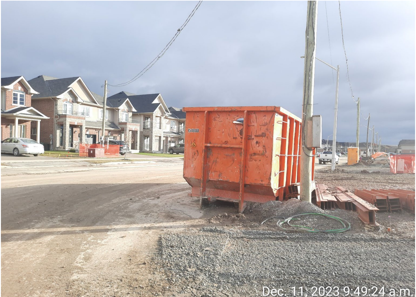
CONTRACTOR'S BIN ON THE ROAD WITHOUT A PERMIT AND CAUSING A SIGHTLINE ISSUE FOR MOTORISTS
