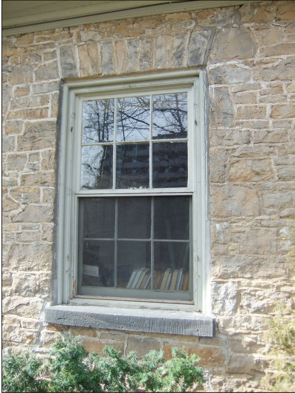
Image 6: Image of a six over six sash window on the dwelling's eastern elevation.
