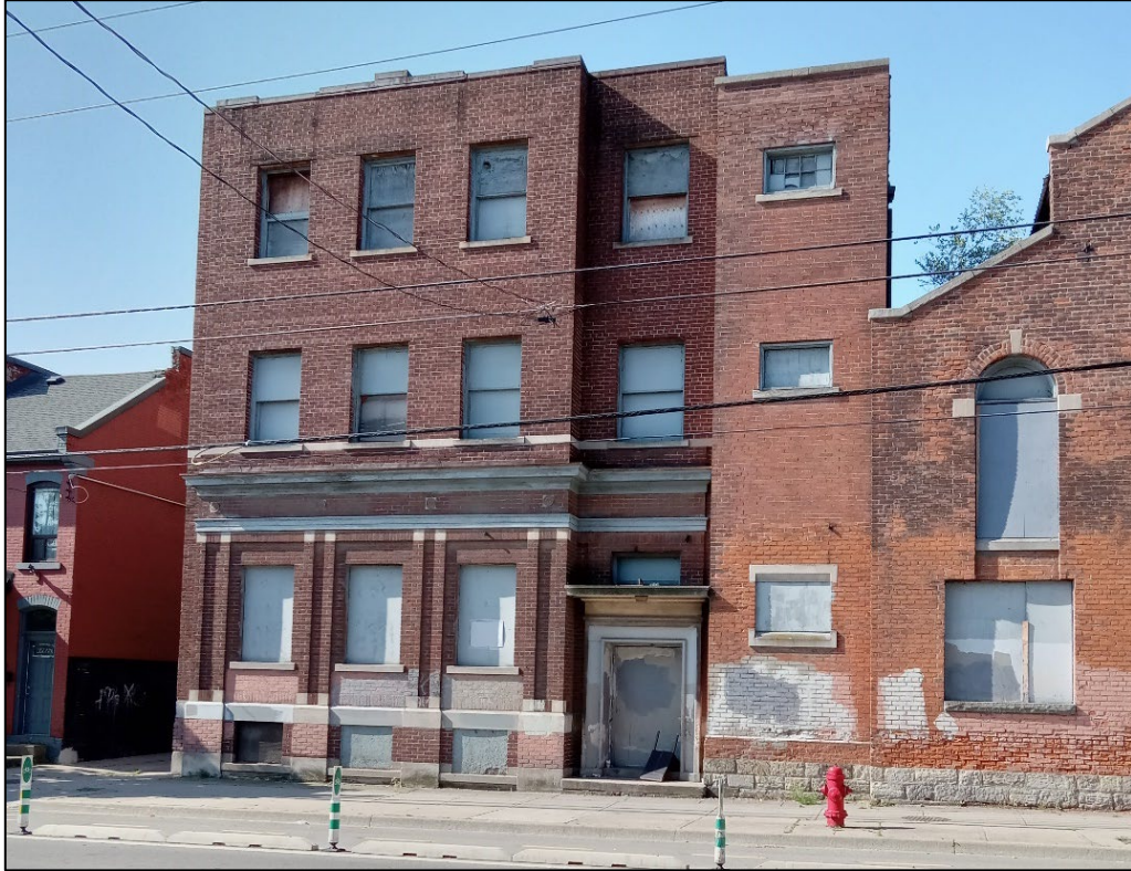
Figure 3: View of the front (north) elevation of 134 Cannon Street East (Structure 5) built circa 1920.
