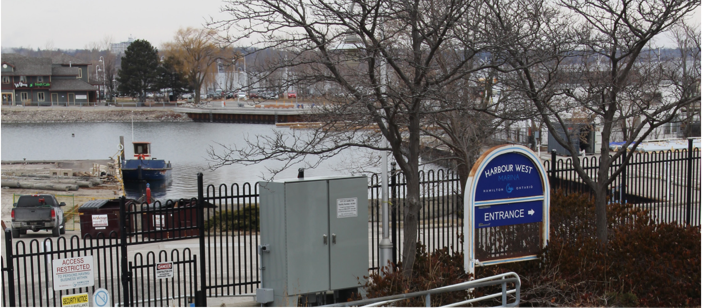
James Street North Combined Sewer Overflow Tank. PHOTO City of Hamilton.
