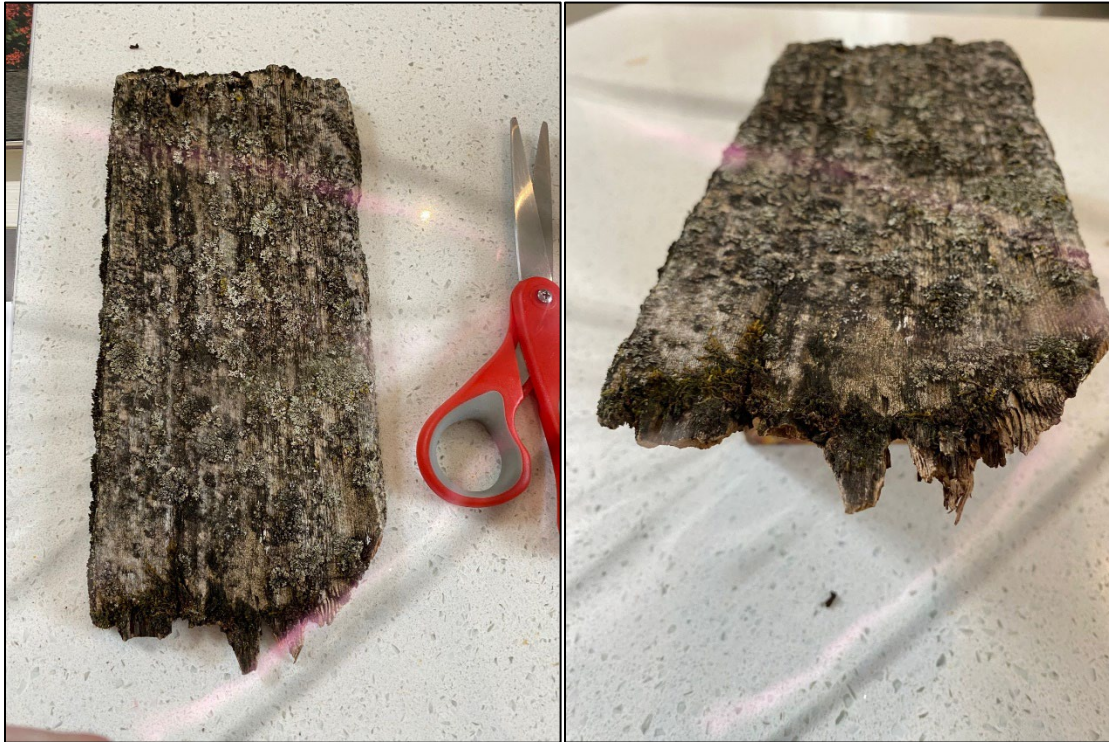
Figure 6: Existing roof shingle that blew off of home during high winds – shows level of deterioration.
