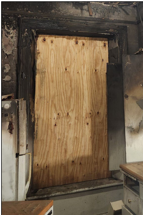
Figure 5: View from interior of one window to be replaced, due to damage from the fire.
