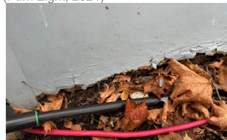
Painted particle wood siding with matching painted corner caps being rotted at grade (Park Eight, 2024)
