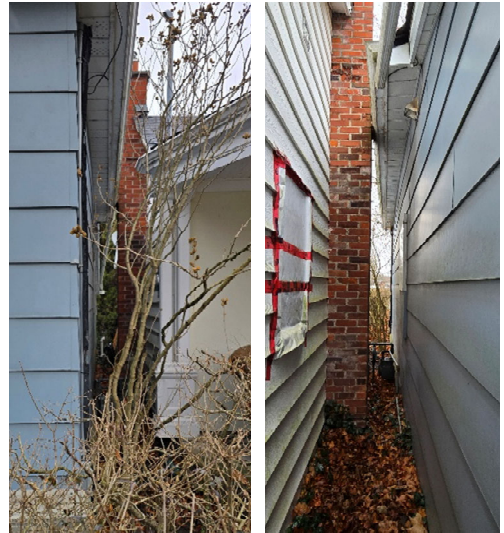
Side elevation photos LEFT photo facing north between bldgs. RIGHT photo facing south between bldgs. Note that ex 191 Melville eaves trough is touching neighboring dwelling (Owner, 2024)
