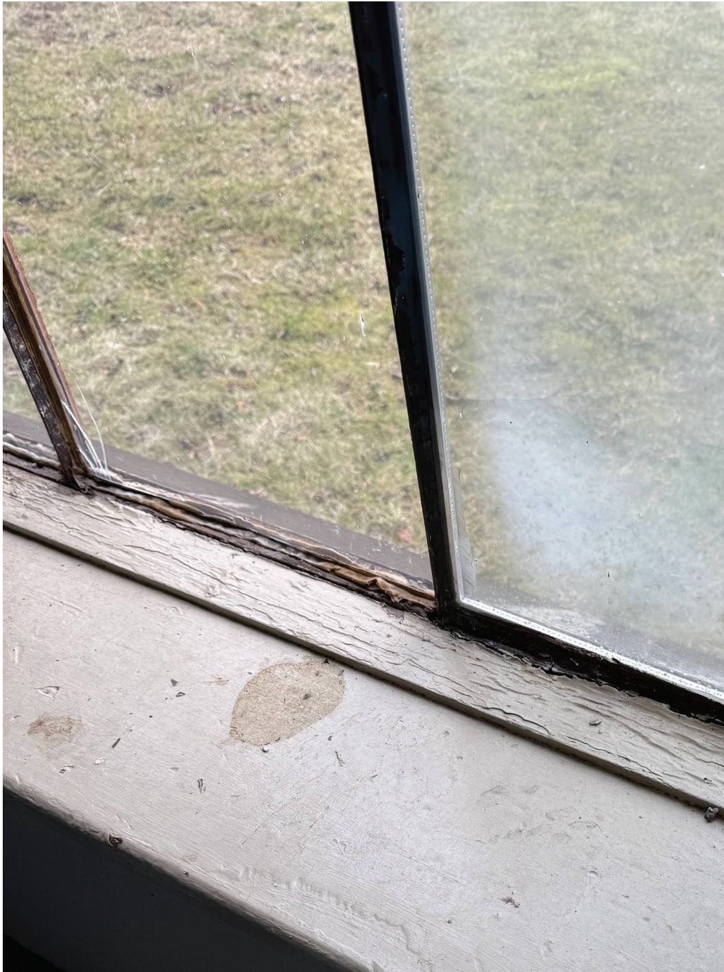
Figure 6 – Existing corroded steel window frame with cracked glass, and water damaged wood window sill.
