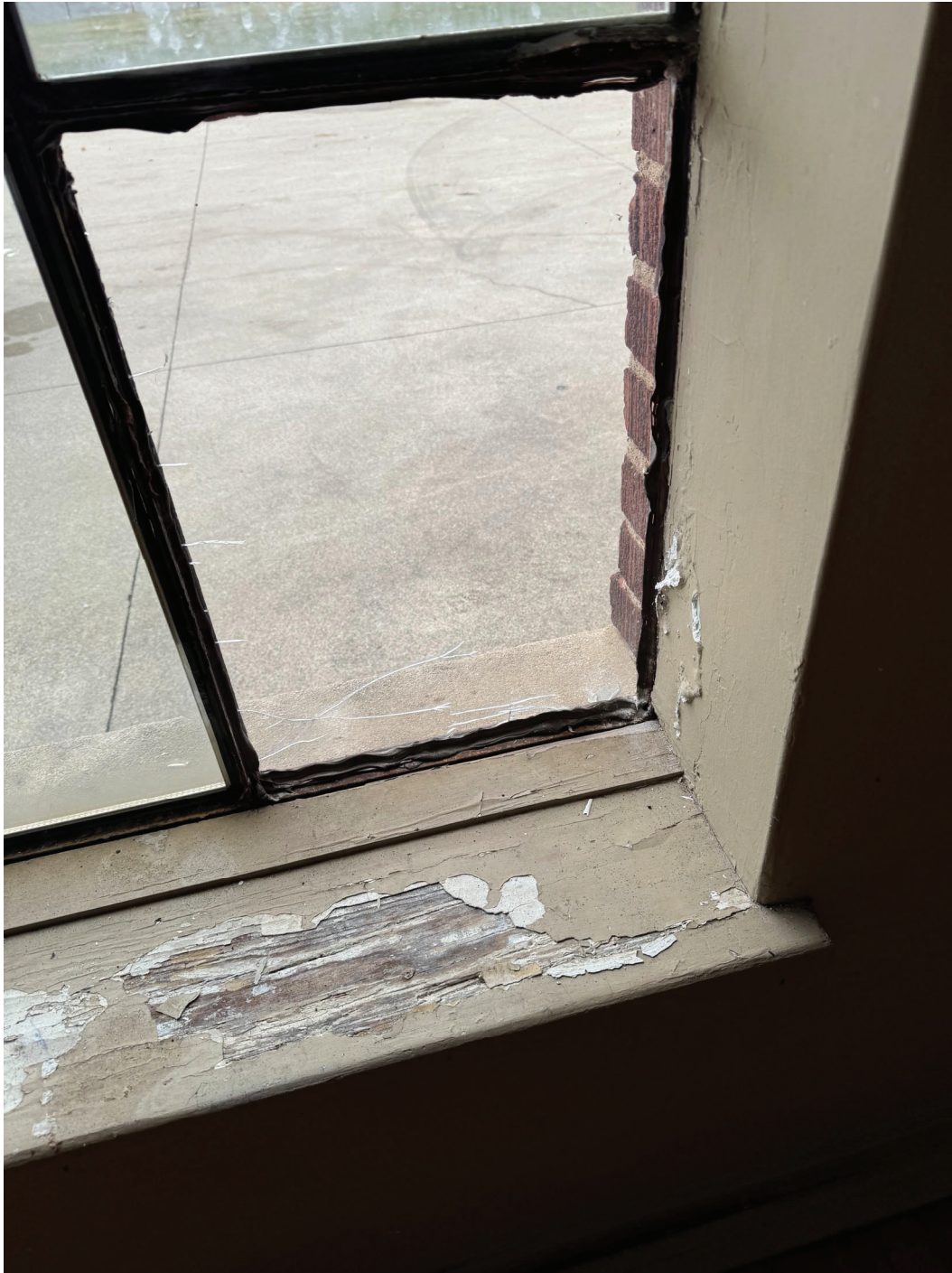
Figure 3 – Existing corroded steel window frame patched with caulking, cracked glass, and water-damaged wood window sill.
