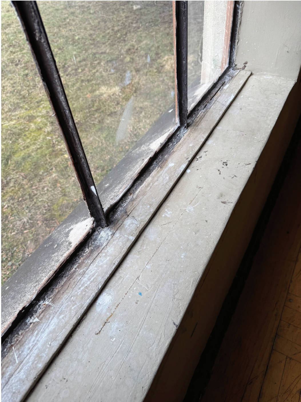
Figure 1 – Existing corroded steel window frame
