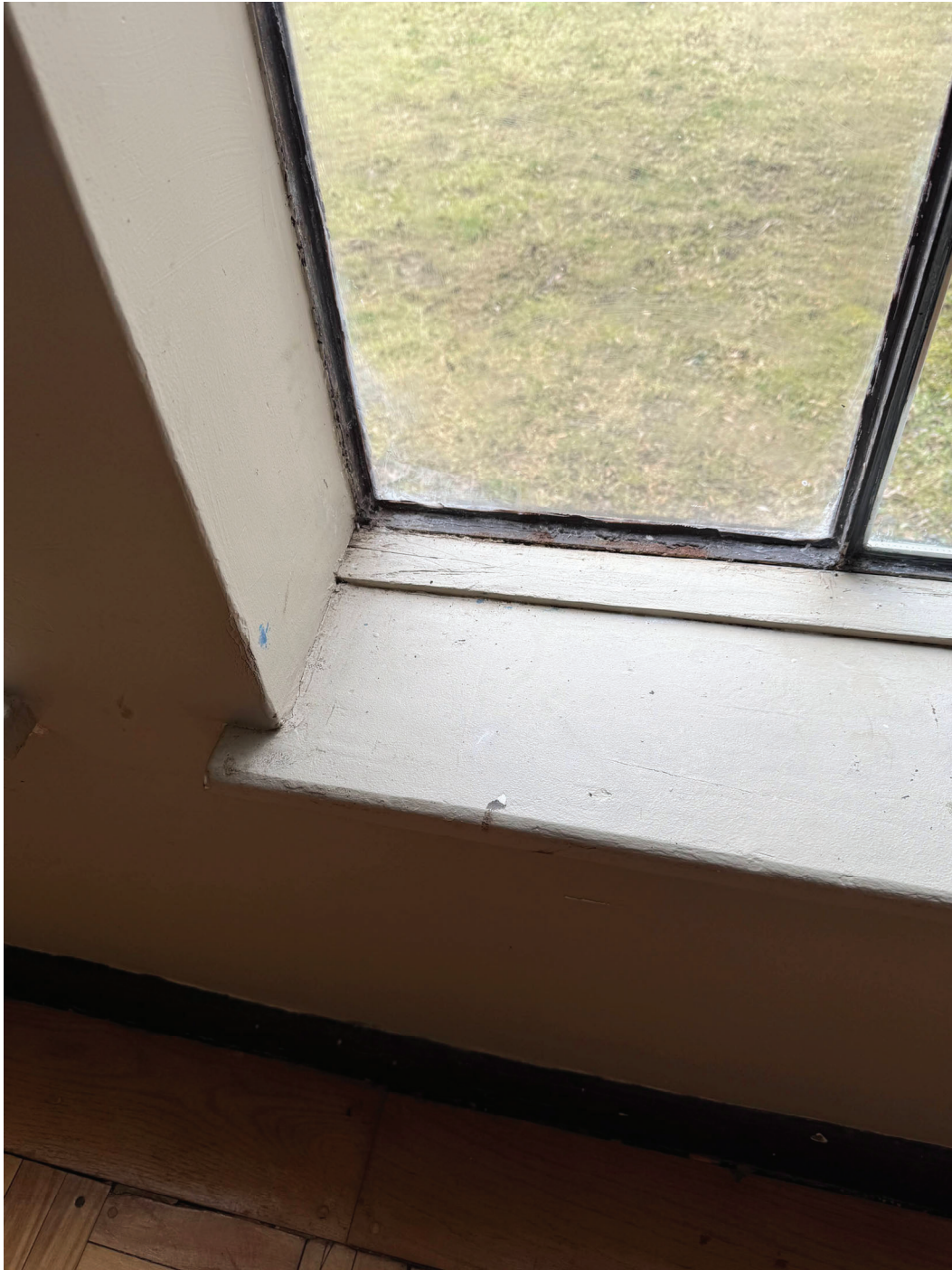
Figure 2 – Existing rusted steel window frame
