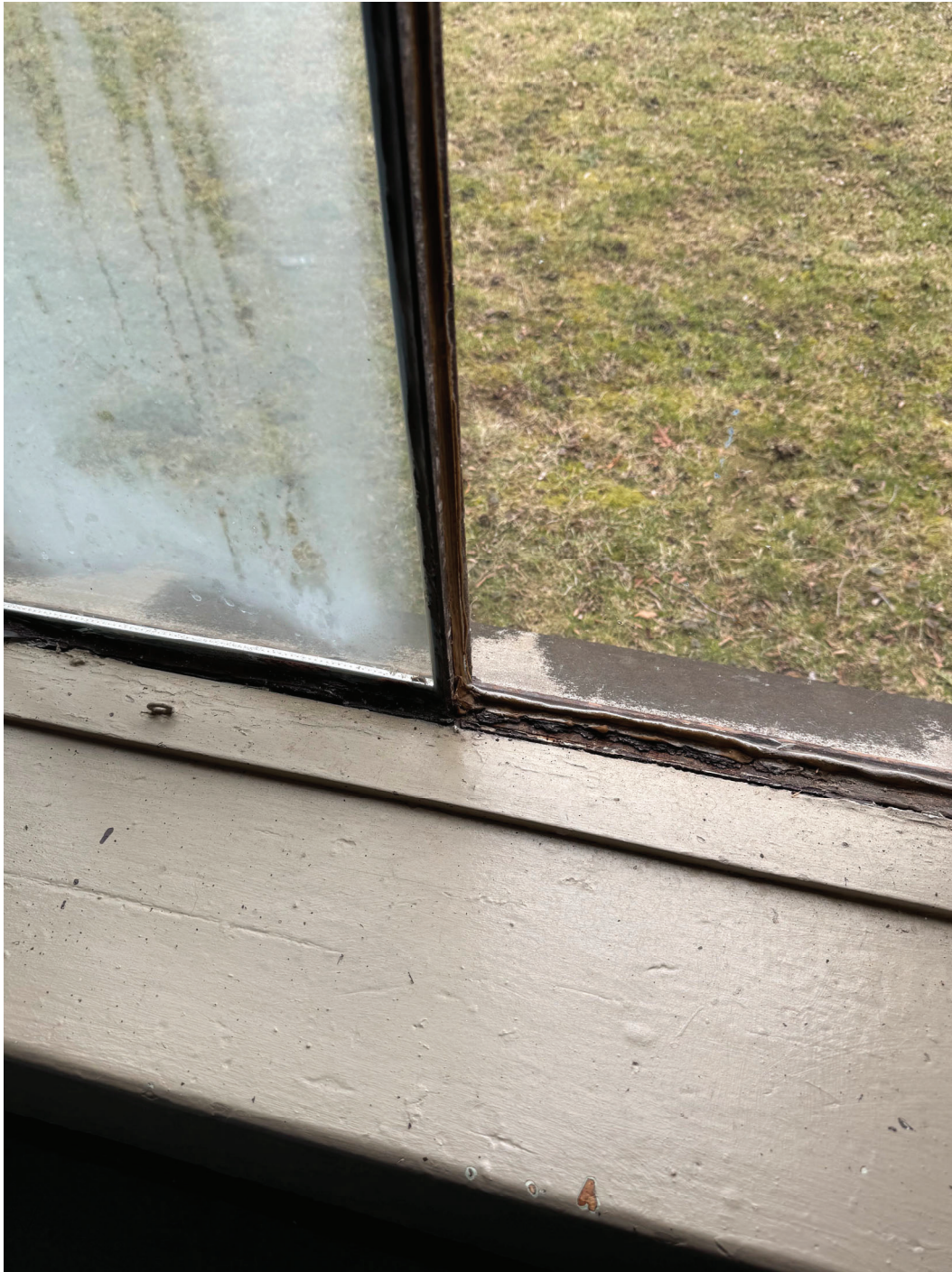
Figure 5 – Existing corroded steel window frame.
