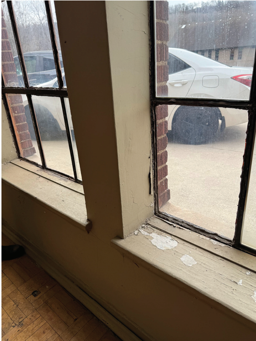
Figure 4 – Existing corroded steel window frame patched with caulking, and water damaged wood window sill.
