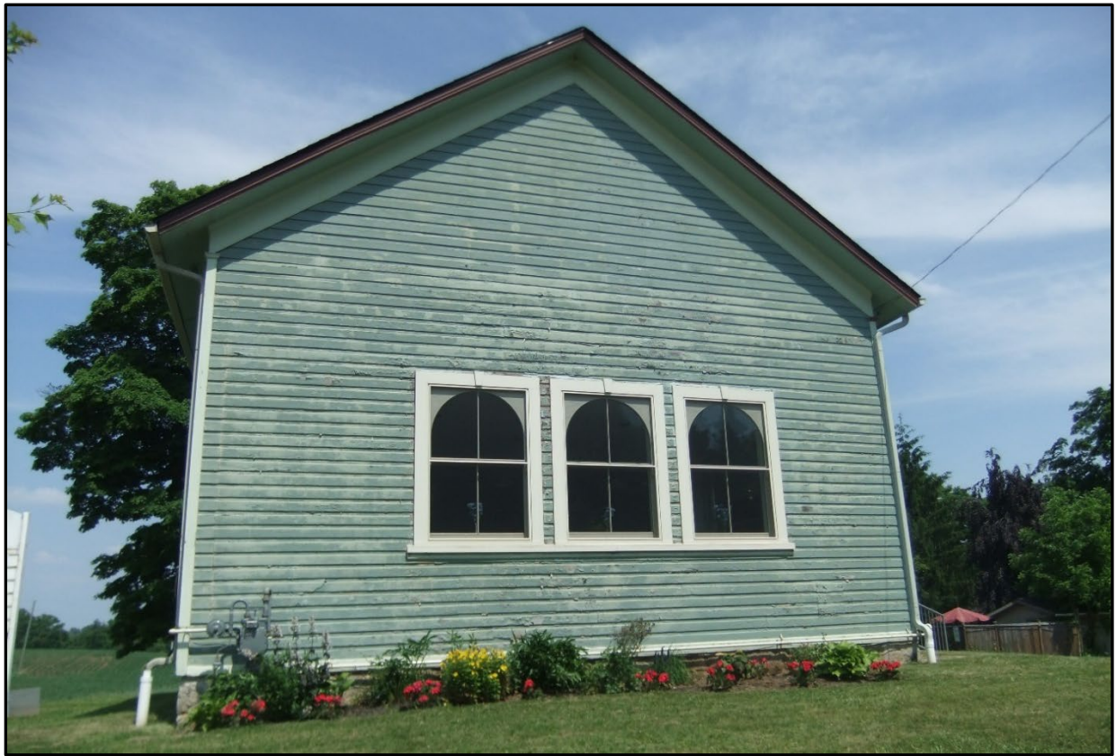
Figure 2: Side (west) elevation of 2295 Troy Road showing the deteriorated wood siding and side gable roof (Site Visit, 2024)
