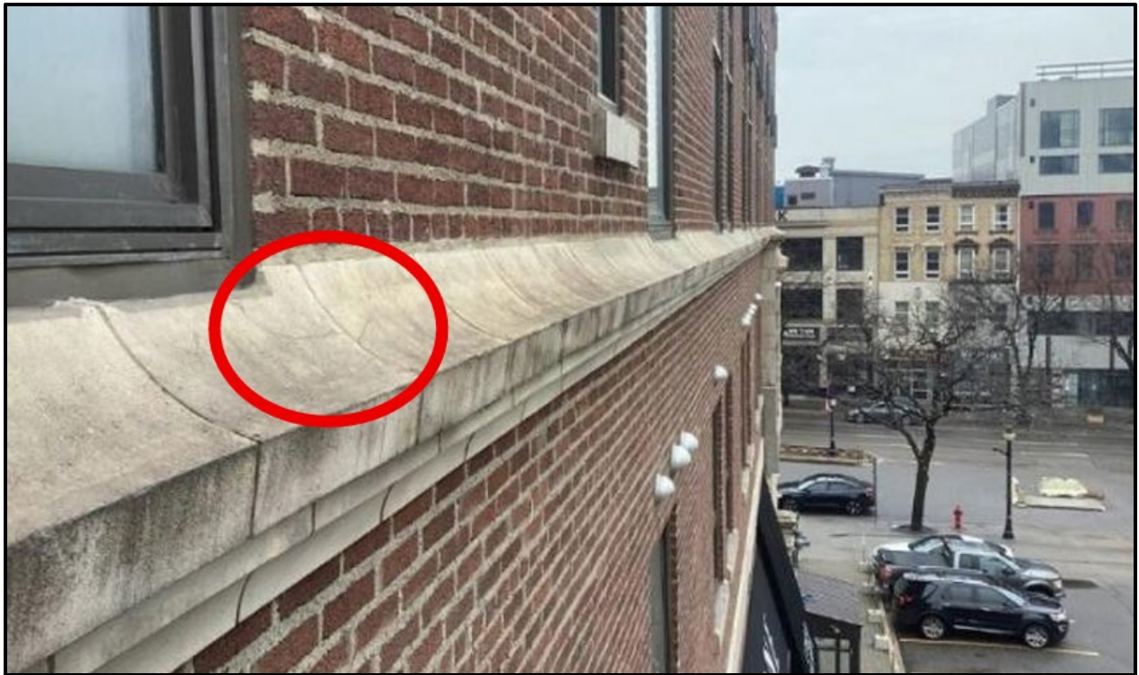
Figure 5: Close up example of a cracked cast stone in need of repair along the east elevation (Proponent Submission, 2026)
