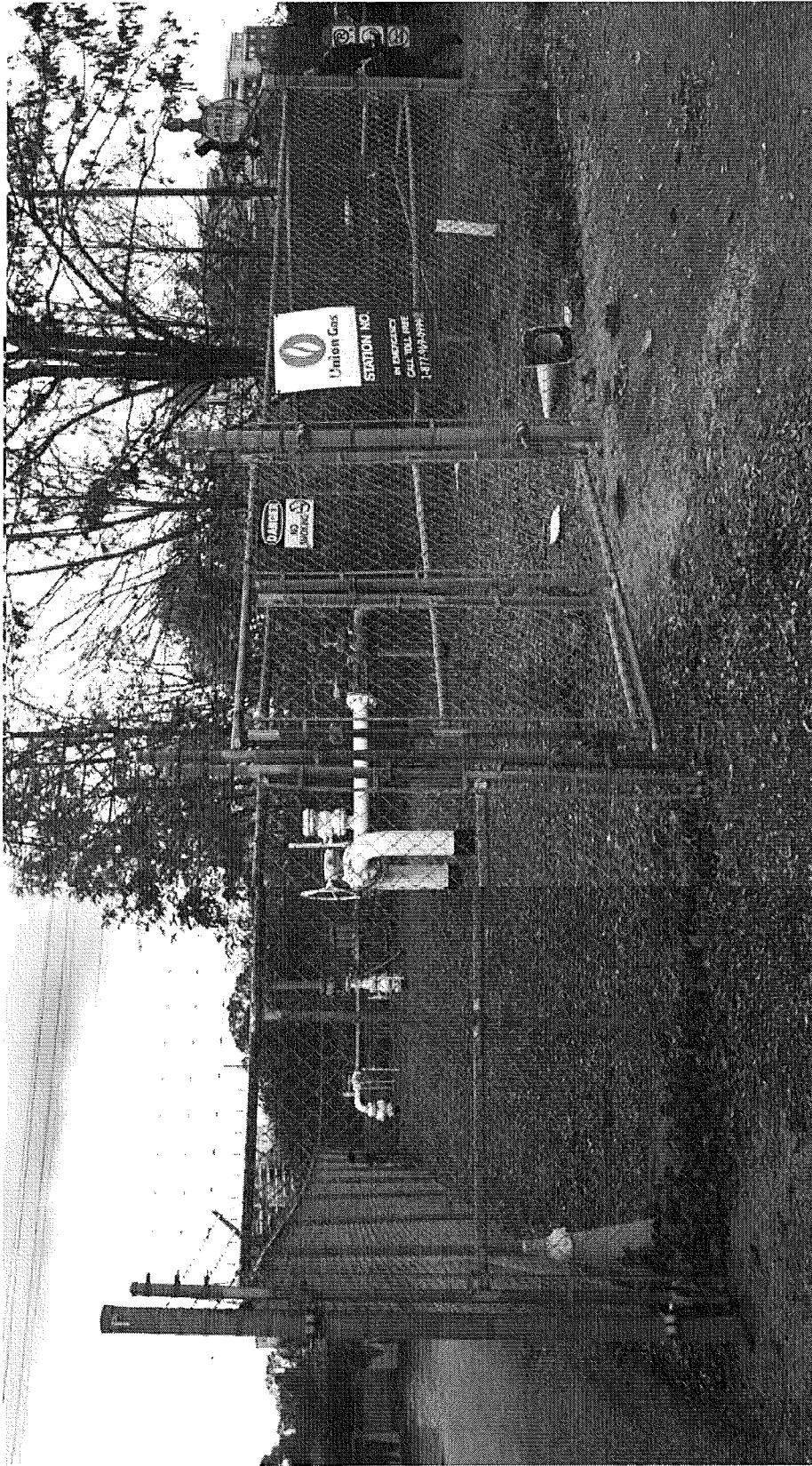
Union Gas Valve Station
