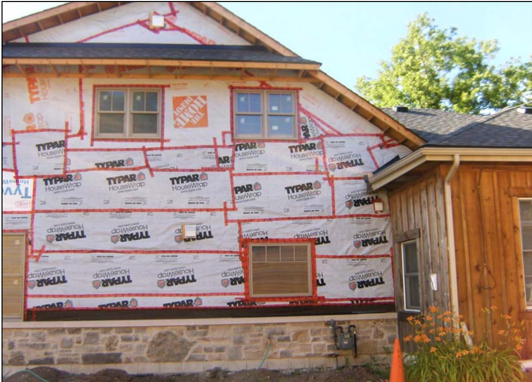
South side of the new addition, with stone cladding along the foundation
