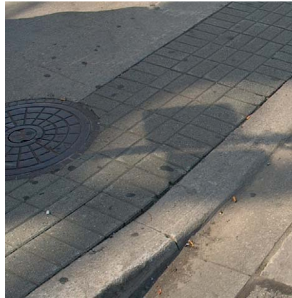
Photo 5.21: Curb ramps should be provided at all intersections. Textured paving also assists those with visual impairments.
