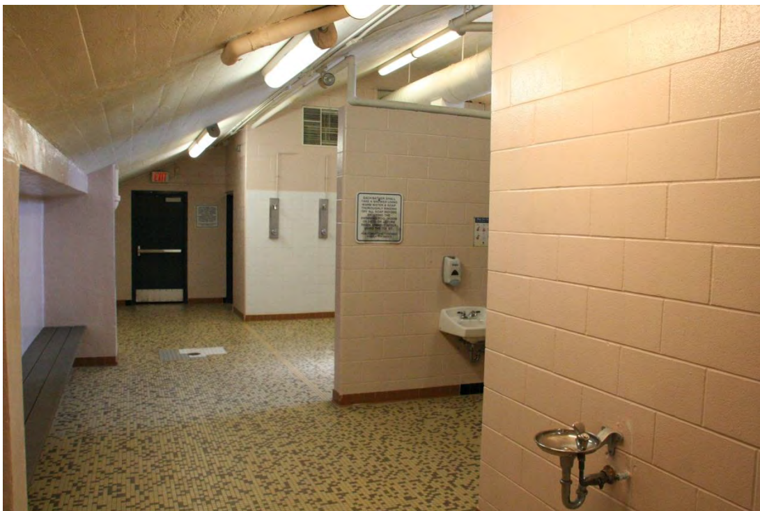
Figure 23: Men's change room looking north showing slope of pool bleachers in ceiling
