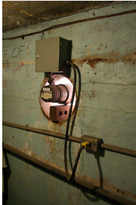
Figure 24: Storage room showing one of the pool's light fixtures on the north end of the pool. The marks of the board forms in the concrete are visible.
