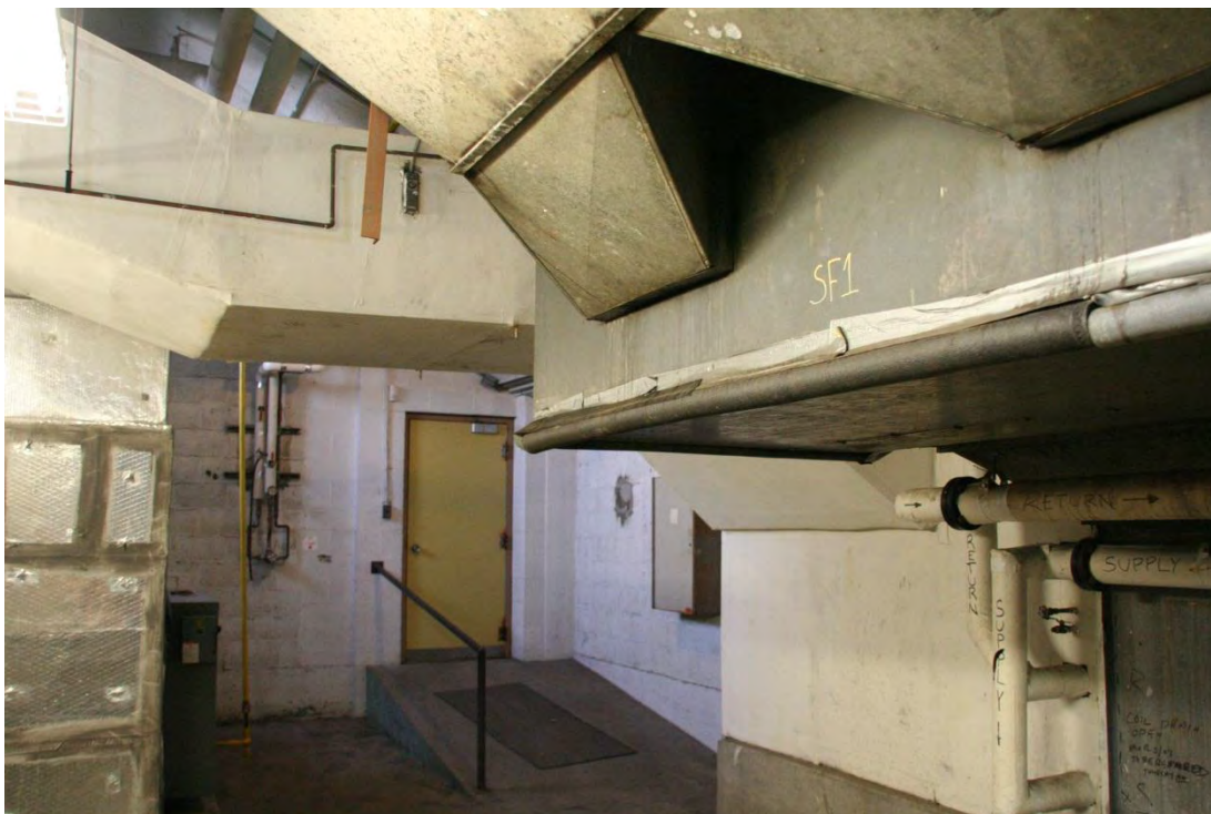
Figure 27: Filter room showing ramp down from ground floor. Air ducts at top of photo
