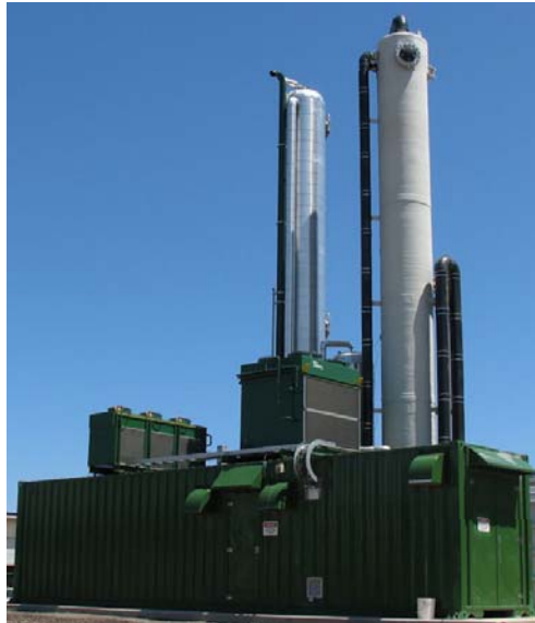
Biogas Enhancement Project Natural Gas Purification Warranty Period 2013
