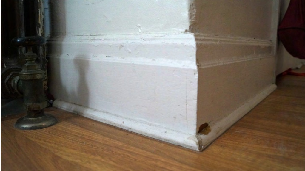
Fig. 233 Southeast bedroom's baseboard
