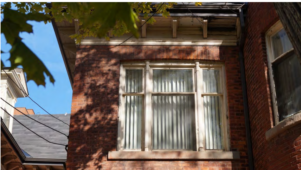
Fig. 41 Tripartite window at attic floor, somewhat shorter than the ground-floor tripartite window
