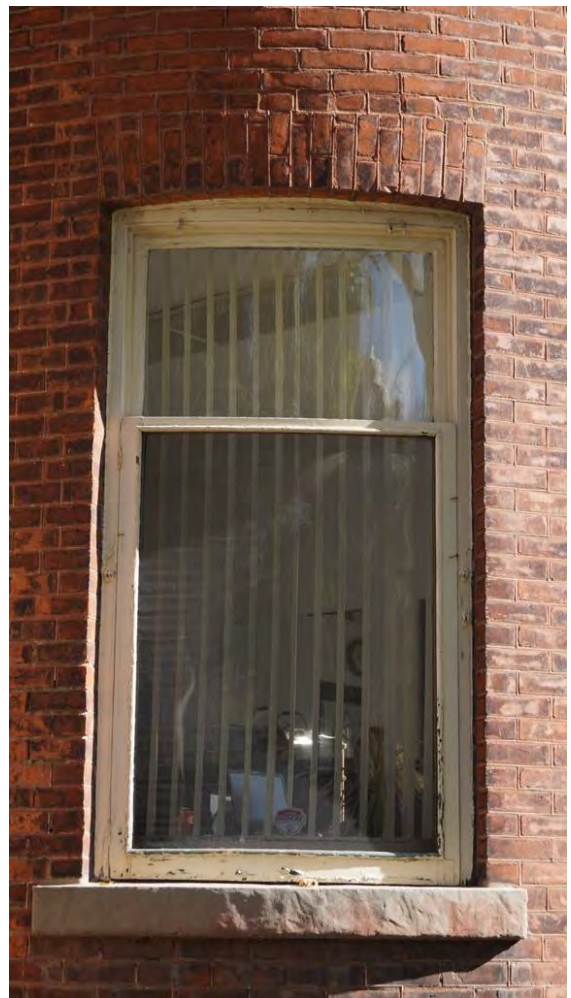
Fig. 37 Another ground-floor window in turreted bay – this one covered by a storm window
