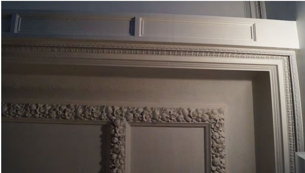
Fig. 182 Connecting room's plaster ceiling panelled with a design of flowers and fruit
