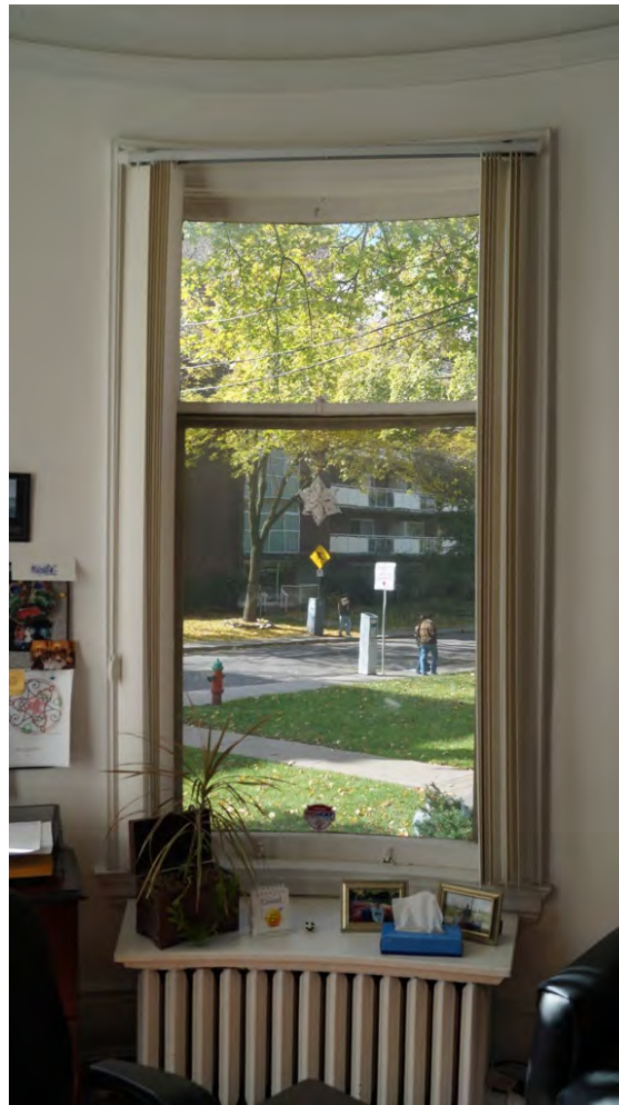
Fig. 75 Curving parlour window with cast-iron radiator below. Note window surrounds are partly hidden by vertical blinds.
