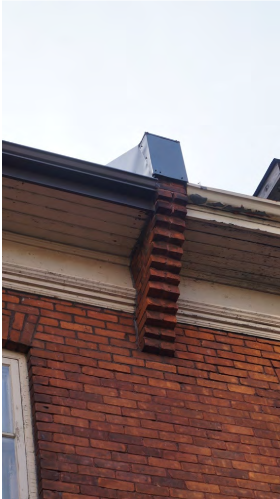
Fig. 154 Rear elevation's wood cornice, corbelled brick bracket and metal-flashed parapet for fire wall
