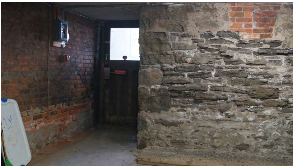
Fig. 64 Basement boiler room, showing brick partition wall, back entrance and limestone rubble stone foundation wall
