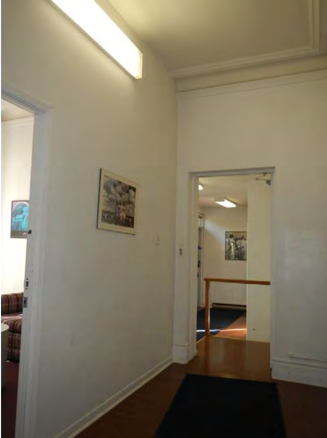
Fig. 66 Current configuration of entry hall, looking west to the link. Note the partition wall on the left is not original.
