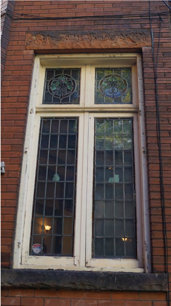
Fig. 146 One of the leaded and stained glass windows incorporated into the fireplace design inside
