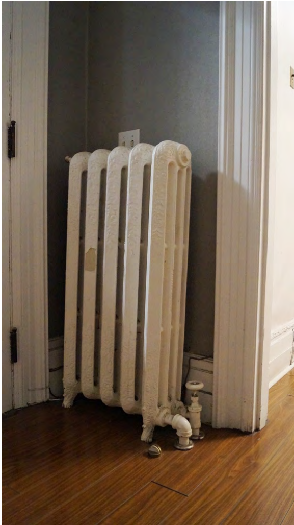
Fig. 166 Cast-iron radiator in front vestibule
