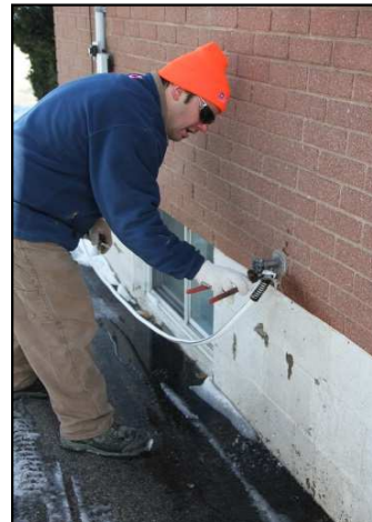
House to House Connection
