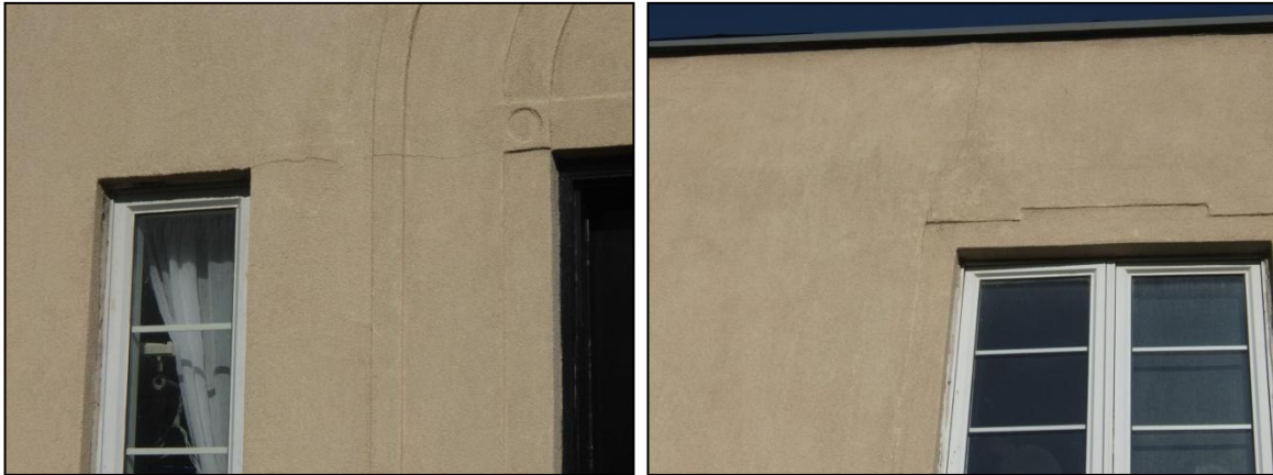
Typical cracking of exterior stucco finish (October 2015)
