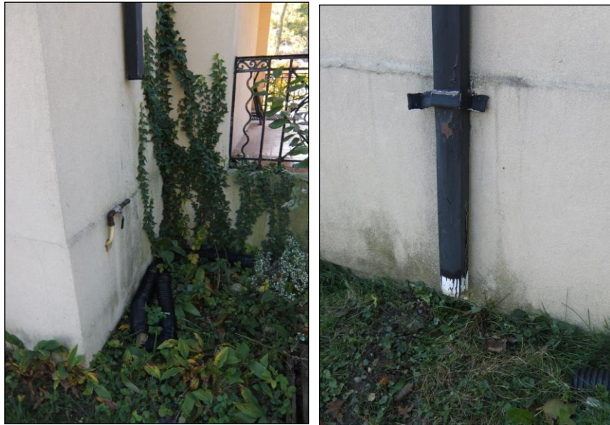
Disconnected downspouts in rear (north) and west (side) walls (October 2015)
