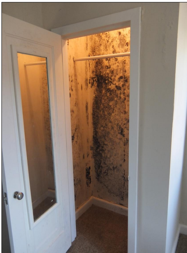
Mould growth in second storey, north bedroom, west closet (October 2015)
