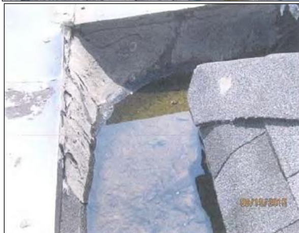
Typical roof system showing raised parapet wall, sunken gutters, flashing and clogged scrubbers (Source: Structure Report)
