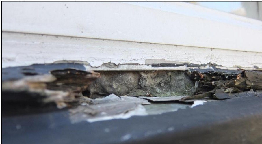
Deterioration of rear window frame (October 2015)
