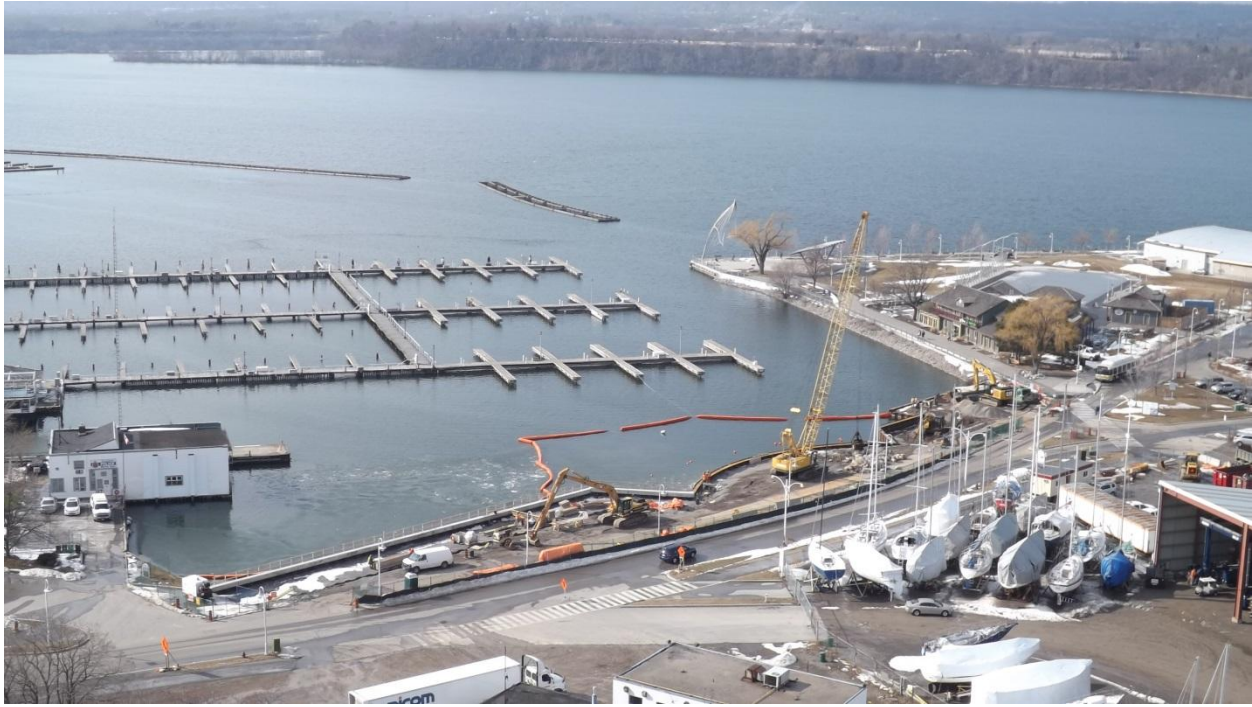
Below: New shoreline construction has eliminated mature trees.
