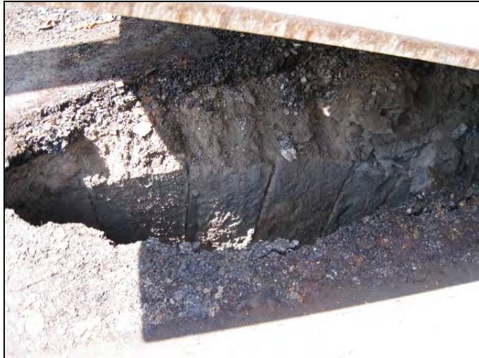
The historic barrel vault under Tecumseh Street in Hamilton is partially exposed for inspection by temporarily raising the overlying protective steel plate in the roadway. This landscape feature was built for Sir Allan MacNab on his Dundurn Castle estate before 1848,
