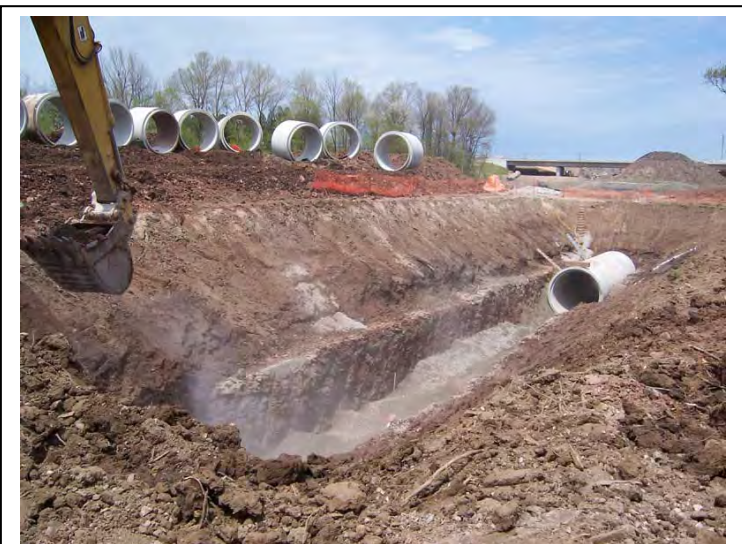
Extensive capital projects such as this combined sewer overflow pipe installed in the area of the Red Hill Valley Parkway Project result in large-scale soil disturbance and are subject to archaeological assessment.
