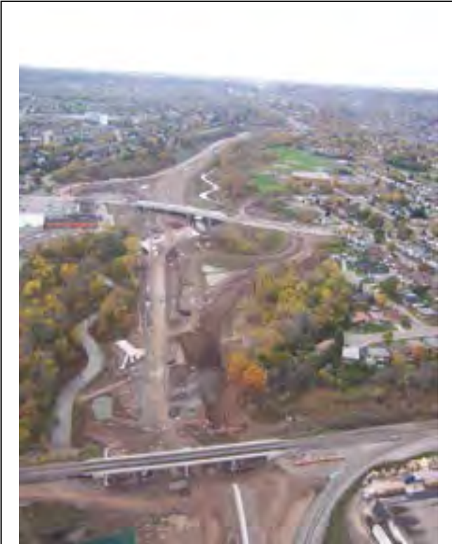
Construction of the Red Hill Valley Parkway through the Red Hill Valley corridor has required extensive grading and soil displacement. Archaeological assessment carried out through the project resulted in the archaeological excavation of several significant Native and EuroCanadian archaeological sites.
