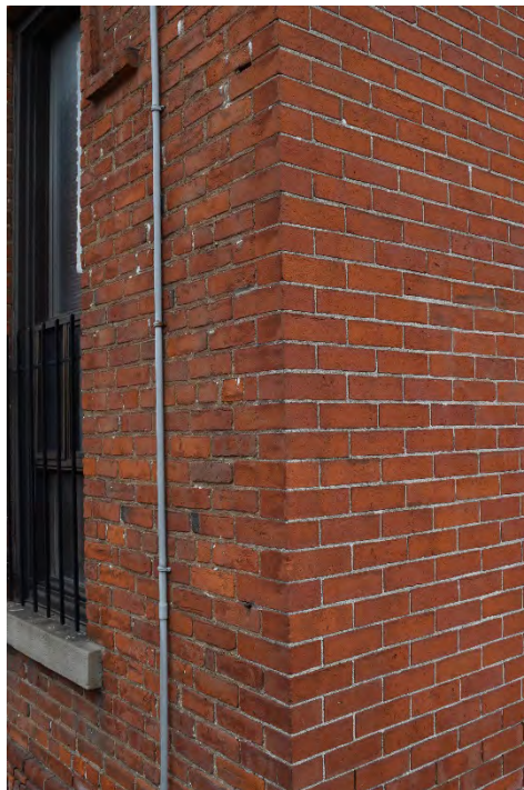
Figure 27: The southeast corner of the Parsonage showing the difference in brick bonding between the east façade (right) and south façade (left).
