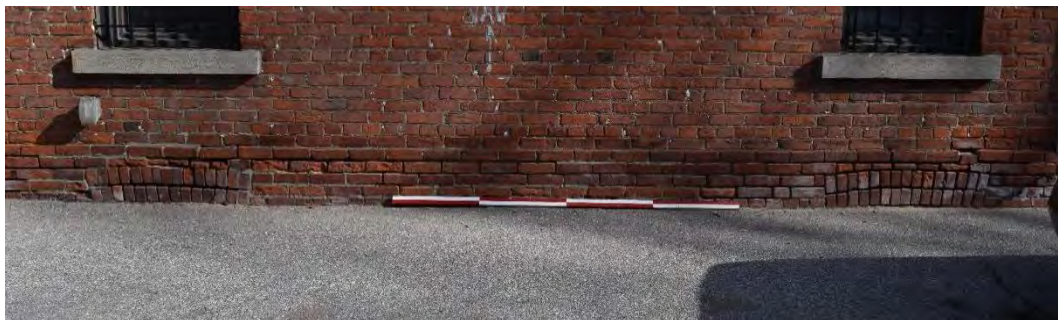
Figure 37: The two brick arches seen in the plinth of the south end wall. .
