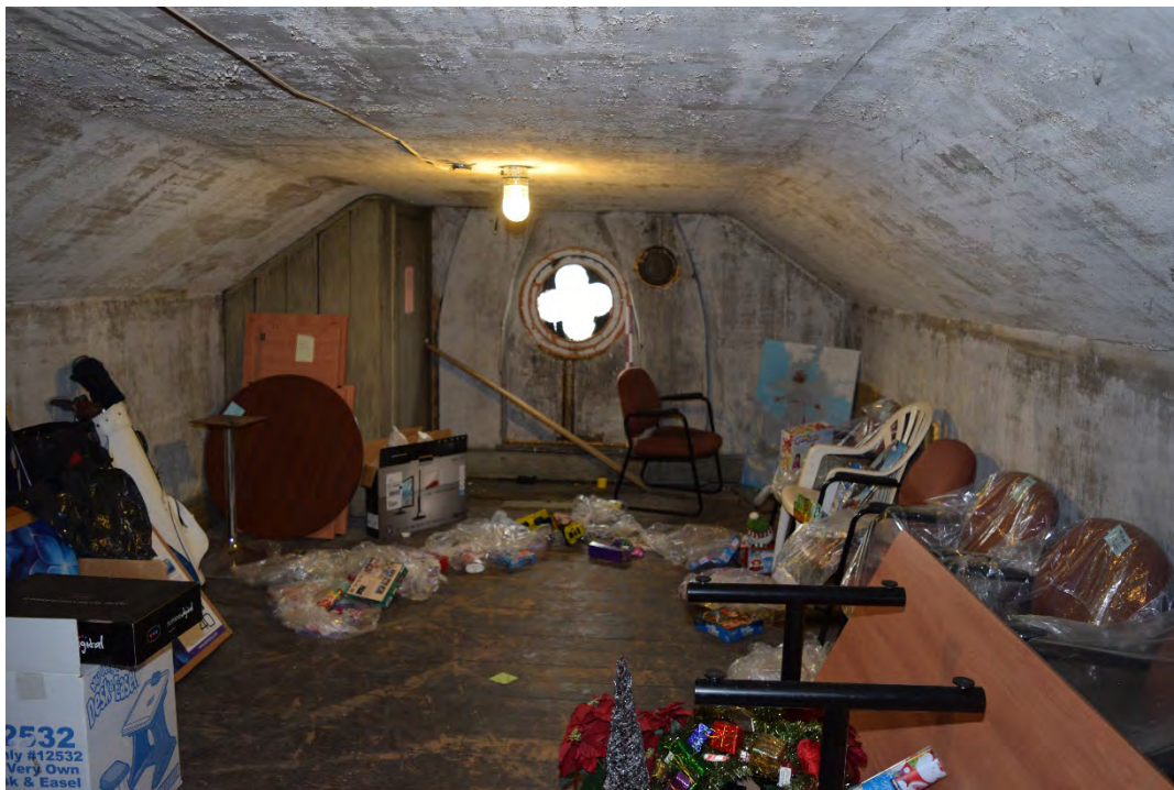
Figure 51: View of the south wing attic showing the quatrefoil window and flues.
