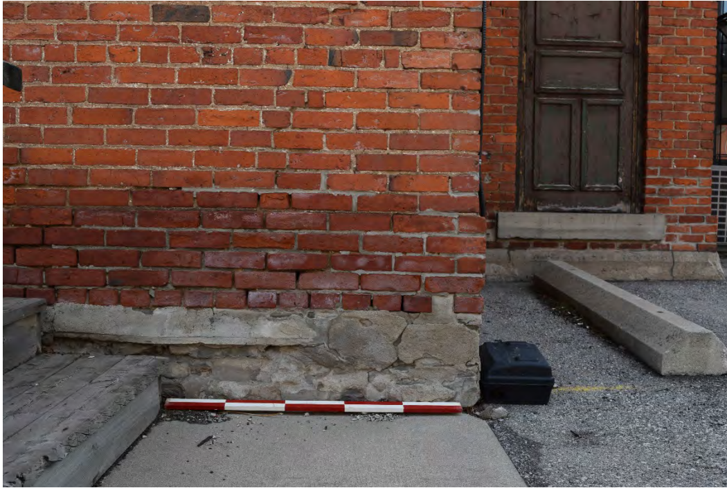
Figure 28: The brick plinth and parging over the squared stone foundation at the southwest corner of the north section.
