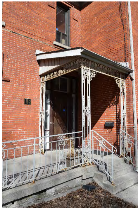
Figure 39: The east porch. Wood remnants of the earlier porch can be seen in the masonry above the present shed roof.
