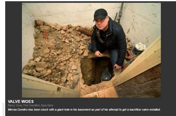
Backwater valve customer left with hole in basement
