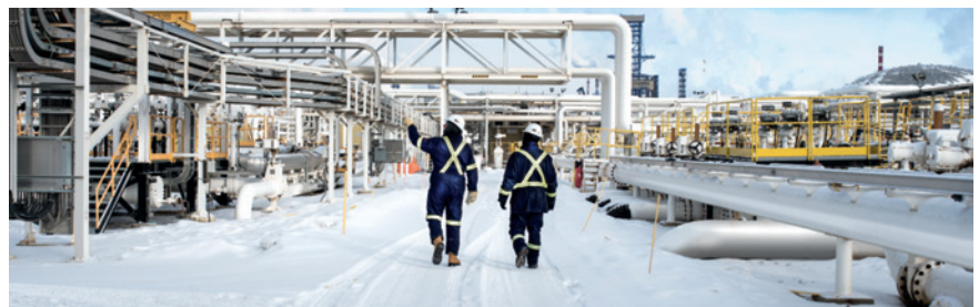
Variable speed drive electric motors at pump stations help to reduce the emissions profile of Enbridge’s liquids pipelines business.
