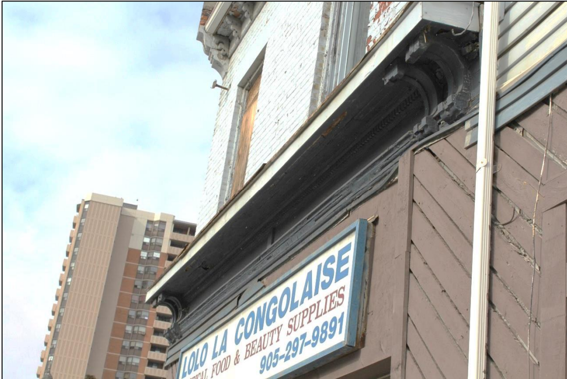
Photograph 5: View showing cornice and bracket details between ground floor and second storey (AECOM, 2017)
