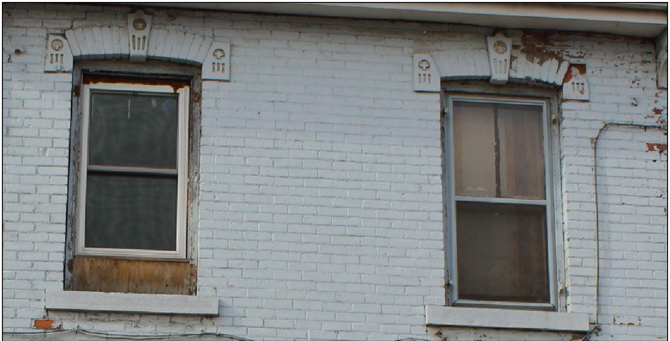
Photograph 8: View showing details brick segmental arch lintels, and concrete details on rear portion of 563 building, formerly 3 Steven Street (AECOM, 2017)
