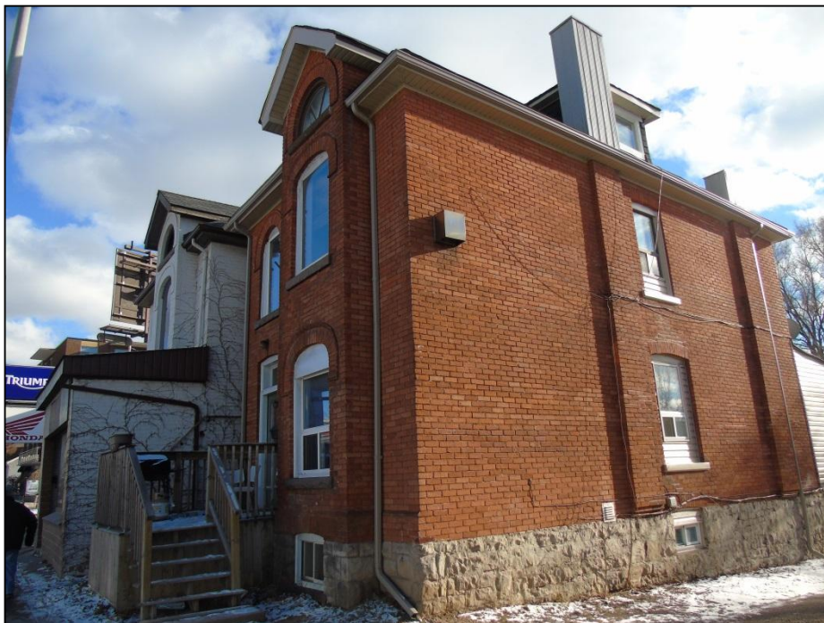
Photograph 4: View showing west facade of 621 King Street West, showing rubble stone foundation and smooth exterior brick
