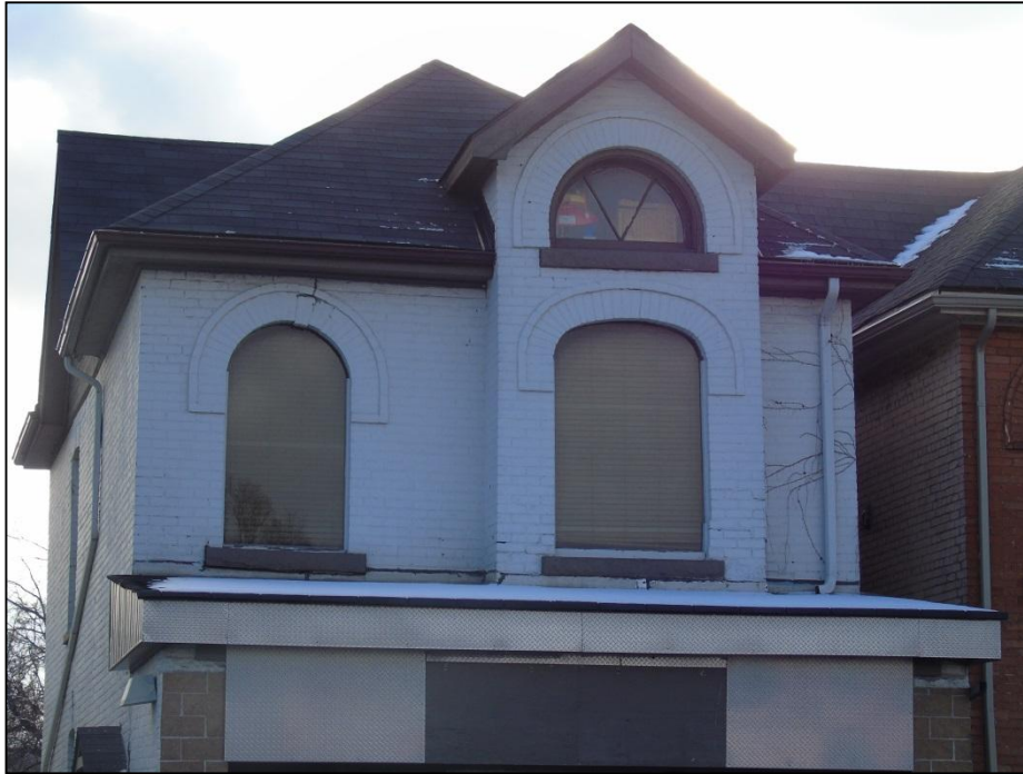
Photograph 5: Second storey details including arched brick lintels, concrete sills, and round-headed attic window
