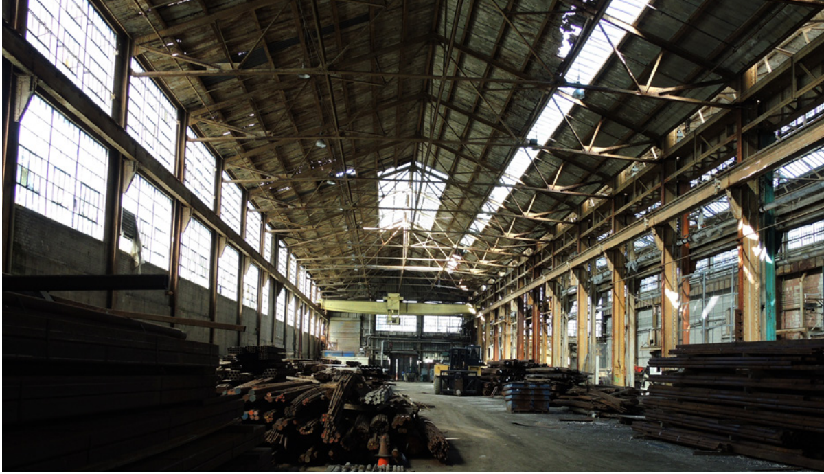
Above: Westernmost production shed, looking north. Note rows of flat skylights along pitched roof, extensive glazing along exterior wall, and overhead travelling crane at the shed's north end, 2016 (ERA Architects).
